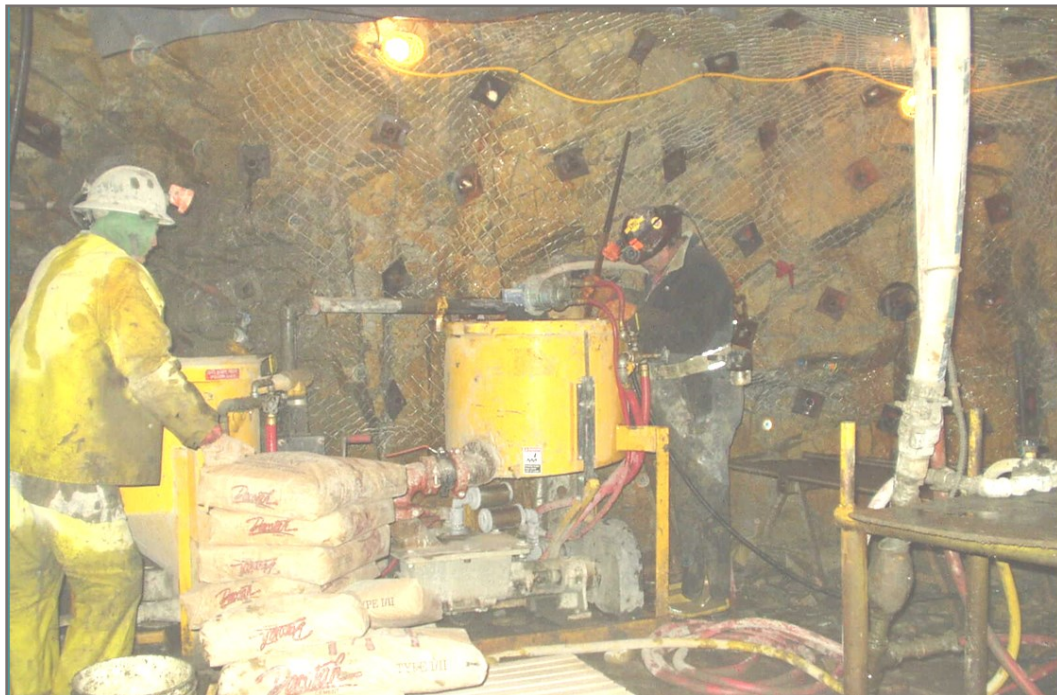
Photo 4: Installation of grout rings All walls and roof should be cleaned and washed free of dust and debris. Grouting rings are installed around the hydraulic plugs and proposed bulk head location.
