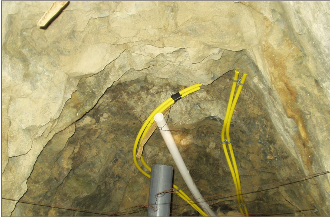
Photo 3: Intersected location of the workings is located and installation of grout and cement pumping lines.
