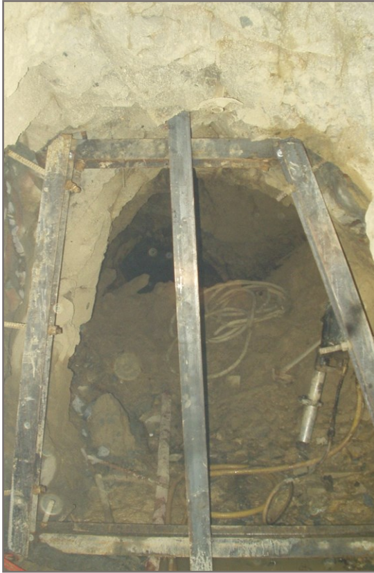
Photo 5: Building of the temporary bulk-heads. 6 Inch Steel High beams installed in preparation for lower seal.
