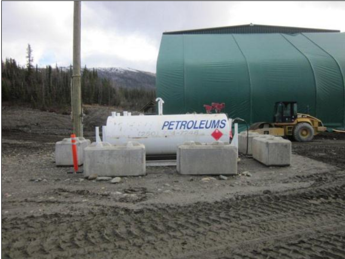
Plate 6-17: Diesel Storage Tanks
