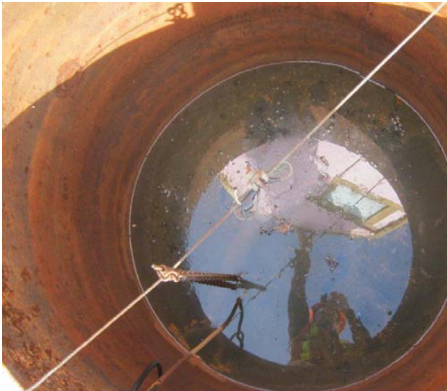
FIGURE 3 – BIOREACTOR INFLUENT SUMP
