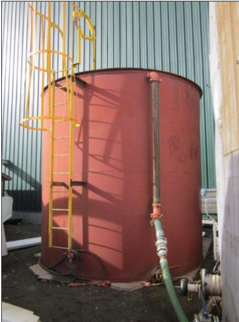
Plate 6-16: Fresh Water Tank
