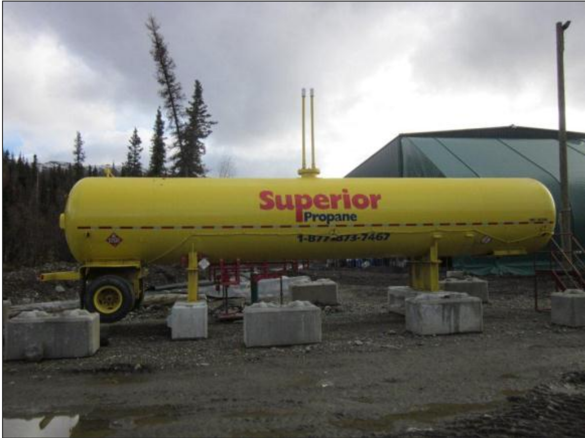
Plate 6-18: Propane Storage Tank
