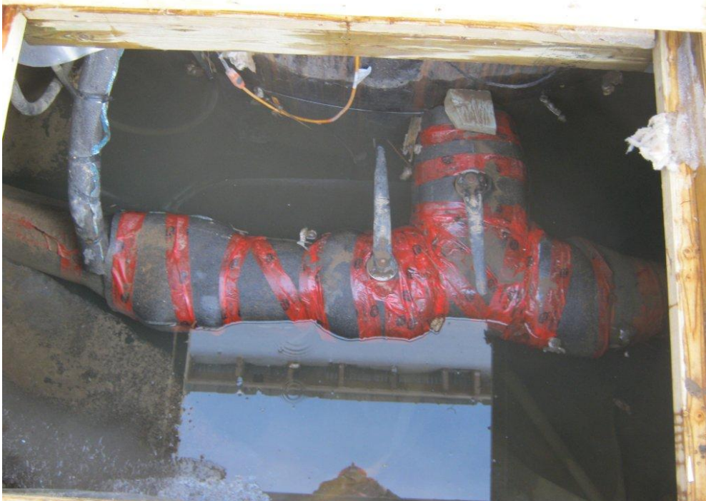
FIGURE 8 – BIOREACTOR DISCHARGE VALVES
