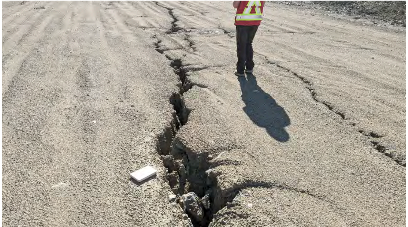
Photo 6-3: Longitudinal cracking along the crest of the SWD first observed in 2019.
