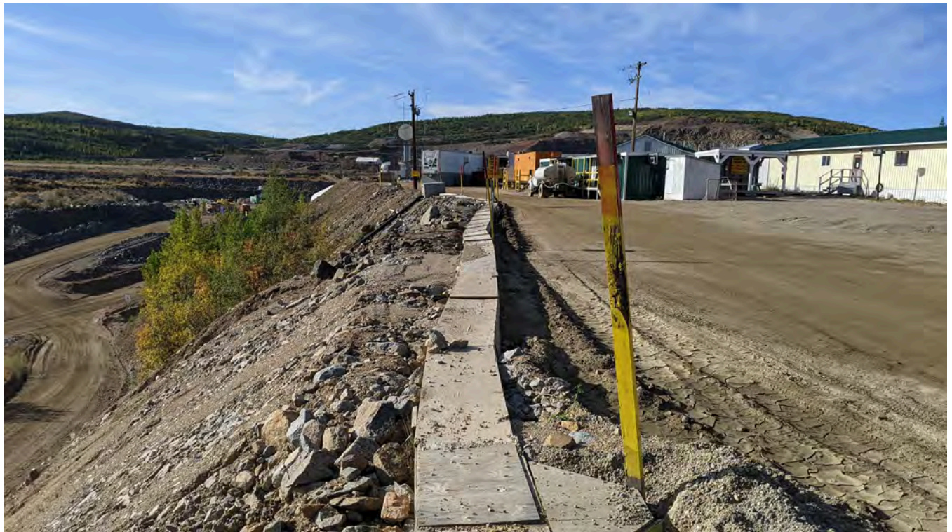
Photo 10-3: Repaired erosion gully noted in the 2020 inspection at the north end of camp. (looking south).
