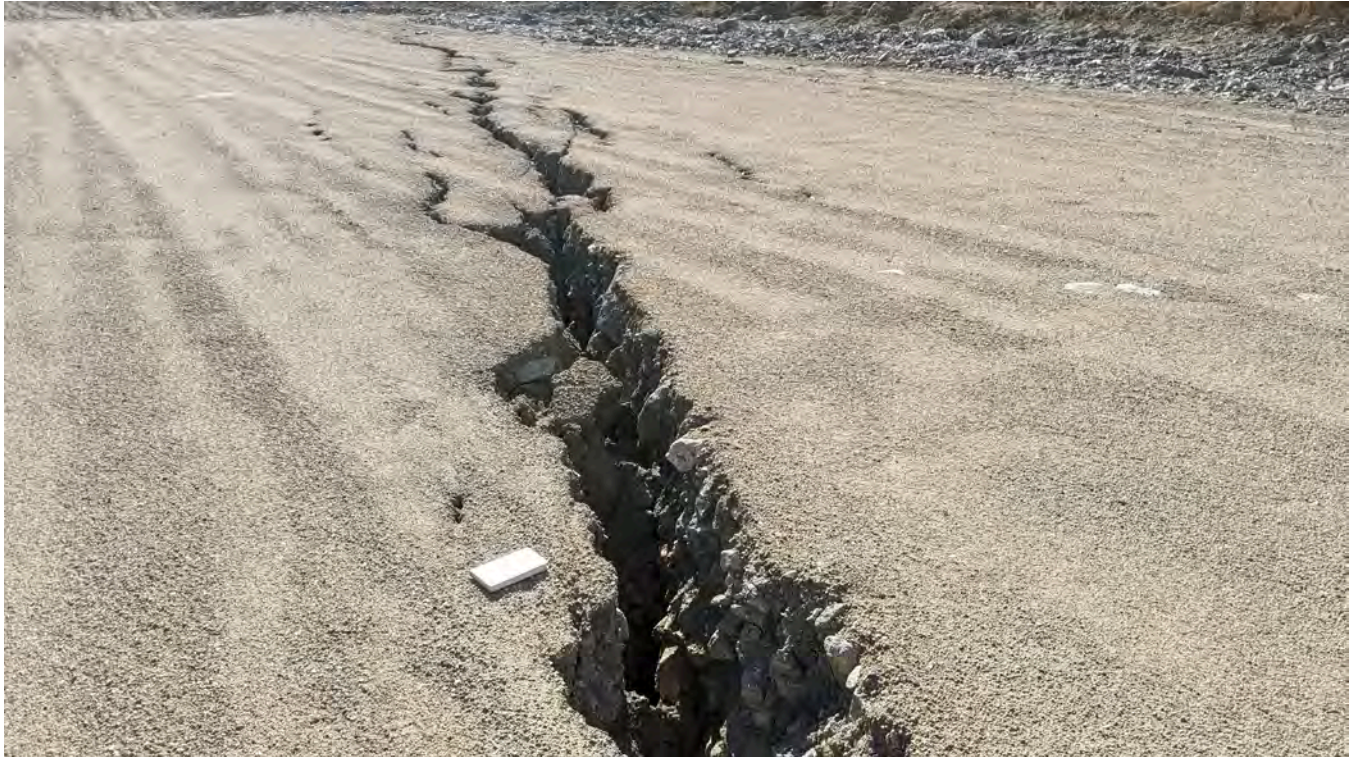
Photo 6-5: Longitudinal cracking along the crest of the SWD first observed in 2019 at its widest point.
