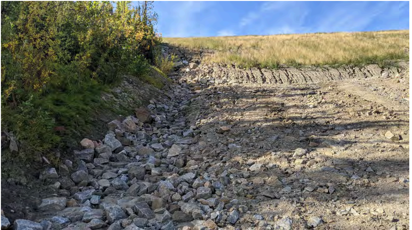
Photo 2-6: The road down to the MVFE Sump has been upgraded with a armored drainage channel constructed on the south side of the road to prevent sediment transport to the MVFE Sump area.
