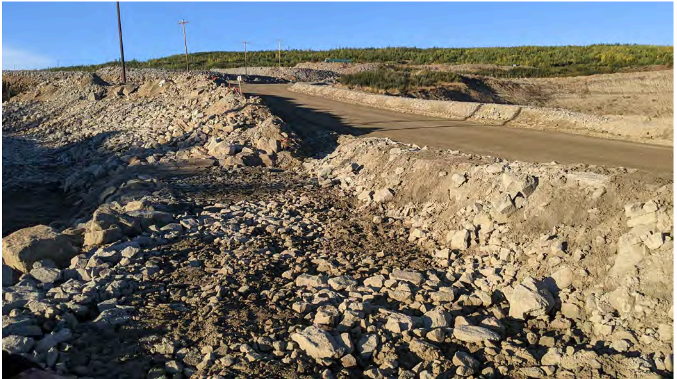
Photo 3-2: TDD Intake Channel. View of the location where the Underground Access Road runoff enters the TDD area. The overflow spillway is non functional. Flows that exceed the TDD intake will continue down the Underground access road. Most of this flow would be directed west of the DSTSF.
