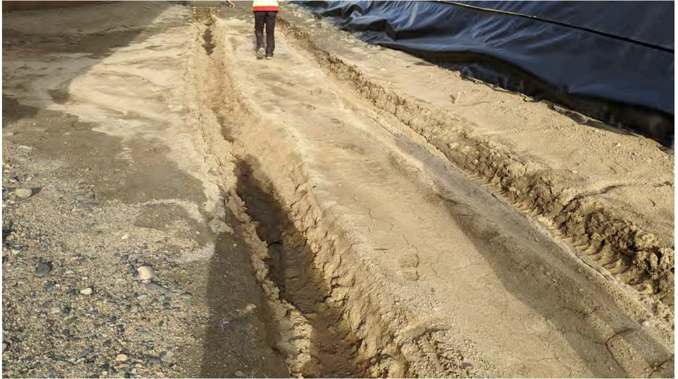
Photo 11-3: Tire ruts between the ramp and sump has exposed the base geotextile and liner in areas.
