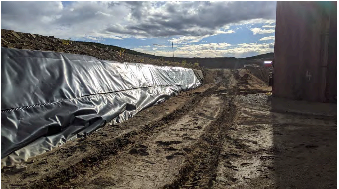
Photo 11-6: View of the ruts and liner along the side wall of the facility.
