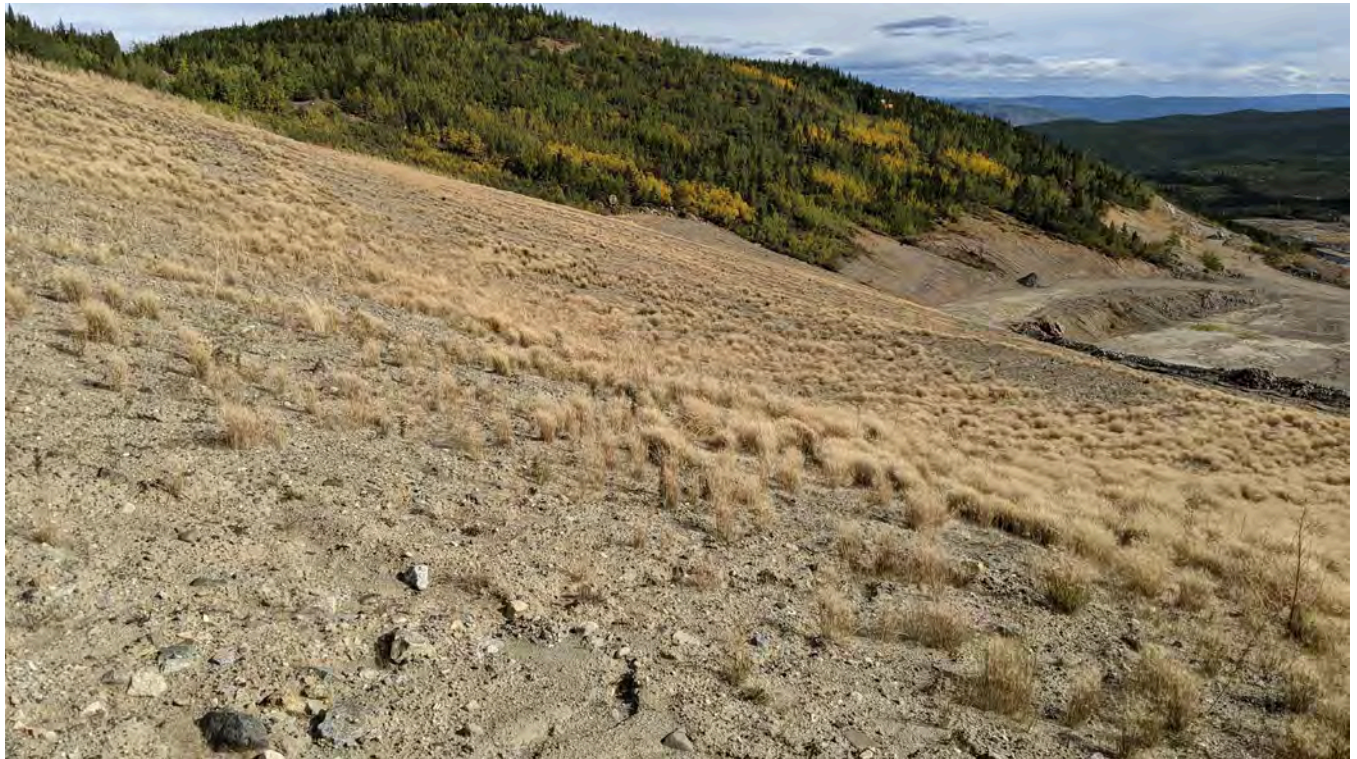
Photo 4-2: MWD regraded slope (looking northeast). Photo is in the location of the cracking of the cover soil noted in the 2019 inspection. The crack was not observed in the 2020 or 2021 inspection. The cover surface in this area has a concave slope.
