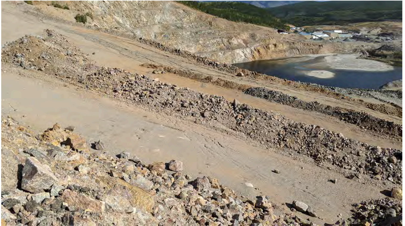
Photo 5-1: Cracking on the crest of the lower bench of the MWD Wrap.
