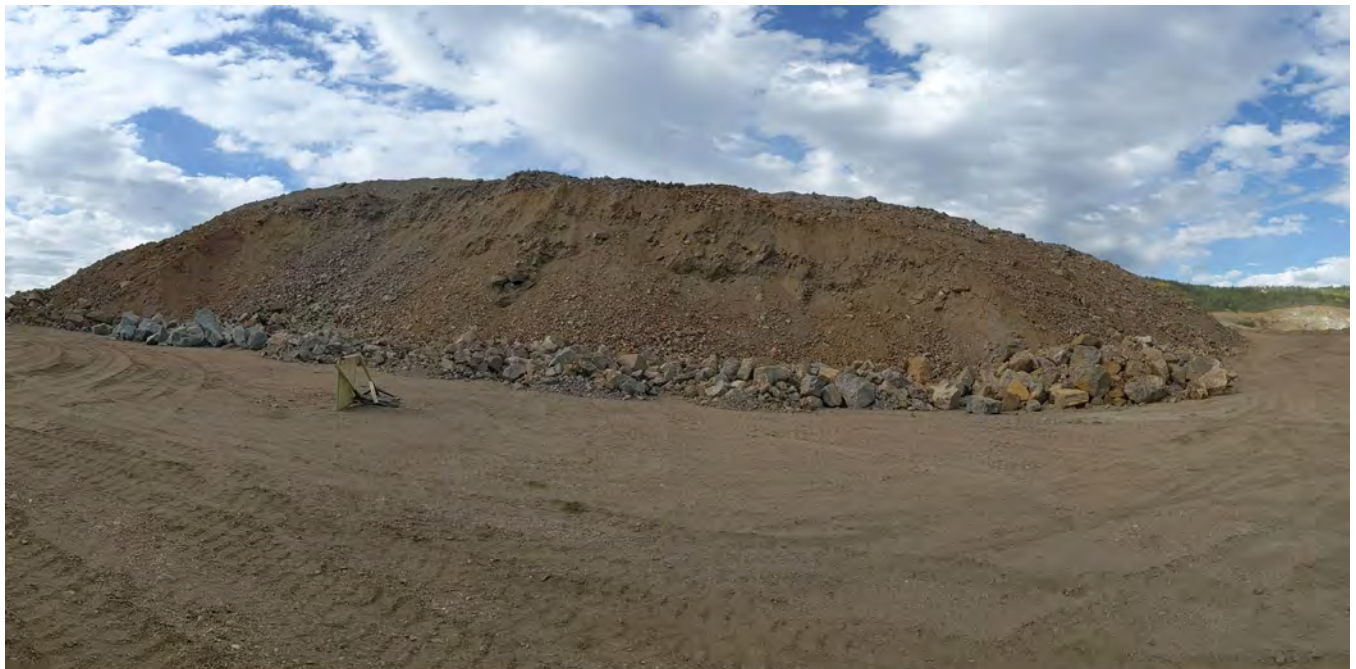
Photo 5-2: Waste Rock excavated from the toe of the MWD Wrap (looking north) that has resulted in an over-steepened slope.
