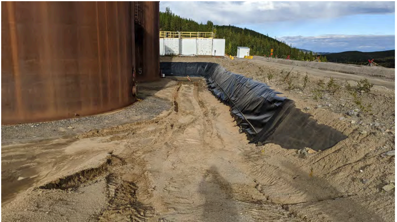
Photo 11-2: Entrance ramp to the facility with a new large rut near the edge and new rutting between the ramp and sump (far end).
