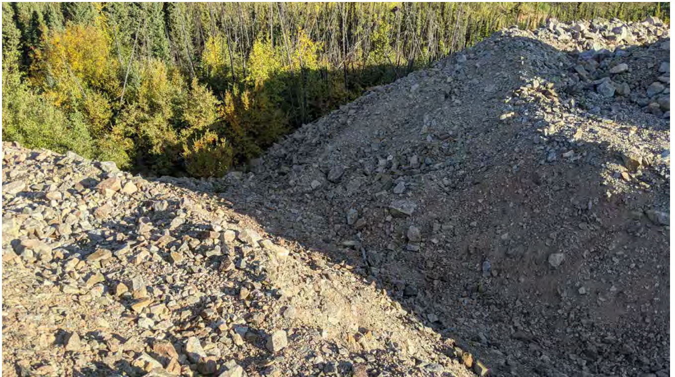
Photo 3-6: TDD Outlet. No flow was observed at the time of the inspection.
