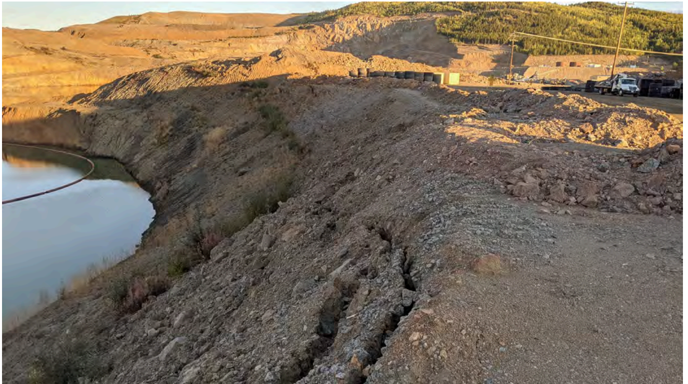
Photo 15-7: Cracking along the Area 2 Stage 3 Pit rim.
