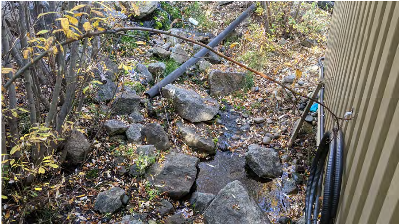
Photo 12-8: Seepage at the toe of the dam immediately upstream of the seepage collection sump. Seepage was clear with no signs of sediment transport.
