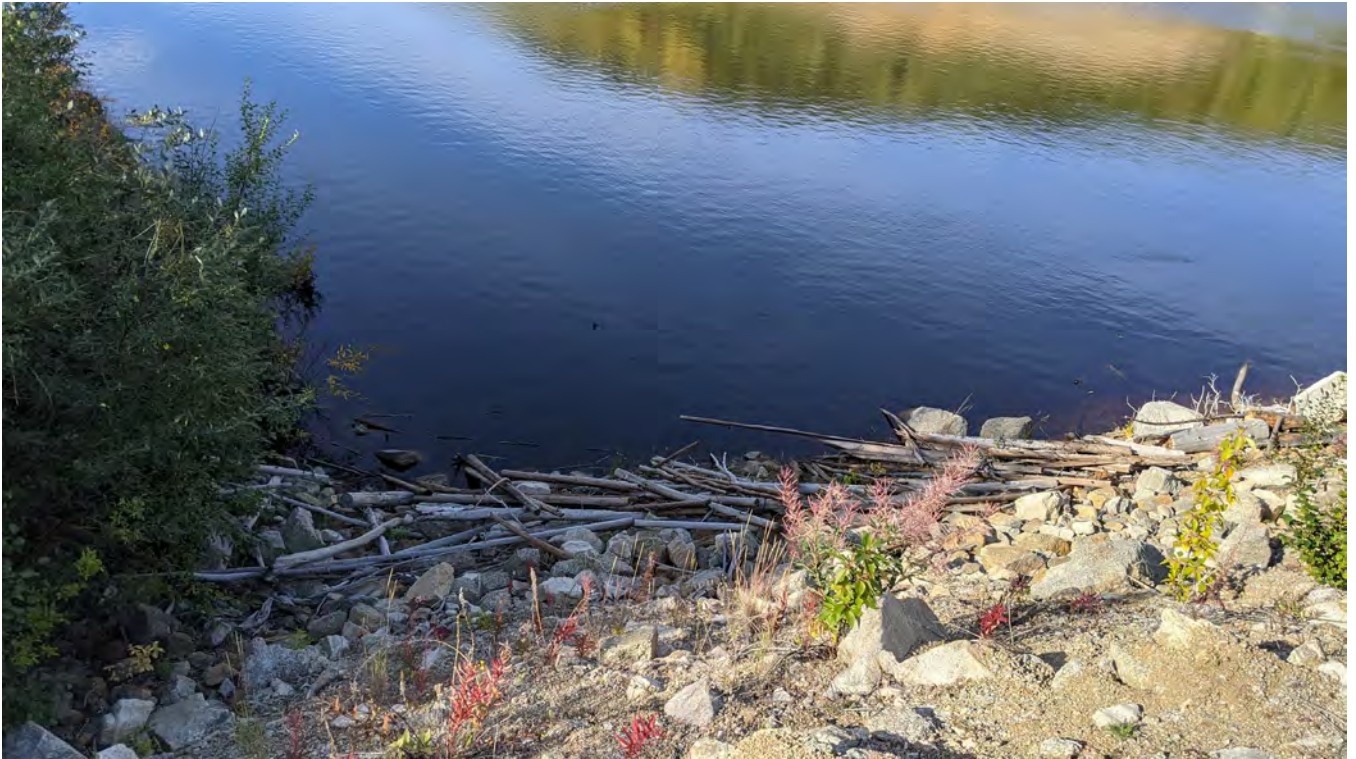
Photo 12-6: Accumulation of logs along the south abutment of the dam.
