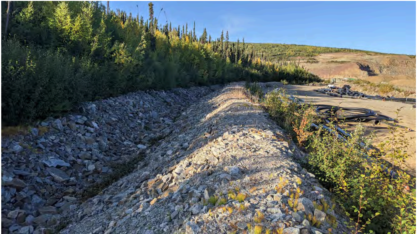
Photo 3-5: Typical view of the lower portion of the TDD with riprap. Sparse vegetation growing in the channel.
