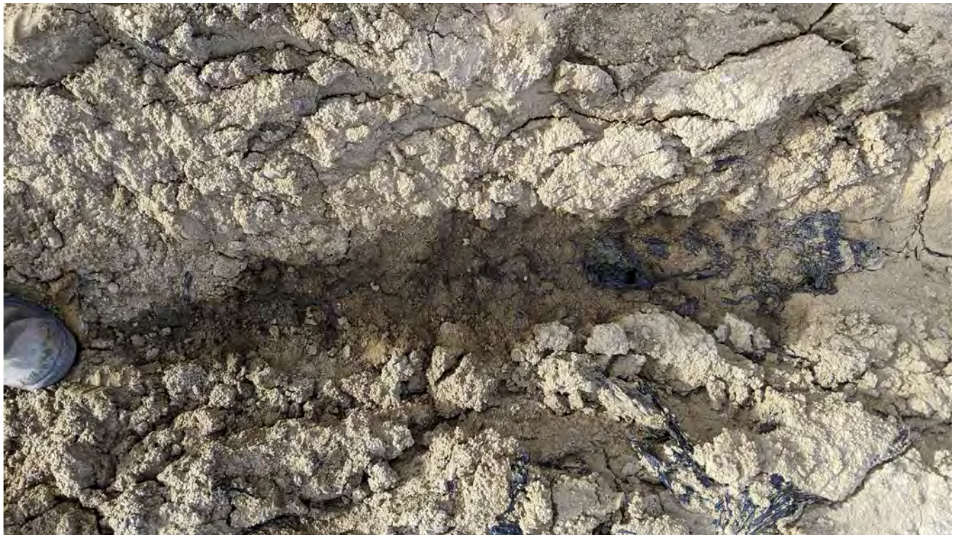
Photo 11-4: Exposed geosynthetics in the rut. A thin plastic is present overtop of the geotextile (that overtops the liner) that appears to be a sacrificial warning layer to prevent liner damage.
