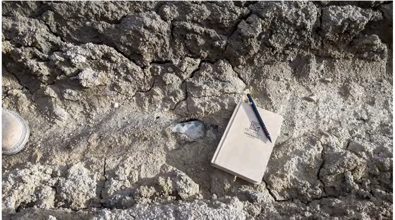
Photo 11-5: A small geotextile tear was found in the rut that is approximately 5cm x 8 cm. Liner damage could not be detected within the tear.
