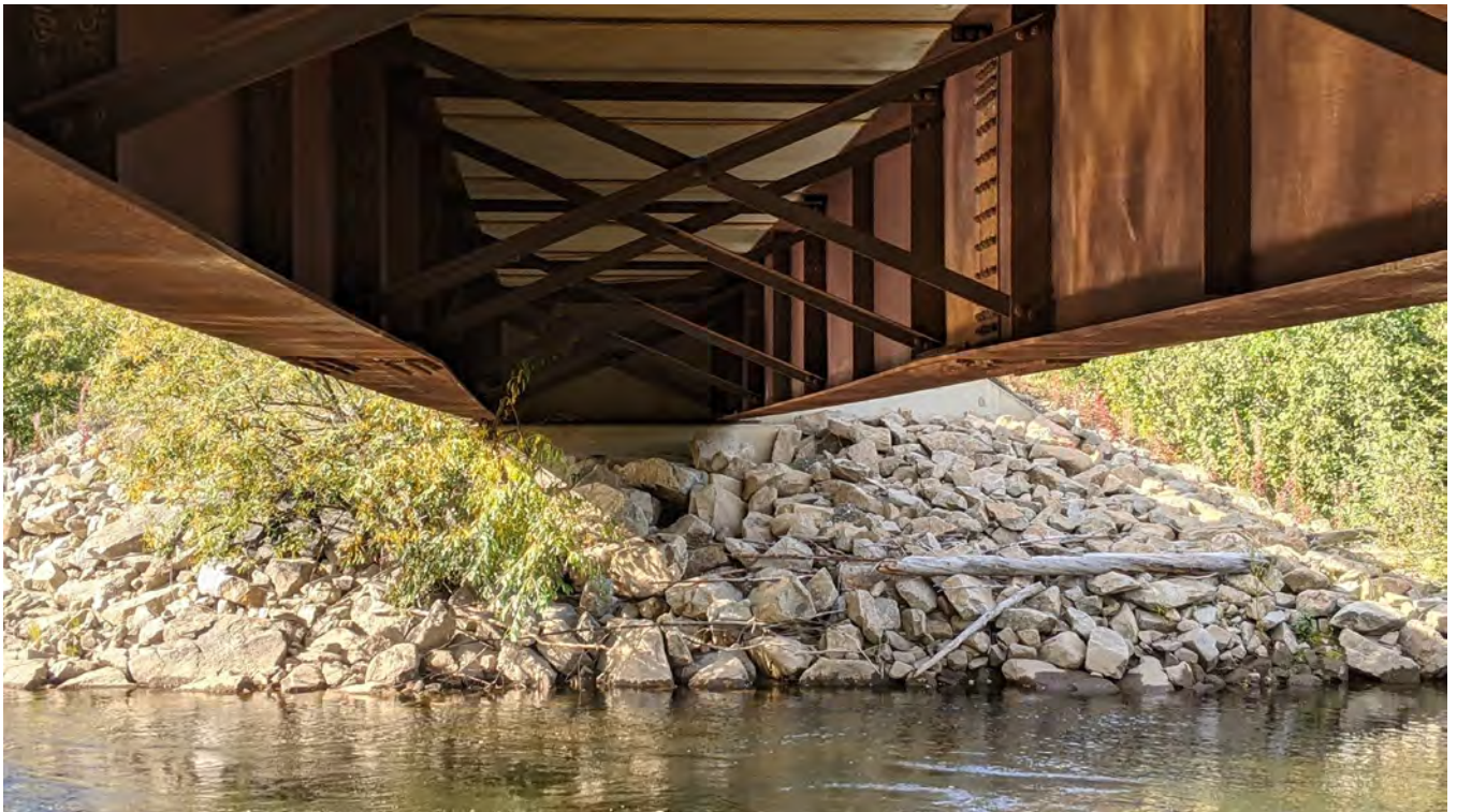
Photo 13-2: Western abutment. A Tree is growing on the upstream side of the western abutment.
