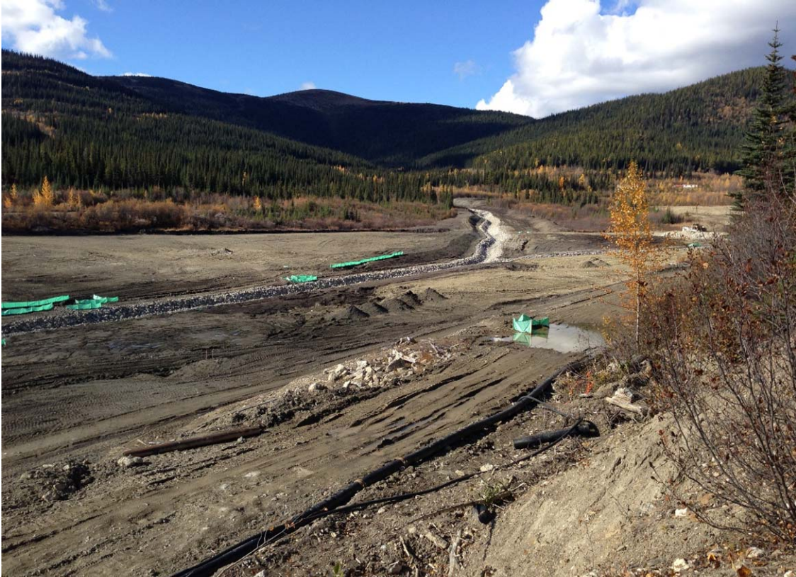
Photo 11: View looking west over the relocated Camp Creek in the riprapped channel.
