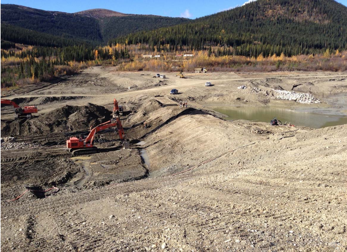
Photo 9: View looking west along the centerline of the removed South Dam. The SRS is seen in the middle of the photo with the filter fabric being placed in the new emergency spillway.
