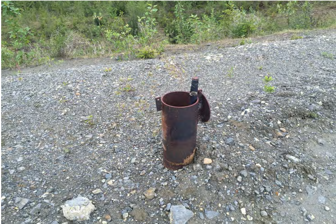
Photo 8: North Dam Settlement gauges
