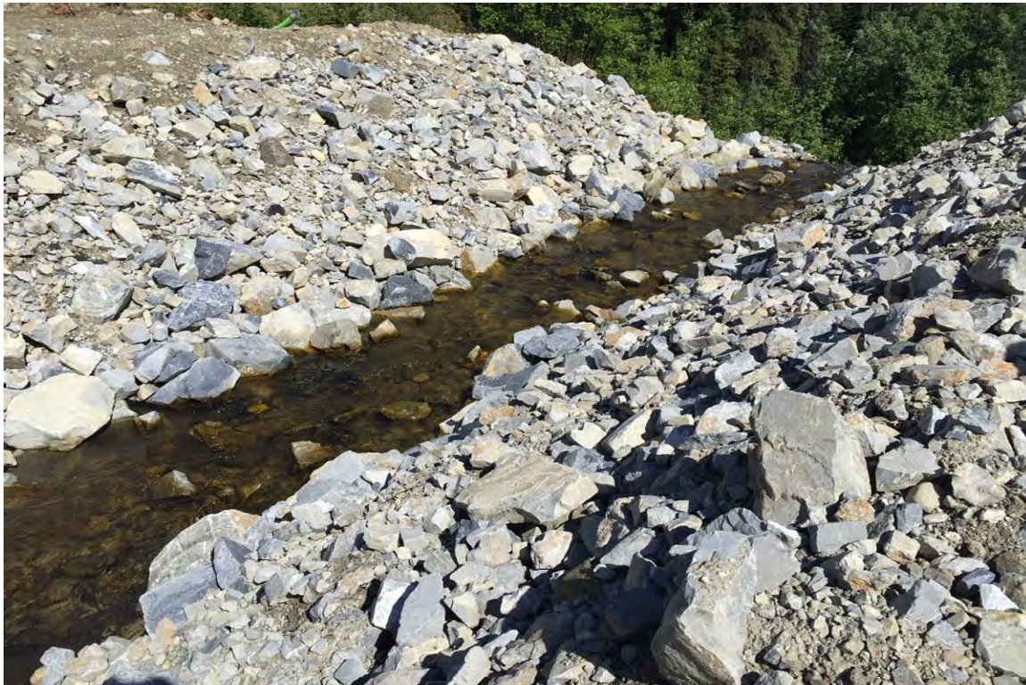
Photo 17: Channel through the North Creek Dyke following removal of the CMP culvert
