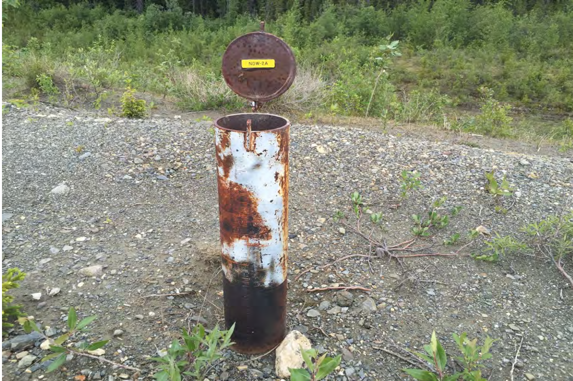
Photo 7: Protective steel casing for the Piezometers in the North Dam
