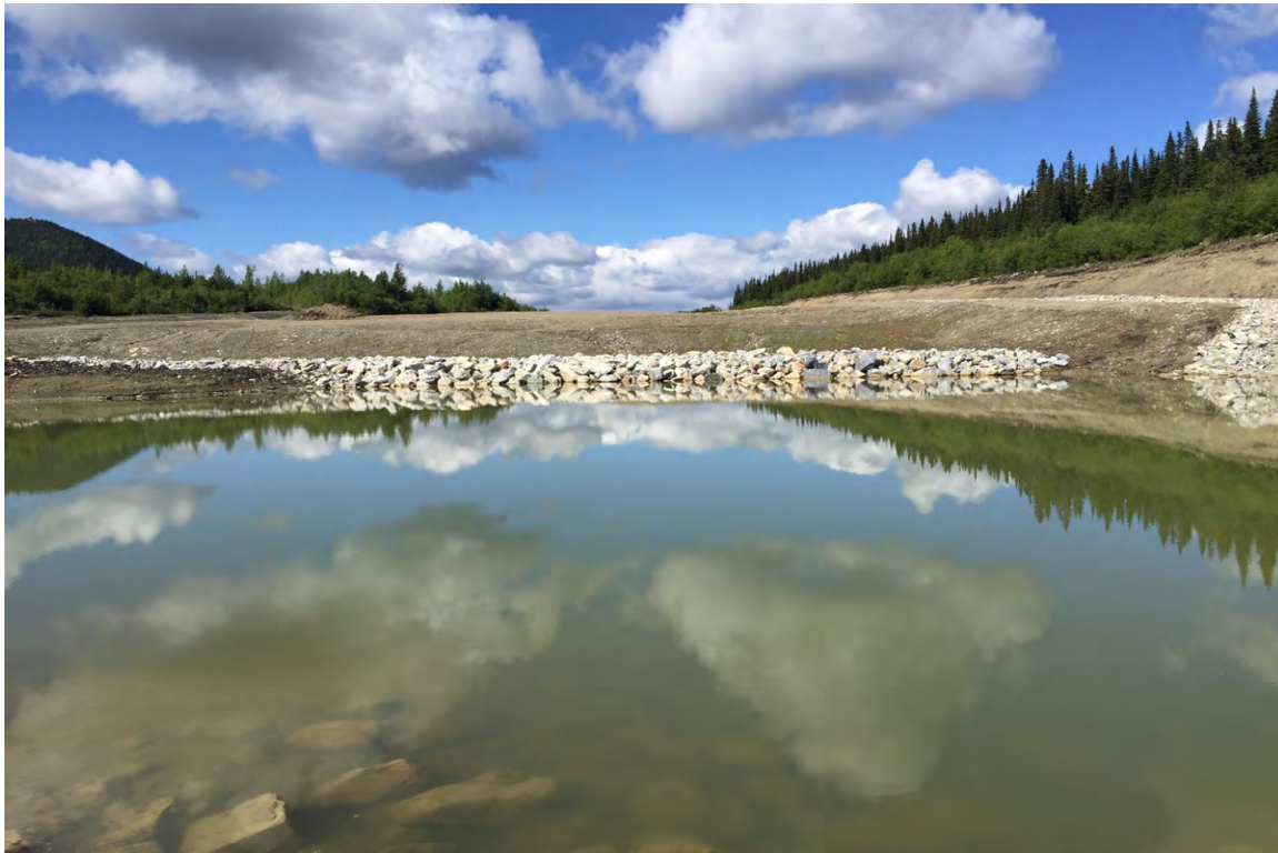
Photo 15: Sedimentation Pond at the SRS. North diversion channel is seen to the right of the photo.
