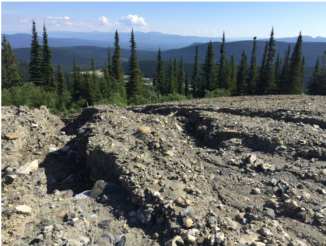
Photo 26: erosion gullies at toe of Jewelbox waste rock dump
