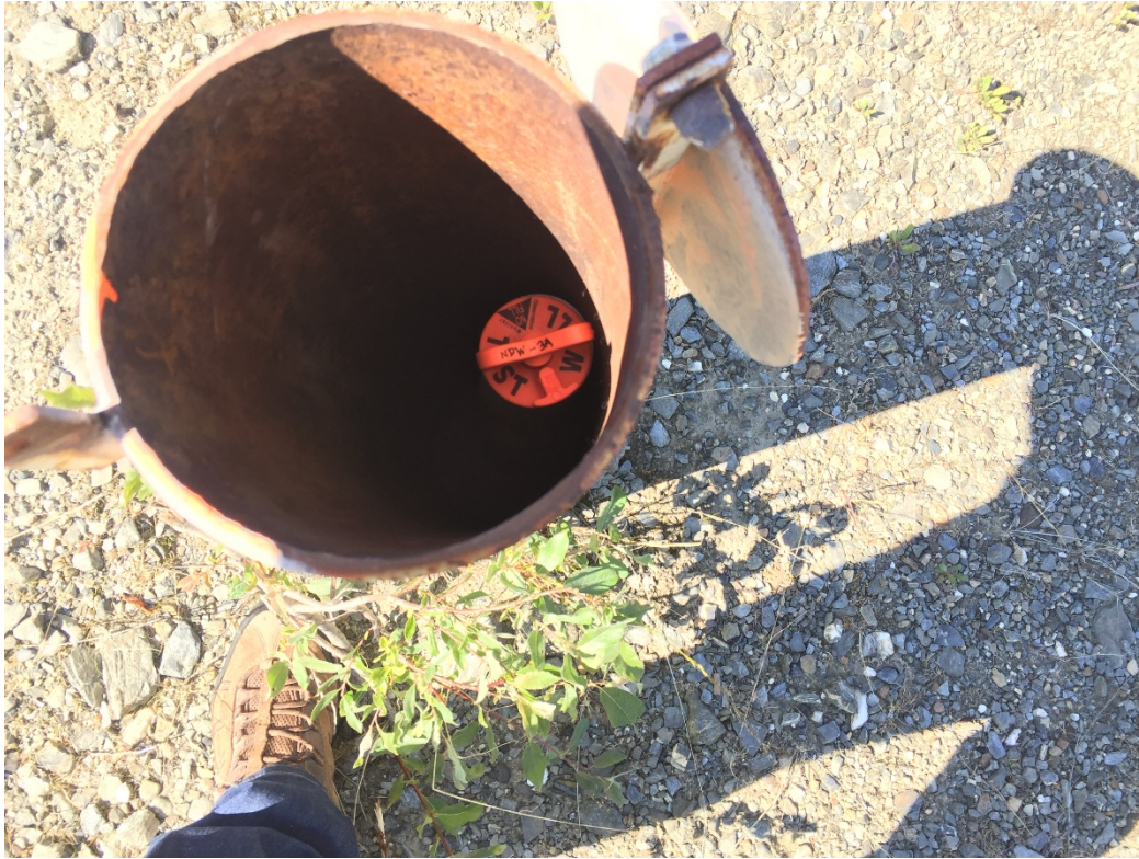
Photo 5: Plastic cap on the Piezometer NDW3A
