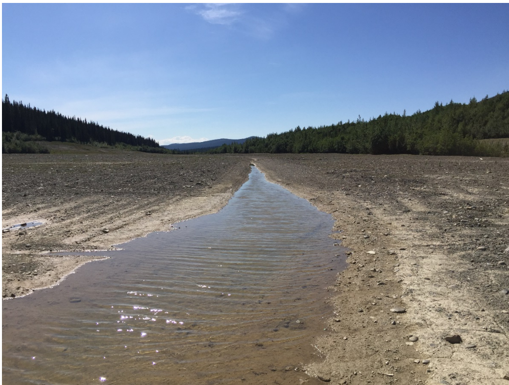
Photo 10: water in drainage swale draining south
