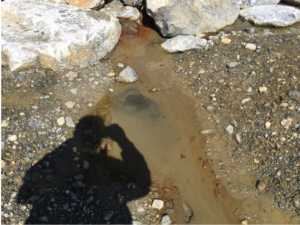
Photo 21: Single boil at toe of the SRS dyke
