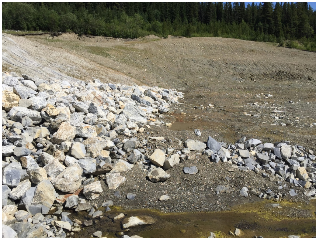
Photo 20: View looking east of the riprap buttress along the D/S toe of the SRS dyke
