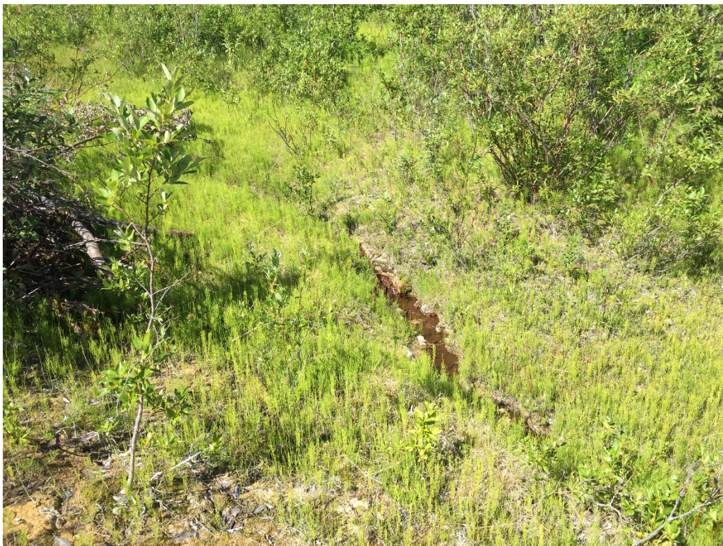
Photo 6: Hillside Seepage at toe of North Dam
