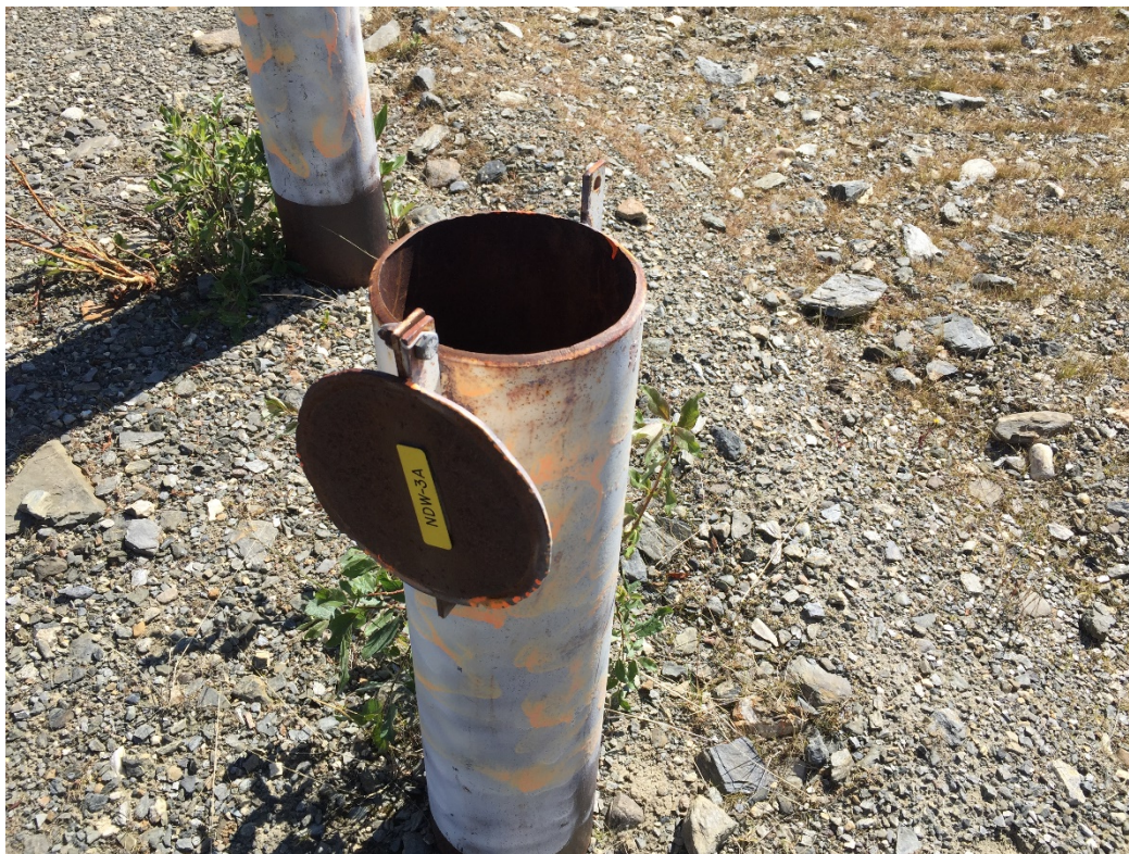
Photo 4: Well cover on NDW 3A
