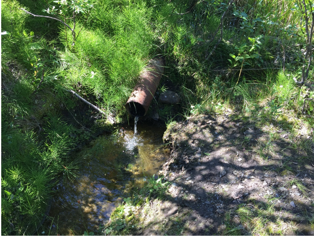
Photo 7: rotated pipe weir at MW 02
