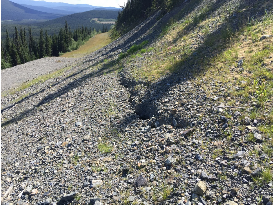
Photo 27 minor subsidence on the slope of the backfill at Portal 1200 on Burnick
