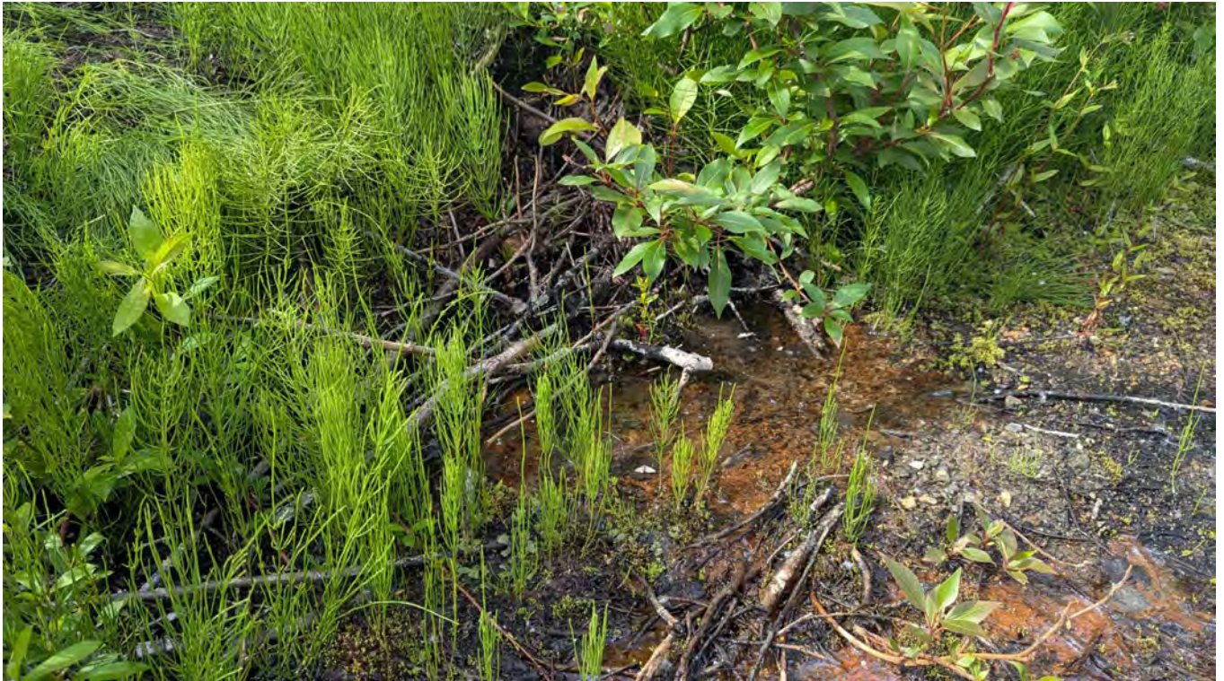
Photo NE-09: Seepage and soft ground observed at the embankment toe during the inspection 10 m west of the French Drain outlet.
