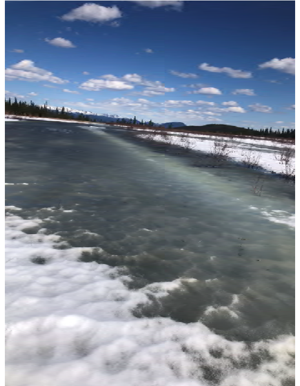
Photo C-2: Ponding/ice along the Main Drainage Channel looking north.
