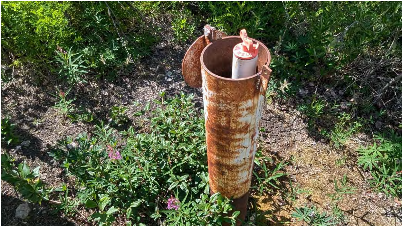
Photo NE-04: NDW-A4 Piezometer raised above the top of the protective casing due to frostjacking.
