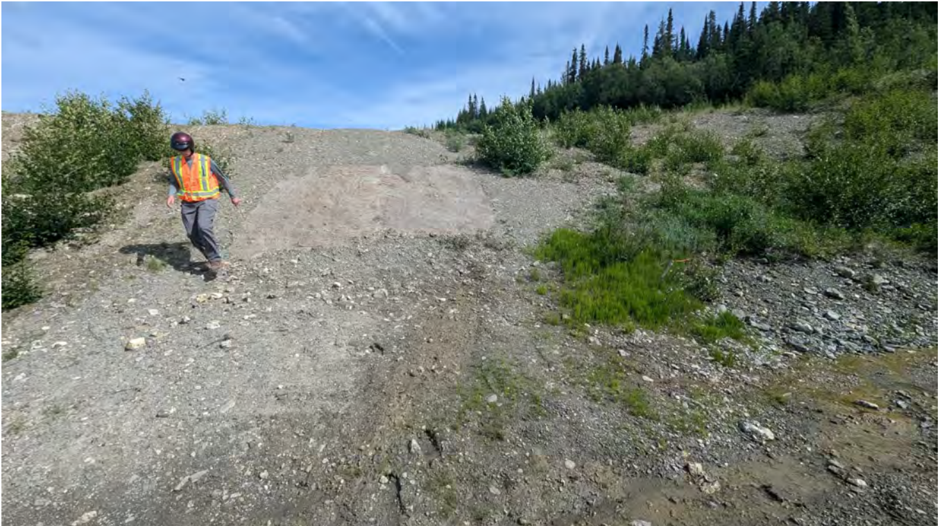
Photo SRS-05: Repaired sloughing area near the east abutment of the SRS. An erosion protection mat was installed on the slope as part of the repair.
