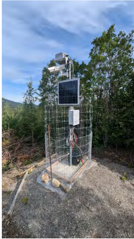
Photo NE-11: A remote-monitoring camera was installed east of the North Embankment to allow for real-time visual monitoring. Camera transmits via satellite.
