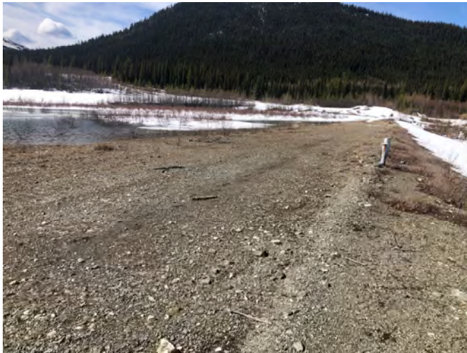
Photo C-3: Ponding adjacent to the North Embankment. Photo taken from near piezometer NDW-1A/B looking west..
