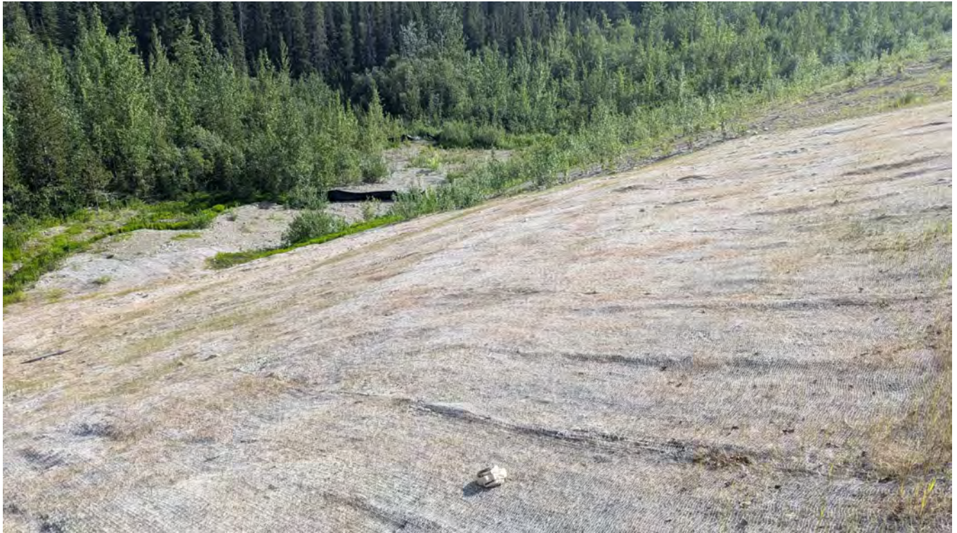
Photo NE-07: North Embankment gully repair erosion control blanket on the downstream slope.
