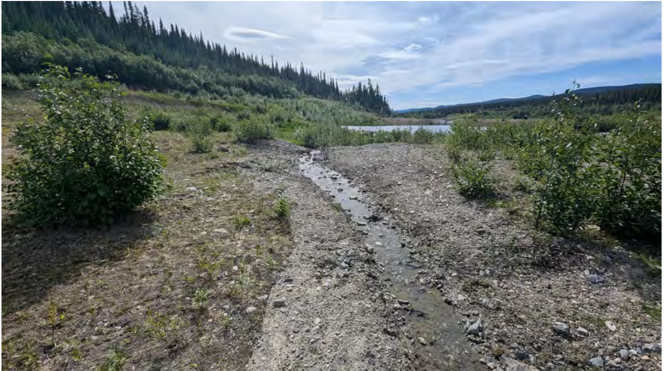
Photo TC-05: Repaired erosion area (repaired in August 2023). Looking downstream towards the SRS.
