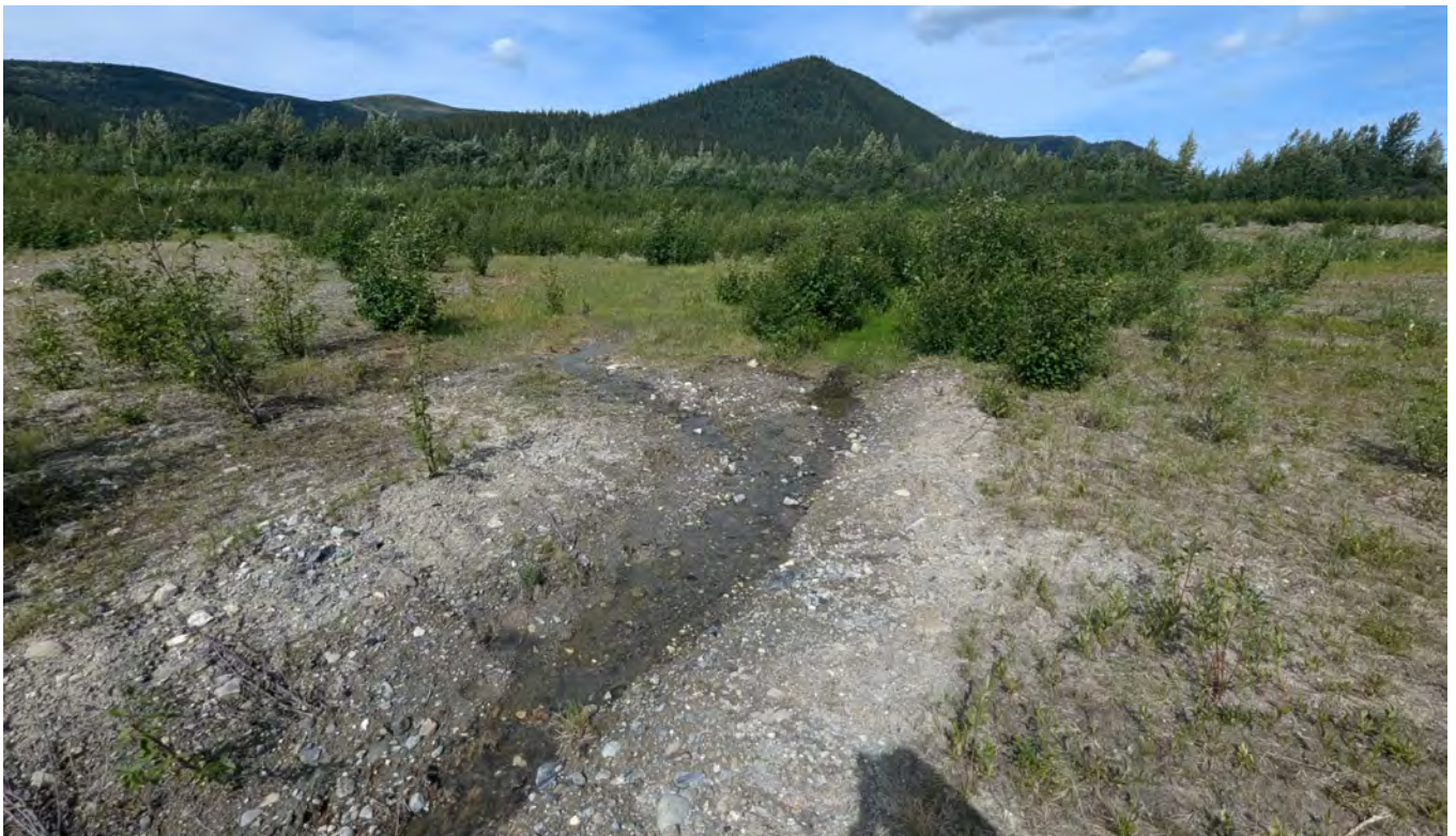
Photo TC-06: Repaired erosion area near the south end of the main tailings area (repaired in August 2023). Looking upstream to the northwest.
