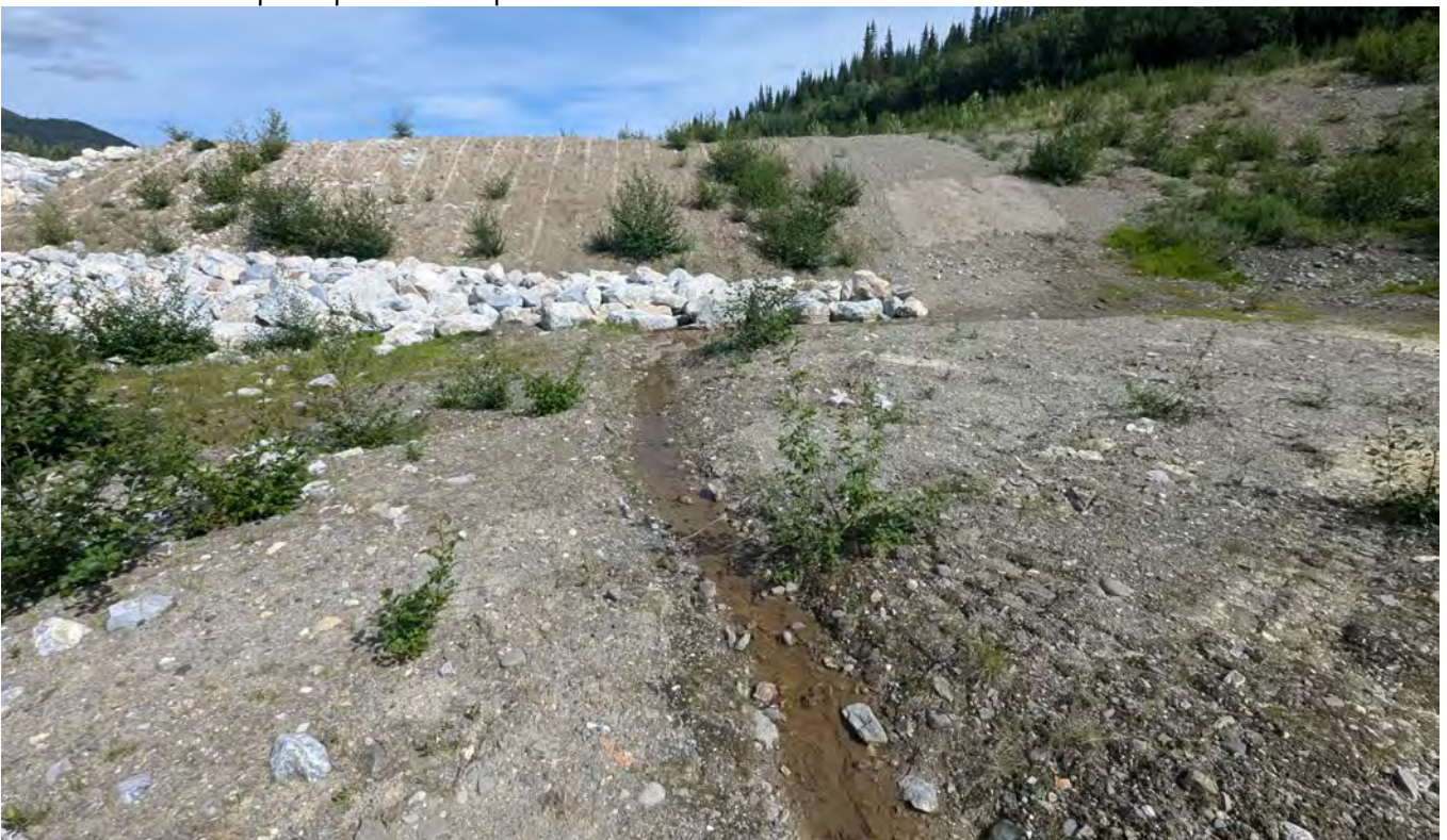
Photo SRS-06: Repaired slough area seen from downstream position. The area is away from the spillway and the ponded water area, and approximately 8 meters from the east abutment. Seepage is seen flowing from the SRS toe on the east side of the spillway.
