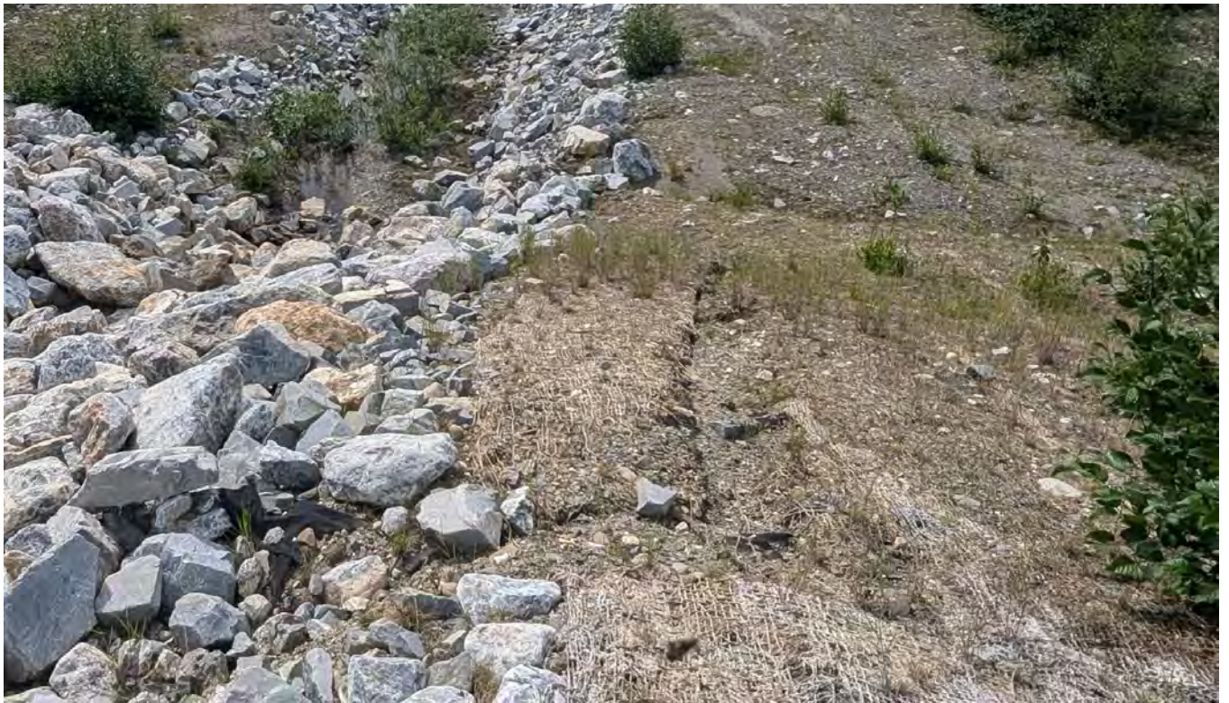
Photo SRS-02: Transverse crack across the dam crest approximately 1m east of the spillway seen from the crest of the SRS.
