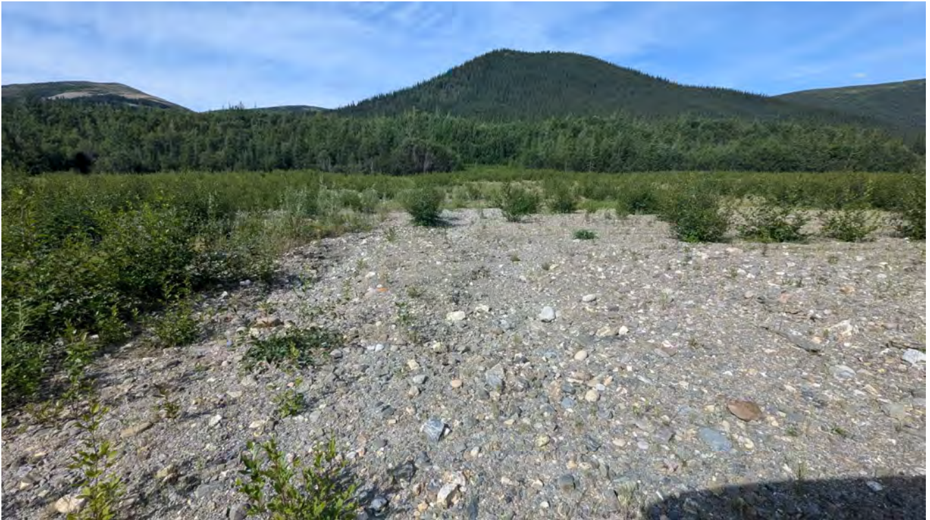
Photo TC-03: Eroded area of the cover where a drainage swale east of the main drainage swale of the cover flows to the west into the main drainage swale. No change in condition compared to the 2023 inspection.
