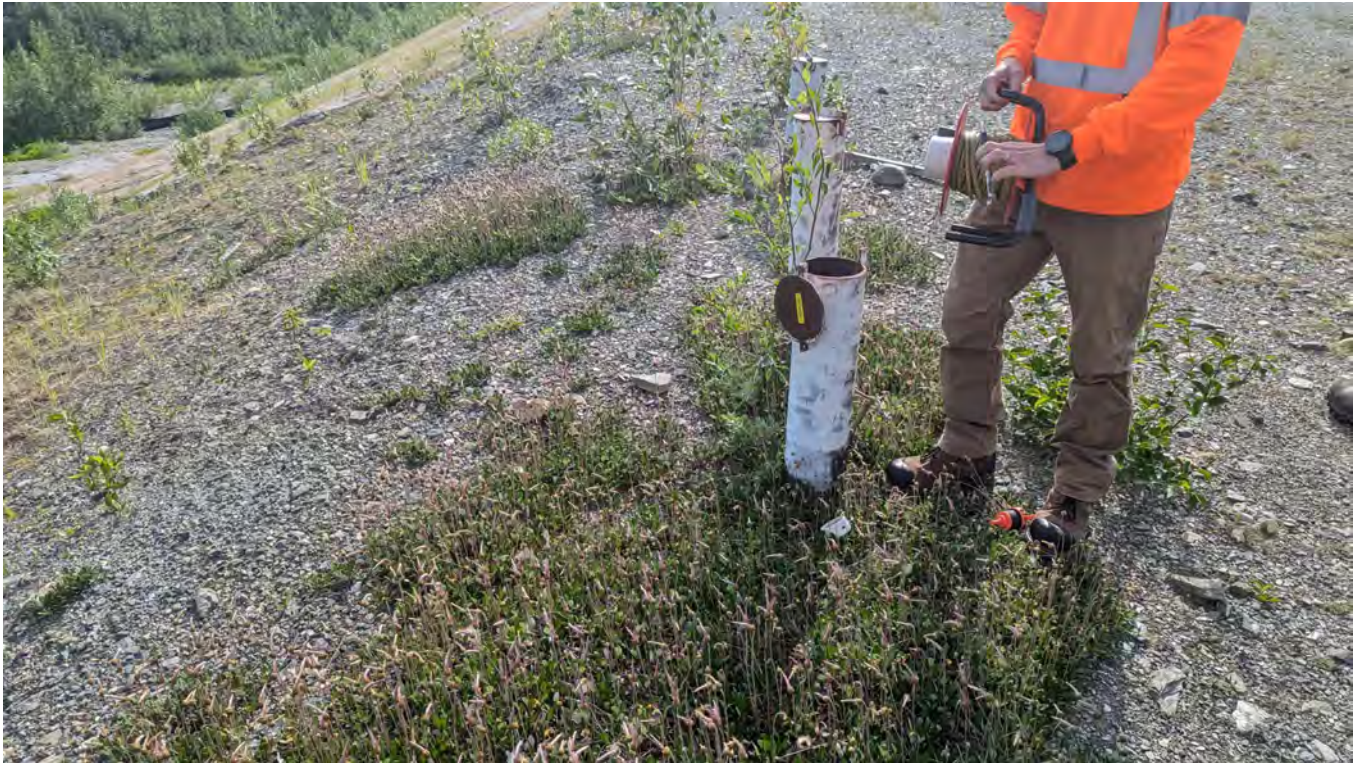
Photo NE-03: North Embankment crest piezometers casings.
