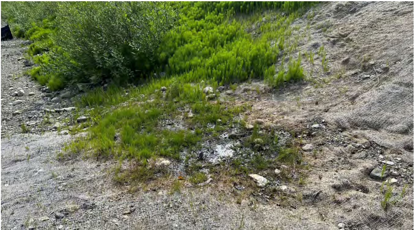
Photo NE-10: Seepage emerging from the French Drain in the 2022 repair area.
