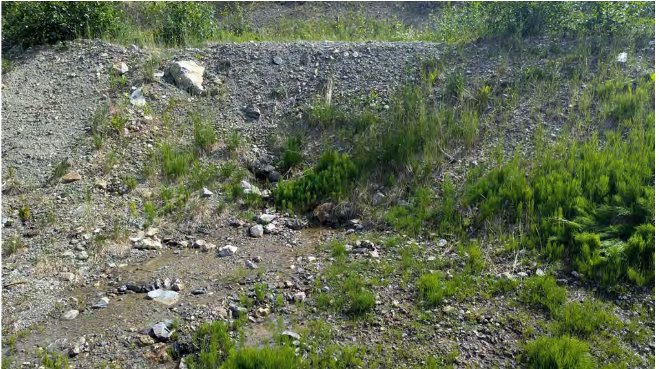
Photo NDC-03: Repaired area of the North Drainage Channel Berm where a slough was repaired in 2020 with a French Drain. Clear seepage was flowing through the base of the drain.
