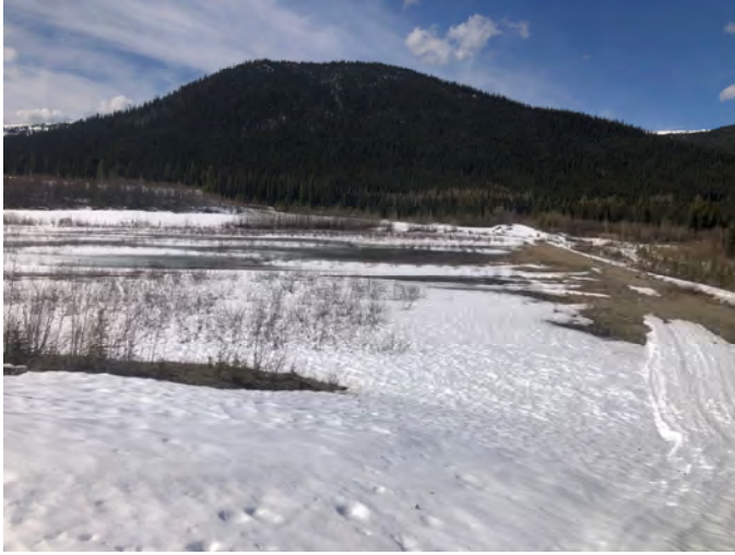
Photo C-1: Ponding adjacent to the North Embankment. Photo taken from East of the TMA looking west.
