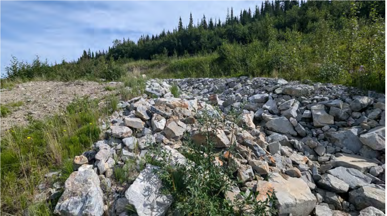
Photo NDC-01: Repaired area at the North Drainage Channel outlet where riprap movement was observed during the 2023 inspection.
