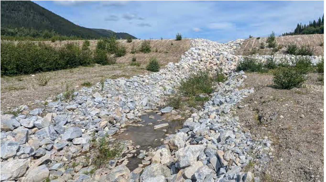
Photo SRS-03: Sediment accumulation and vegetation growth downstream of the SRS spillway. Looking upstream.
