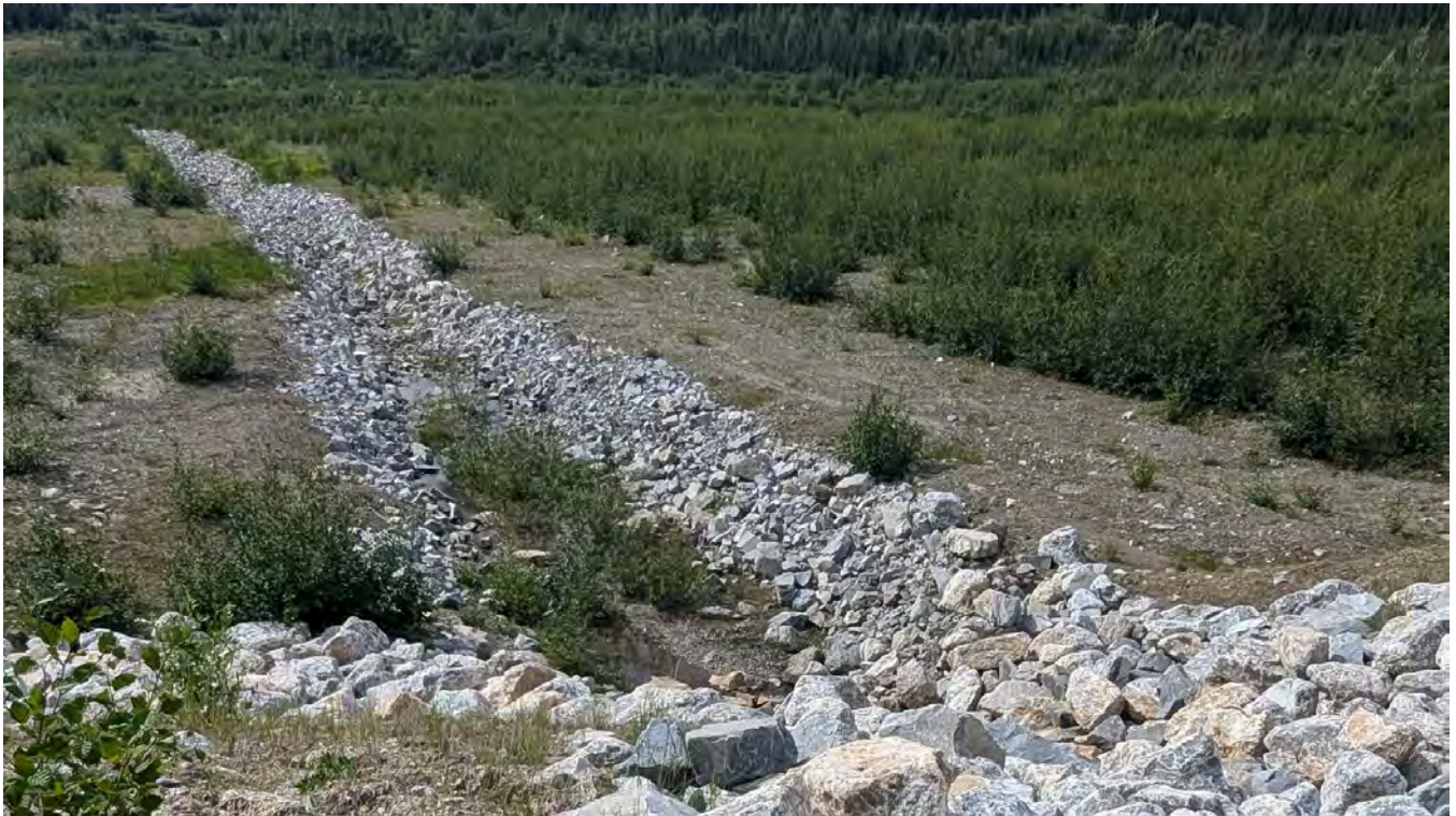
Photo DC-01: Upstream end of the South Drainage Channel immediately downstream of the SRS Spillway. Sediments are accumulating in the channel due to erosion at the base of the SRS spillway.
