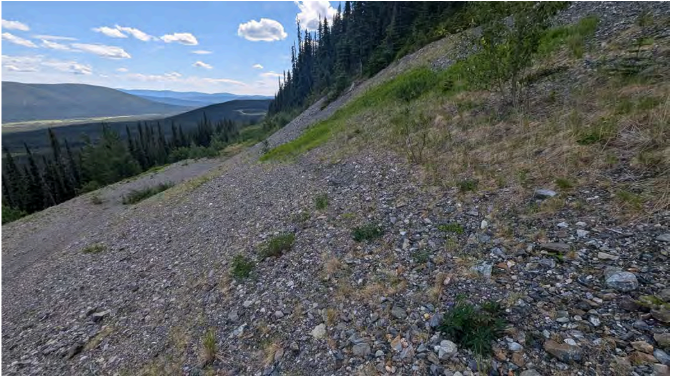
Photo WR-13: Regraded Burnick Waste Dump at the 1200 Portal. The minor settlement cracking observed during the 2023 inspection has partially filled with fine sediment.
