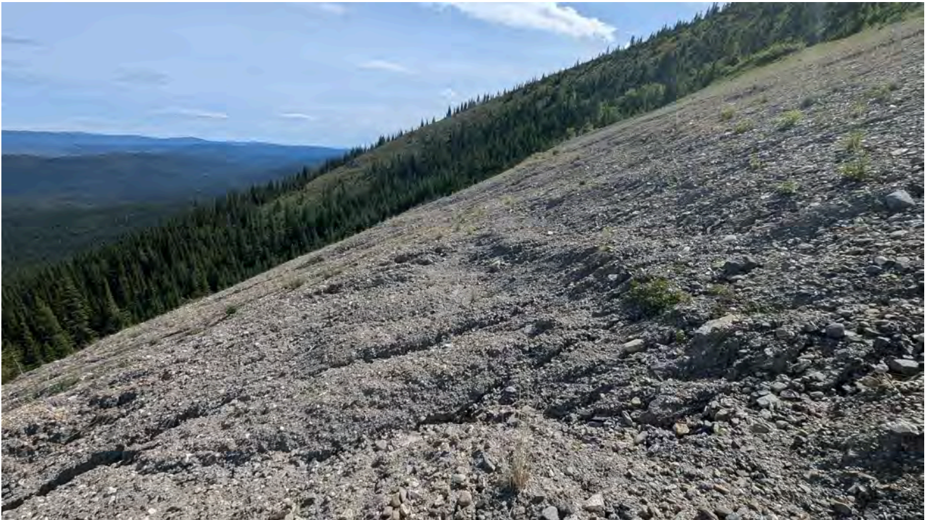
Photo WR-07: Surficial slumping near the south end of the 1408 Portal Waste Rock Dump.
