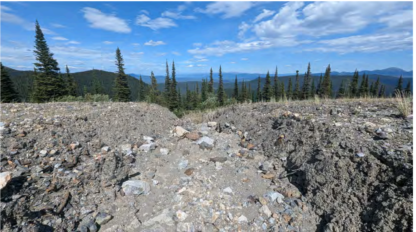
Photo WR-06: Erosion at the lowest point of the Jewelbox Waste Rock Dumps through the former Jewelbox Haul Road (looking northwest). Erosion has developed down to bedrock. Extent of erosion is unchanged compared to 2023 inspection.
