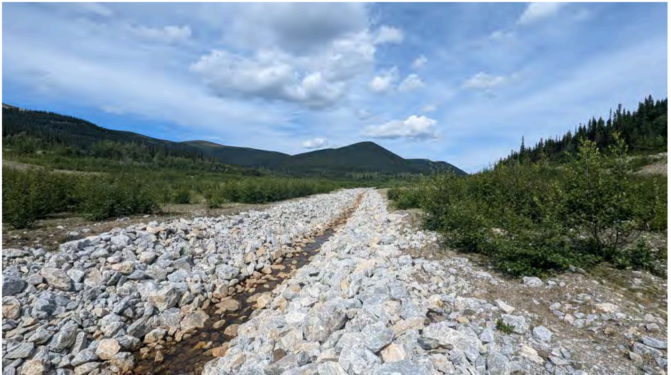
Photo DC-04: South Drainage Channel looking upstream from the confluence with the Camp Creek.
