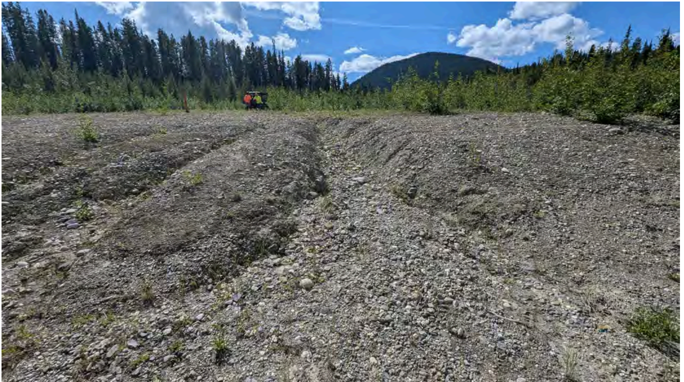
Photo L-02: Erosion channel that enters the Landfill drainage channel. The condition of the channel is unchanged compared to the 2023 inspection and no signs of debris were observed.
