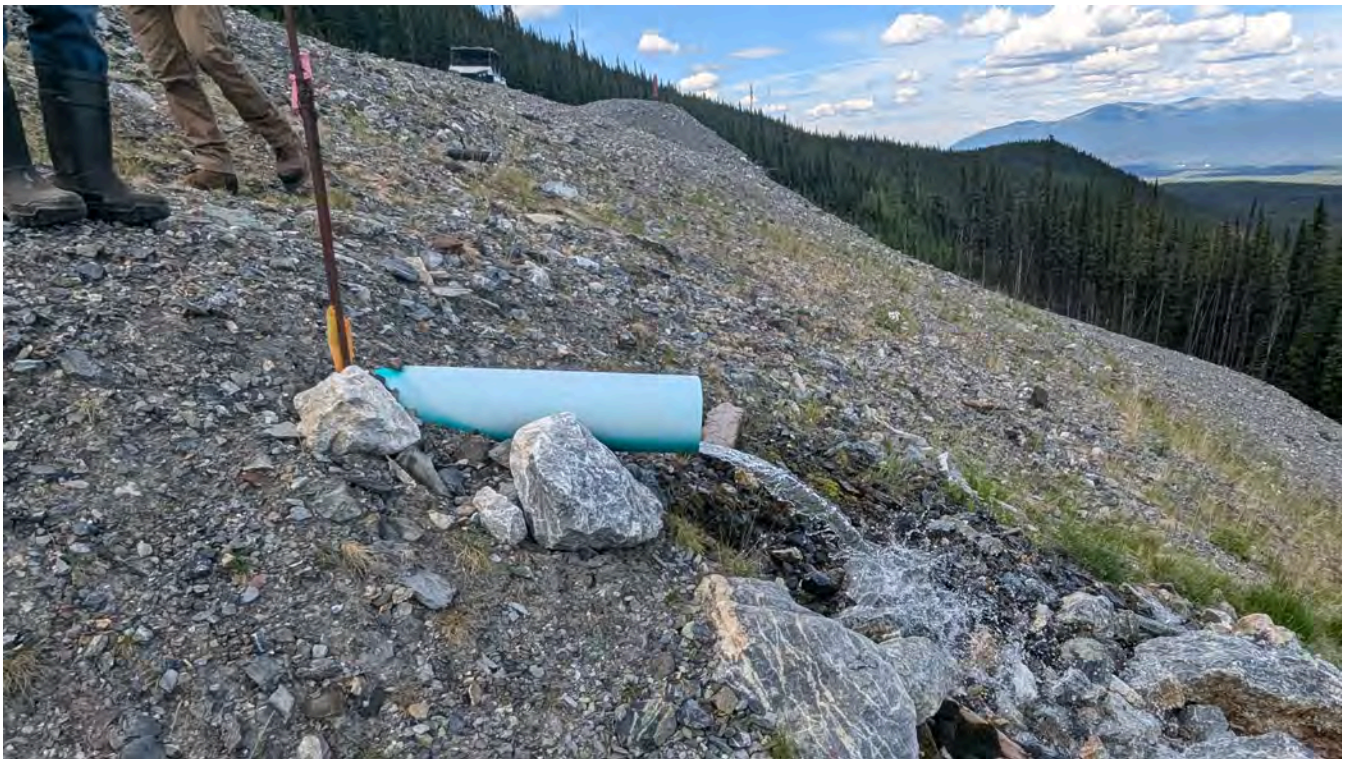
Photo WR-14: Drainage pipe at the Burnick 1200 Portal.
