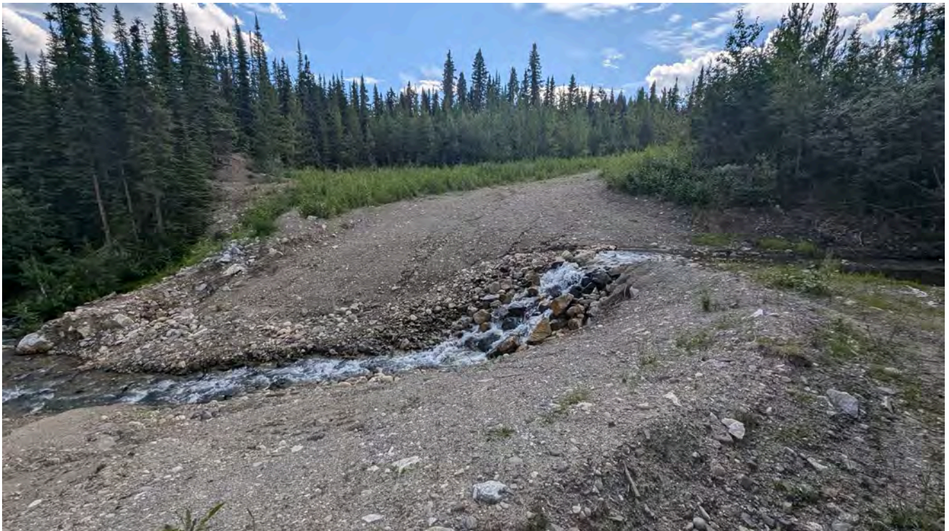
Photo NC-06: North Creek second crossing (to landfill) looking upstream. Maintenance was performed to return the slopes to approximately 3H:1V.
