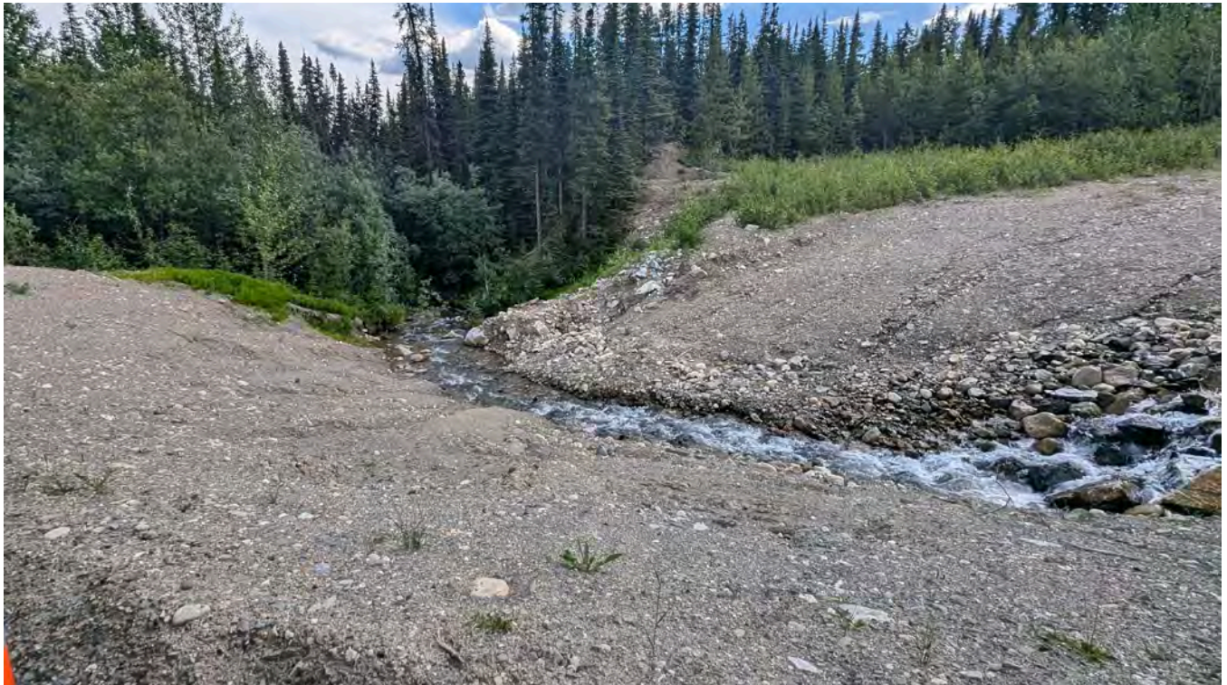
Photo NC-05: North Creek second crossing (to landfill) looking downstream. Maintenance was performed to return the slopes to approximately 3H:1V.
