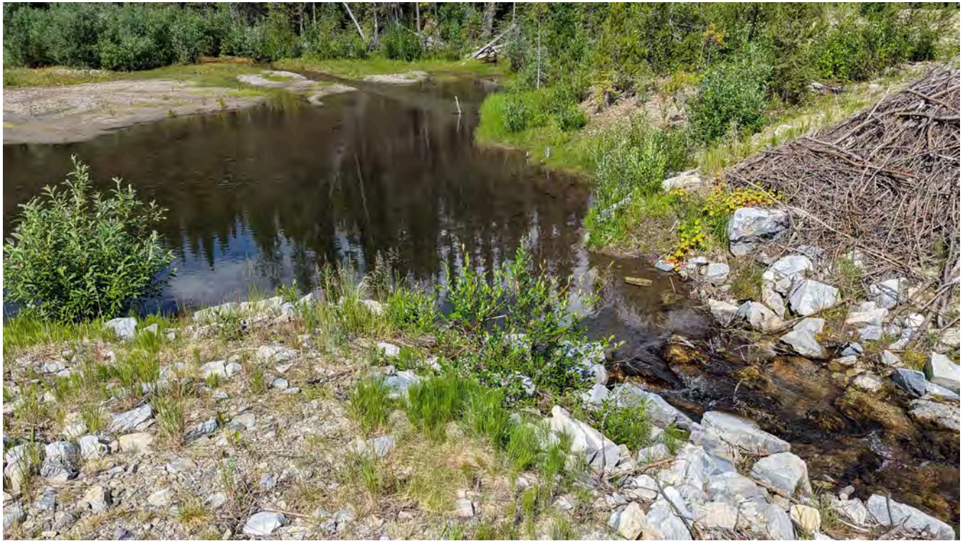
Photo NC-03: Former North Creek Dyke area. Inlet to the decommissioned dyke.
