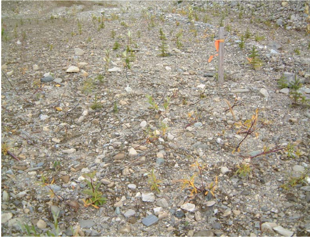
Km 22 main access road – grass seed germinating in depression downhill from test plots
