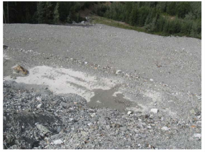
Figure 40 Erosion Gully on Slope Between Upper and Lower Benches and Water on Second Bench from Top (from WP 210)
