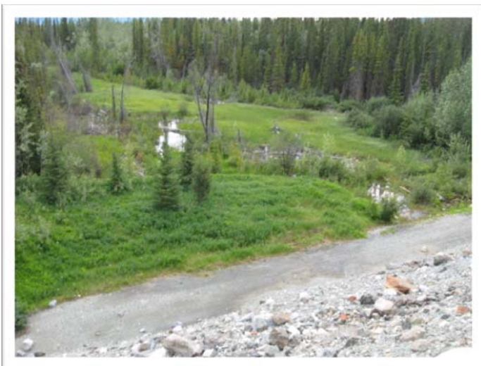
Figure 12 Ponded Water at Toe of Dyke
