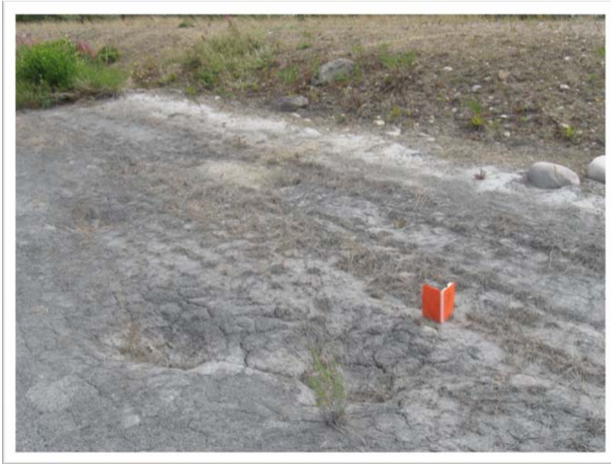
Figure 14 Depressions in Tailings Surface
