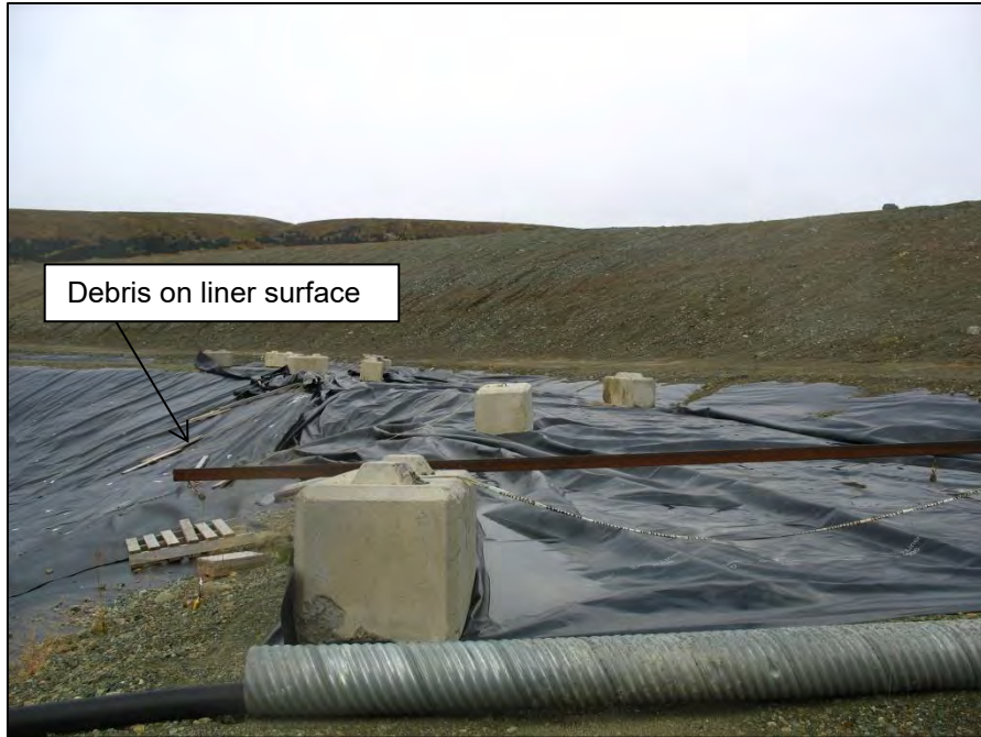
PHOTO 17 – TSF slump area cover material.
