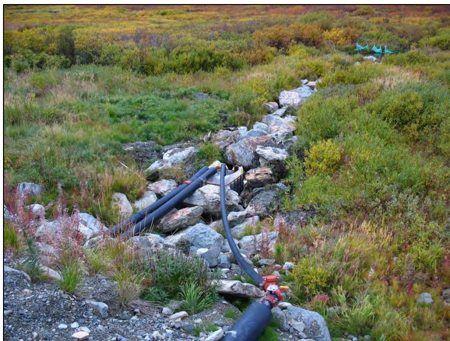
PHOTO 24 – TSF Underdrain Discharge Area at west side of the Seepage Collection Pond.
