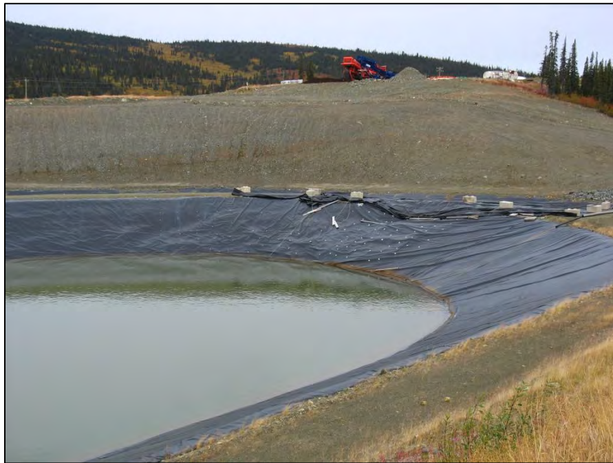
PHOTO 15 – North TSF Upstream Slope – Slump area.
