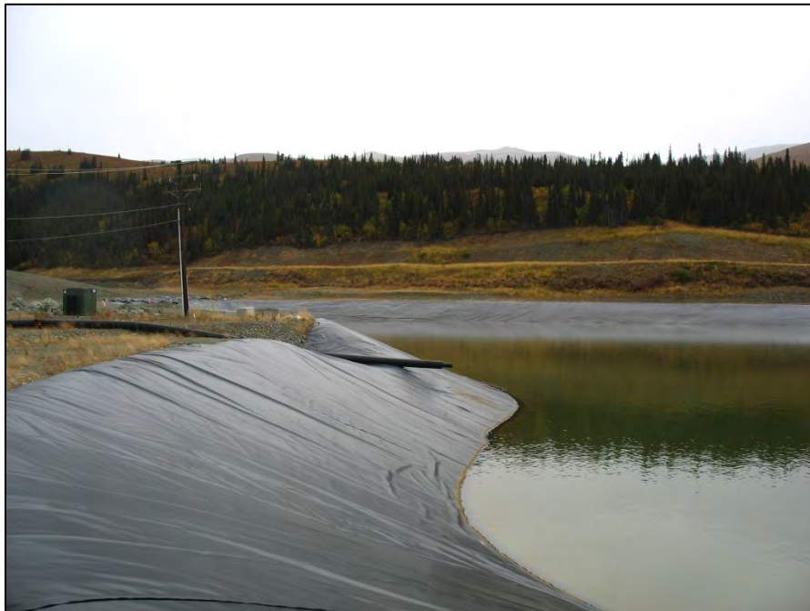
PHOTO 58 – East slope of lined TSF. Note diagonal lines on the liner which may be an indicator of liner stress.
