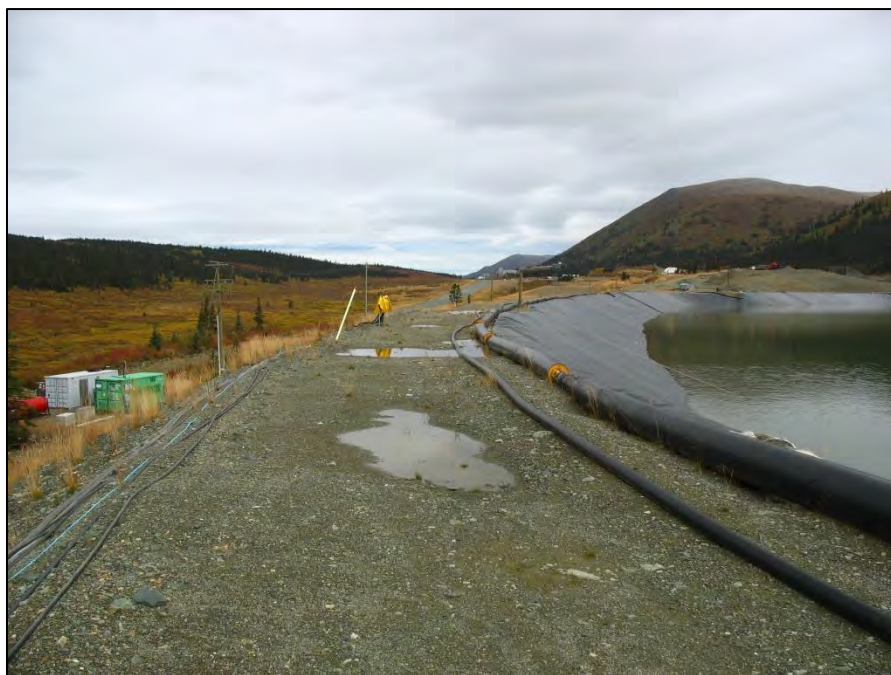
PHOTO 10 – TSF West Embankment – Ponding on crest
