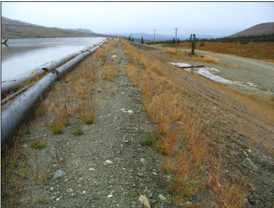
PHOTO 12 – TSF West Embankment crest looking south. Ponded water at toe.
