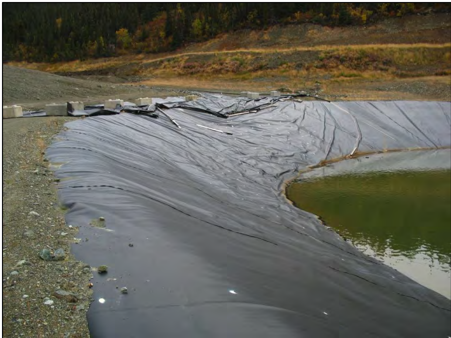
PHOTO 14 – North TSF Upstream Slope – Slump area.
