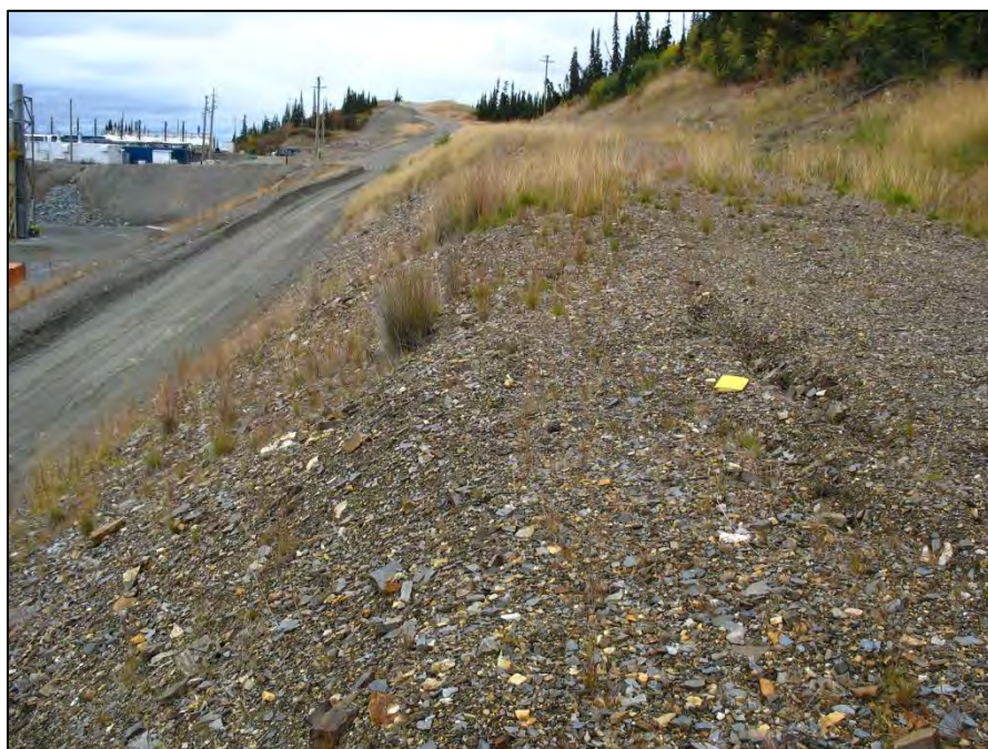
PHOTO 46 – Ditch 1 – Tension crack in berm fill material.
