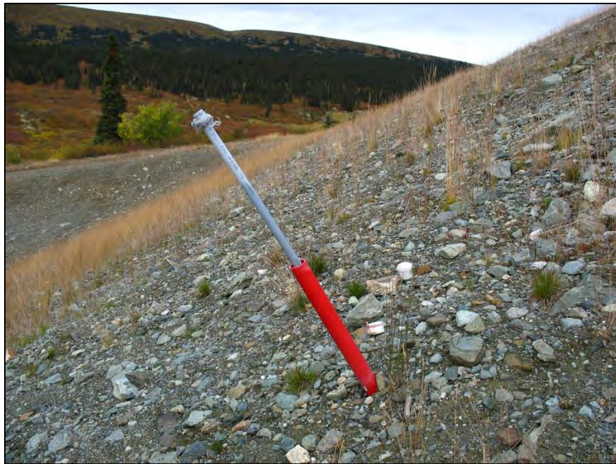
PHOTO 8 – TSF South Embankment – Pipe stuck in inclinometer – no longer functioning.
