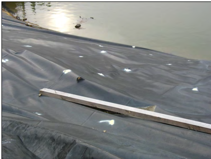
PHOTO 16 – TSF slump area – Liner damage
