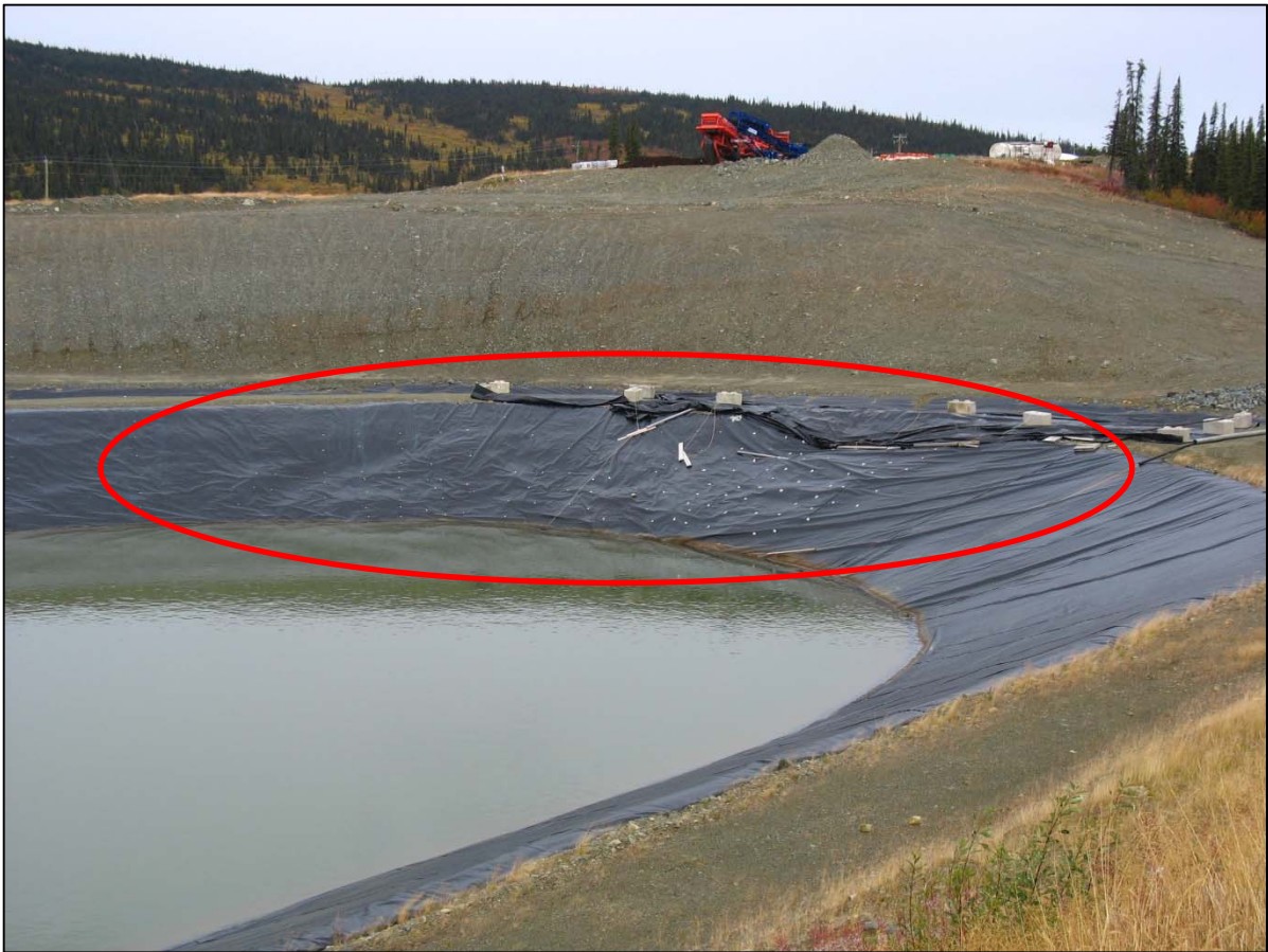
Figure 3.1 Slump at North End of TSF
