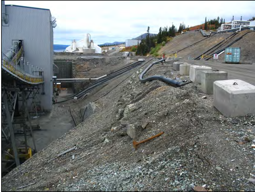
PHOTO 57 – Slope upstream of MSE Wall – Small tension cracks observed on downstream site of access road.
