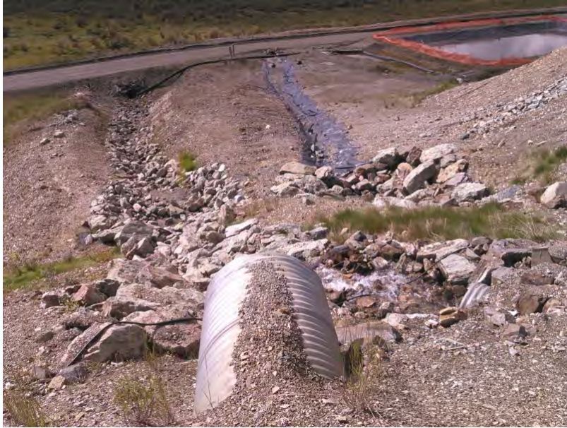
Figure 3 – Outlet of culverts draining to the environment and Ditch #3. Culvert outlet at the right with running water connected to groundwater collection and was observed with significant flows.
