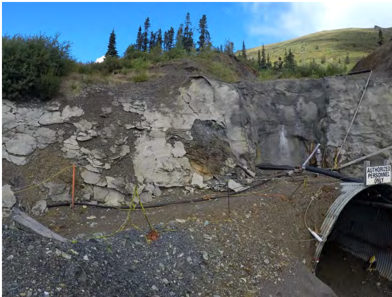
Figure 38 – Mine Portal, some shotcrete has come loose and fallen from the slope. Exposed bedrock appears relatively stable, but could be erodible under flow and/or weathering.
