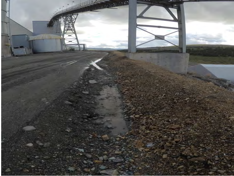
Figure 19 – Ditch #5 manhole located at the top of the MSE wall on the west side of the Mill Pad.
