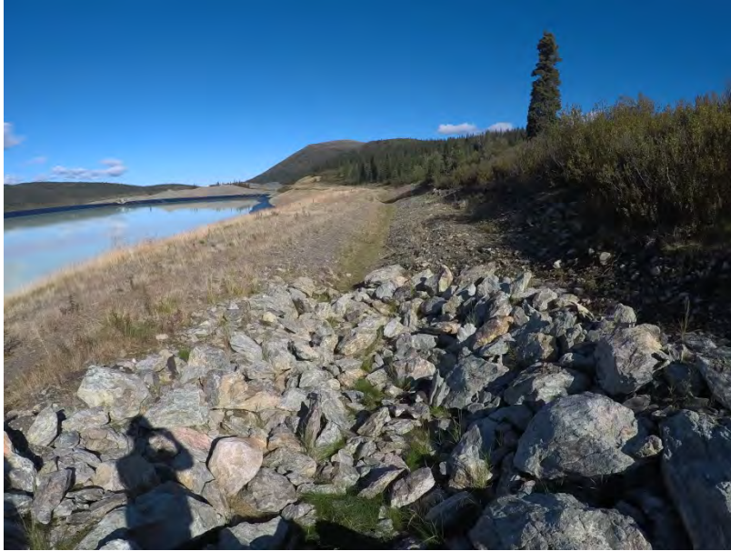
Figure 31 – Diversion Ditch B facing north and located above and on the east side of the TSF.
