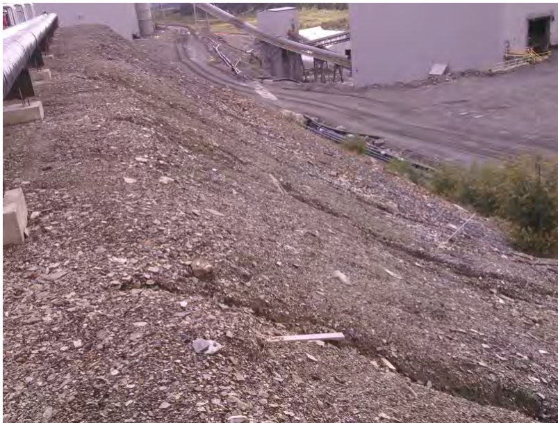
Figure 10 – Embankment slope below Generator Pad, small rill erosion can be observed.
