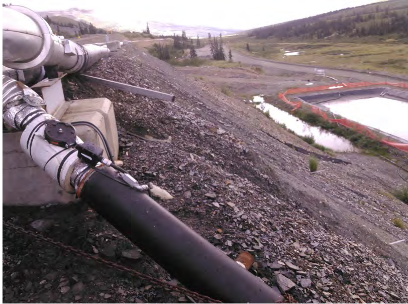
Figure 1 – Erosion down slope of mill pad. Repairs from previous years using rip rap and non-woven geotextile can be observed in the background.
