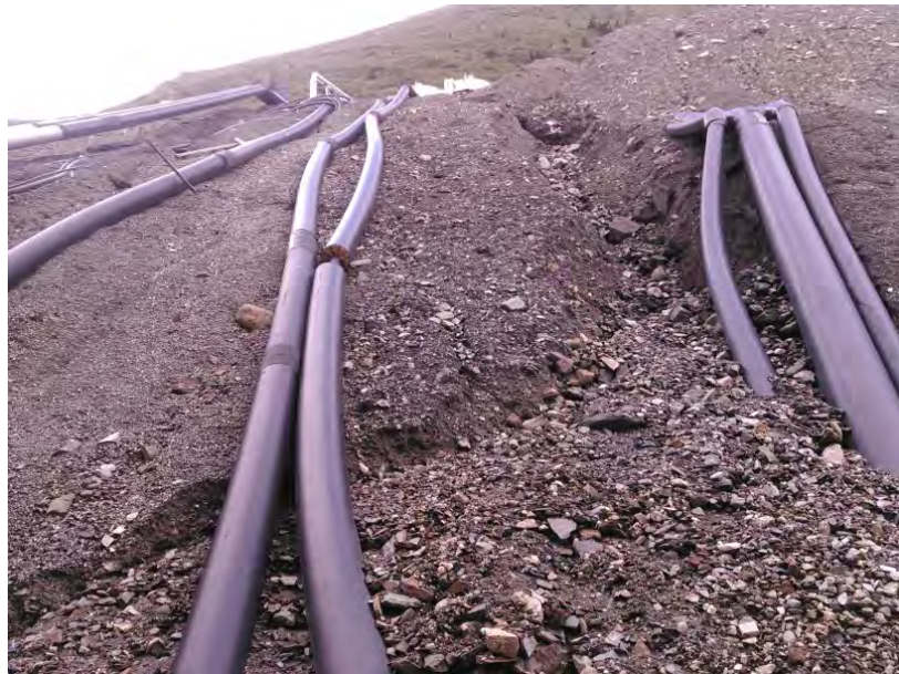
Figure 2 - Base of erosion from North West corner of Mill Pad.
