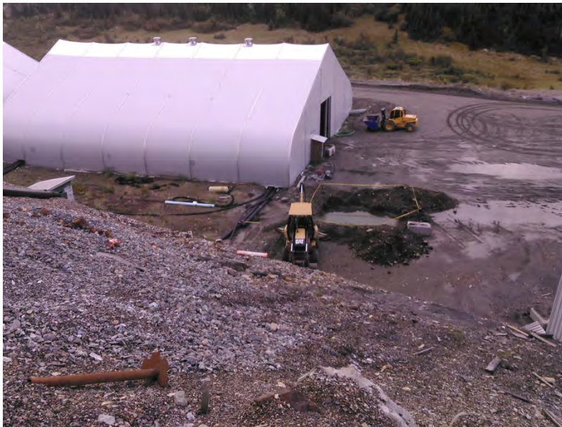
Figure 12 – Recently constructed sump excavated upstream of Sump #2 in order to control flow during the relining of Sump #2.
