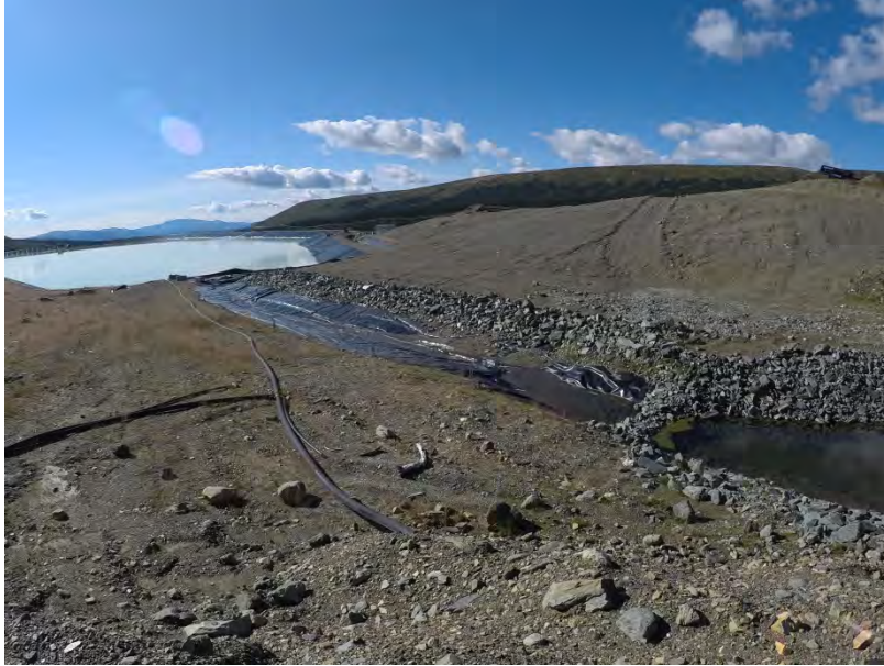
Figure 33 - Diversion Ditch A, beginning of lined portion of drainage ditch which flows along the southern edge of the tailings pond.
