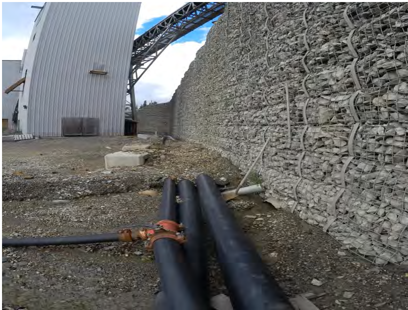
Figure 6 – MSE wall facing North West towards the crusher and conveyor belts. Culvert from Ditch #5 can be seen in the lower right section of the photo.
