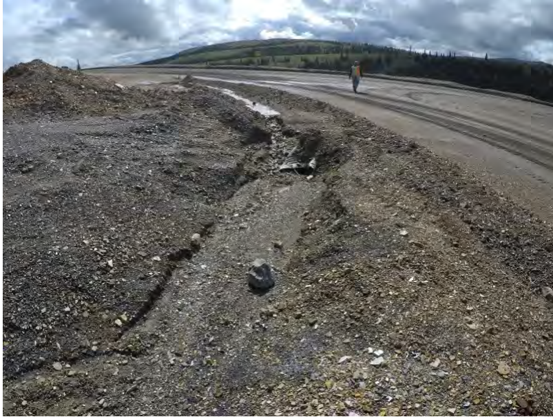
Figure 15 - Ditch #1 culvert at the south end of the Mill Pad. Buildup of sediments and damage to the culvert can be seen.
