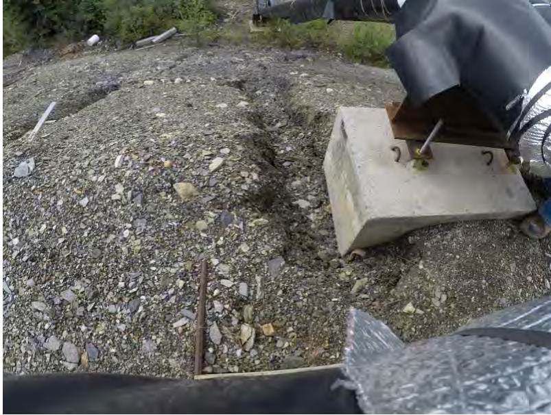
Figure 9 – Erosion undermining concrete anchor at the North West side of the Fuel Pad.
