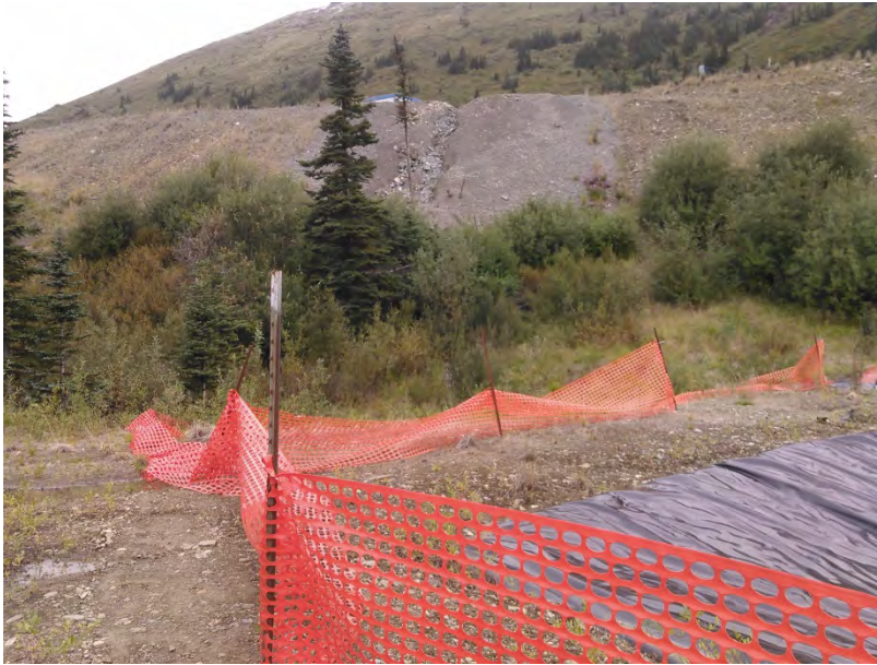
Figure 20 – Previously repaired erosion along the Camp Pad as seen from the Sewage Pond.
