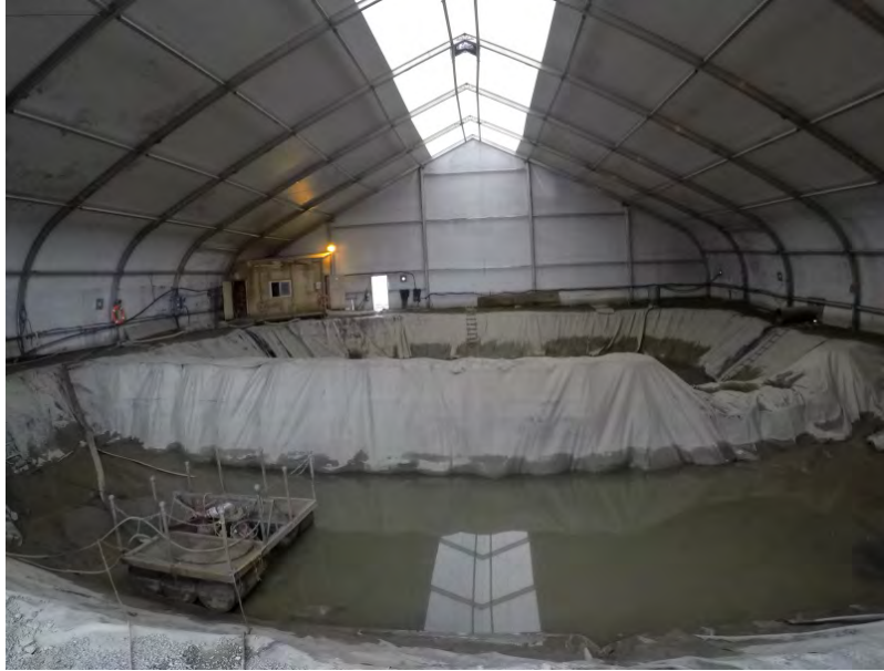
Figure 11 – Sump #2 being drained for replacement of liner, drainage from Ditch #3 visible at the right of the photo.
