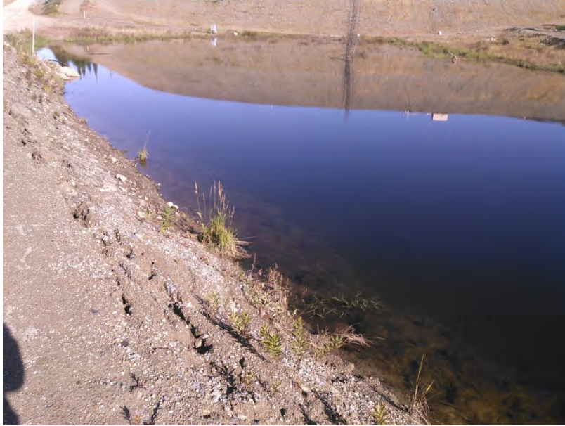
Figure 29 - Seepage Pond downstream of the TSF. Wolverine access roadway serves as dam. Embankment slope has settled causing over steepening of slope as well as tension cracks.
