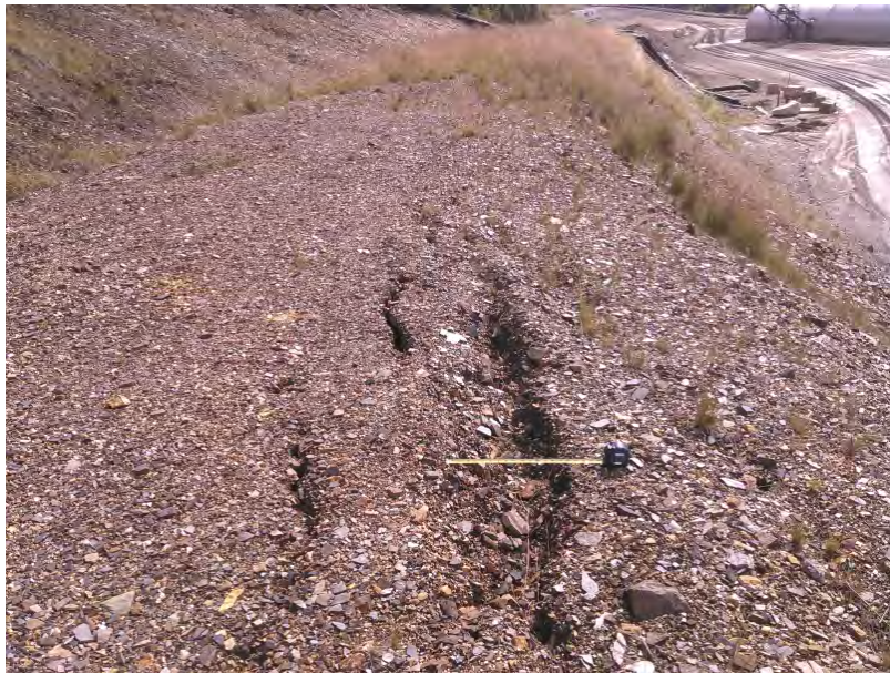
Figure 14 – Settlement/tension cracks observed in berm adjacent to Ditch #1. Area has been noted in previous reports and no new indication of soil distress was noted.
