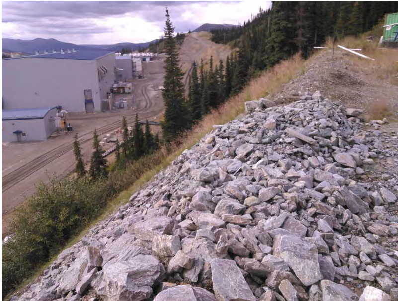
Figure 22 – Recently repaired erosion rill due to heavy rainfalls located in the North West corner of the Camp Pad facing north.
