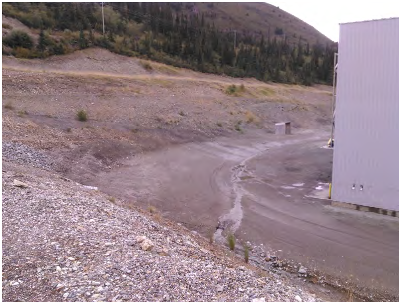
Figure 4 – Embankment seepage from North West corner of the Mill Pad. Toe of the embankment paralleling Diversion Ditch #1, water flows to Ditch #5, shed at centre of photo contains vertical sump pump.
