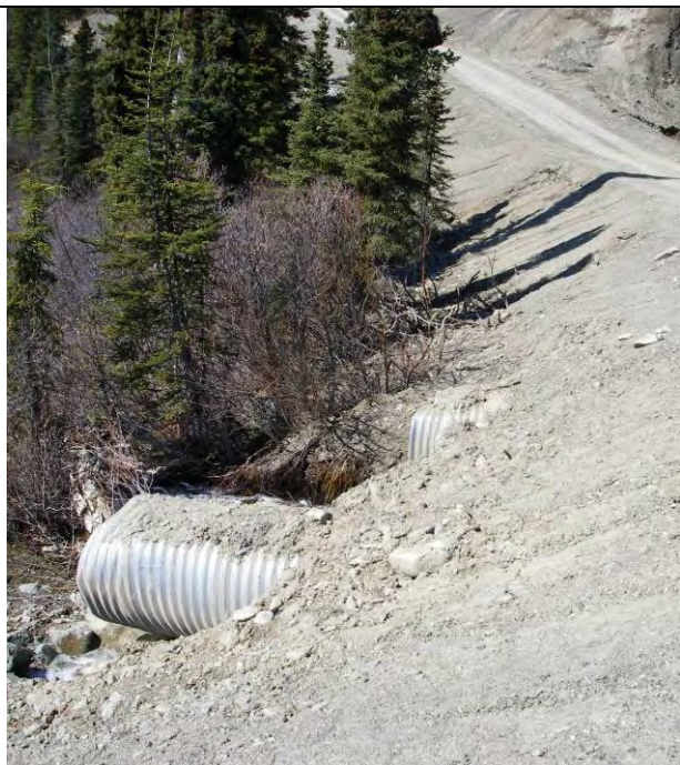
05/21/07 South slope of road at gorge area; facing N
