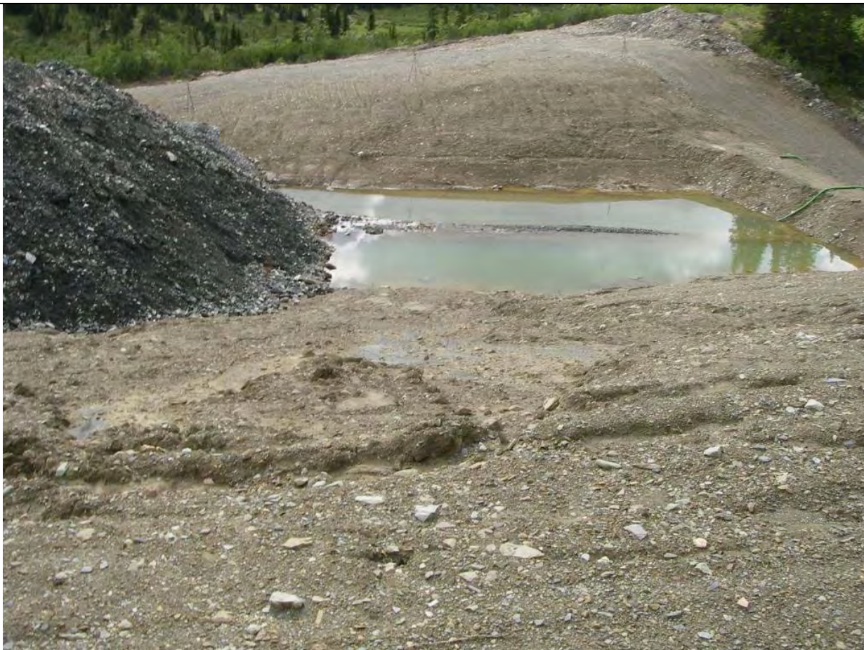
07/07/07 Slumping of clay liner on East side of WRP (facing W)
