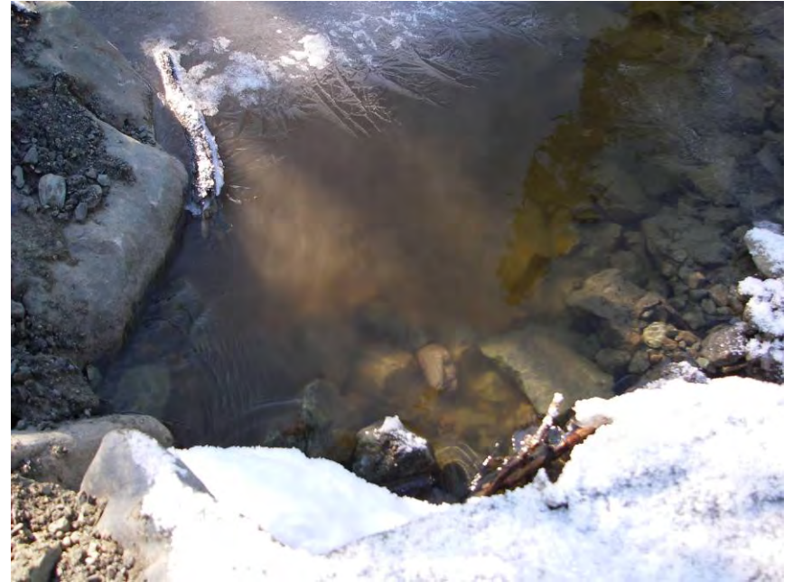
Silt flowing into the culvert
