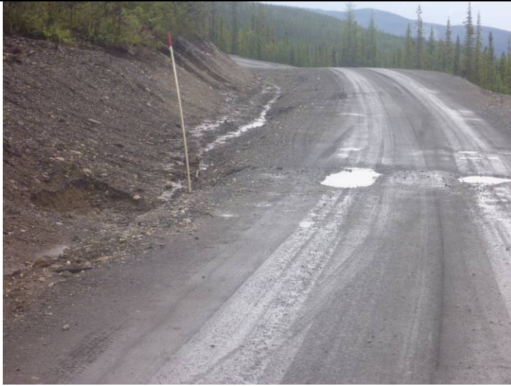
KM11.2 Erosion in the ditch
