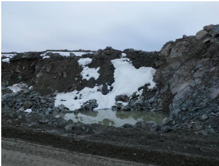
Photo 11 (11/05/20) Pool of water at KM 19.2 – may be seeping through road
