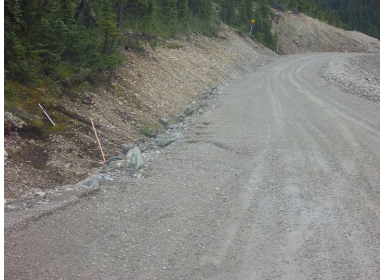
KM17 Erosion into the road
