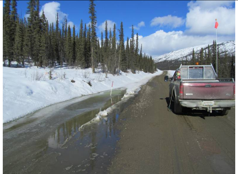
11/04/01 Km 10 blocked culvert requiring steaming
