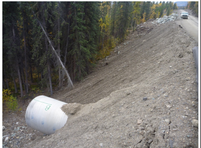
Photo 4 (Sept 13, 2011): km 4.6 Looking north - fill-in tension cracks and erosion channels along west side of the road cut and fill slope.
