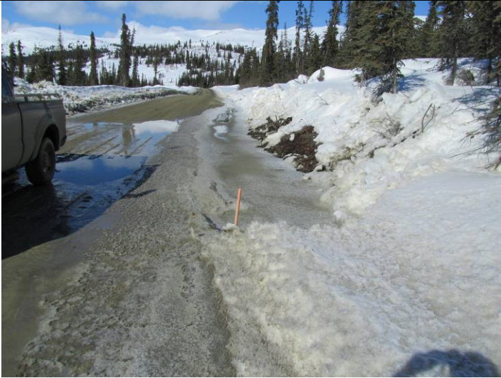
11/04/01 Km 23+050 blocked culvert requiring steaming
