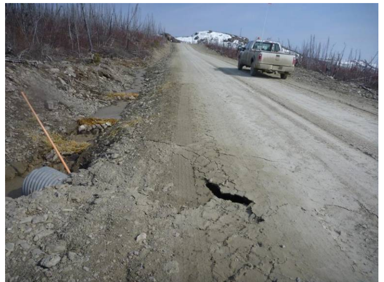
Photo 4 (11/05/18) Cave-in on road caused by culvert being undermined by high water flow
