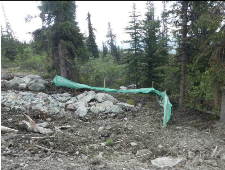
Photo 1 (11/06/17) Before (silt fence has fallen down)
