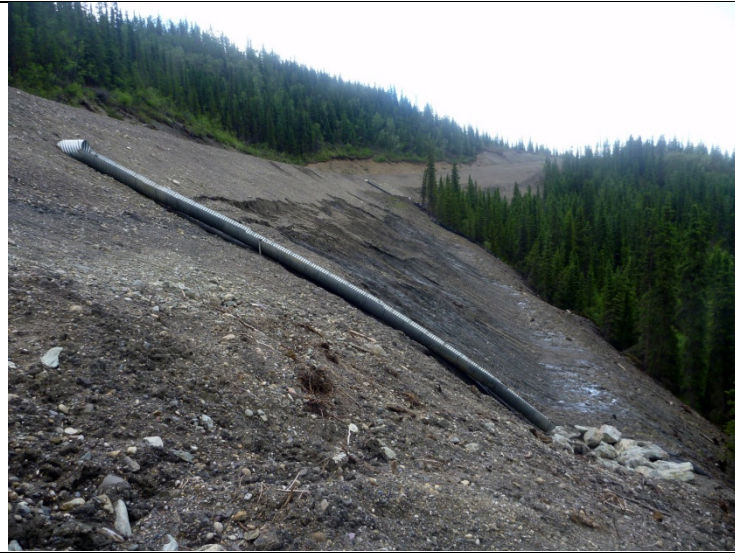
Photo 5 (July 1, 2011): km 9.5 Looking south - tension cracks & erosion channels down slope of the road. Note: Visible water seepage through sand/gravel.
