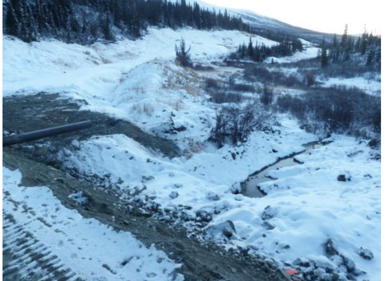
Photo 4 (11/10/21) The french drain runs under the Pad and exits here (south end) through a culvert. Is working great.
