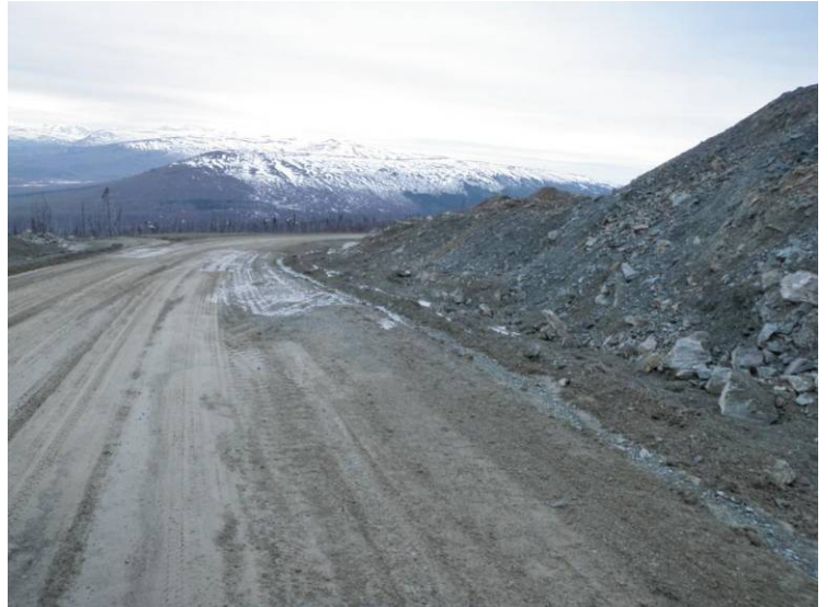
Photo 12 (11/05/20) More water seeping through ground and may be sourced from opposite side of road
