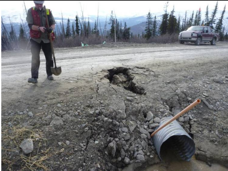
Photo 5 (11/05/18) Cave-in at KM 19.5 due to culvert being undermined by water
