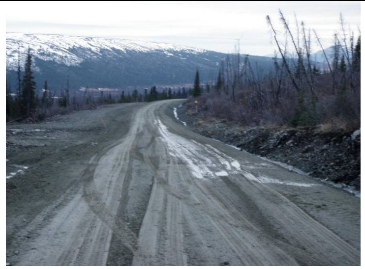
Photo 10 (11/05/20) Water seeping from middle of road at KM 20
