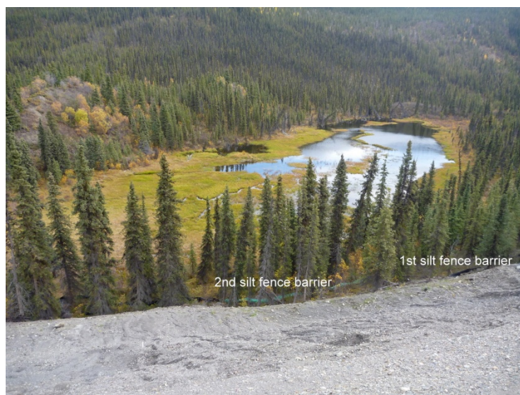
Photo 7 (September 13, 2011): km 9.5 Looking west – portion of 1 st silt fence barrier covered by moving sand/gravel. 2 nd silt fence still in place at the toe.
