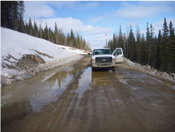
11/04/08 Km 4+500 blocked culvert requiring steaming
