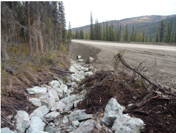
Photo 3 (Sept 13, 2011): km 4.6 Looking south - fill-in tension cracks; laid geo-membrane and placed rip rap on east side of road fill slope.
