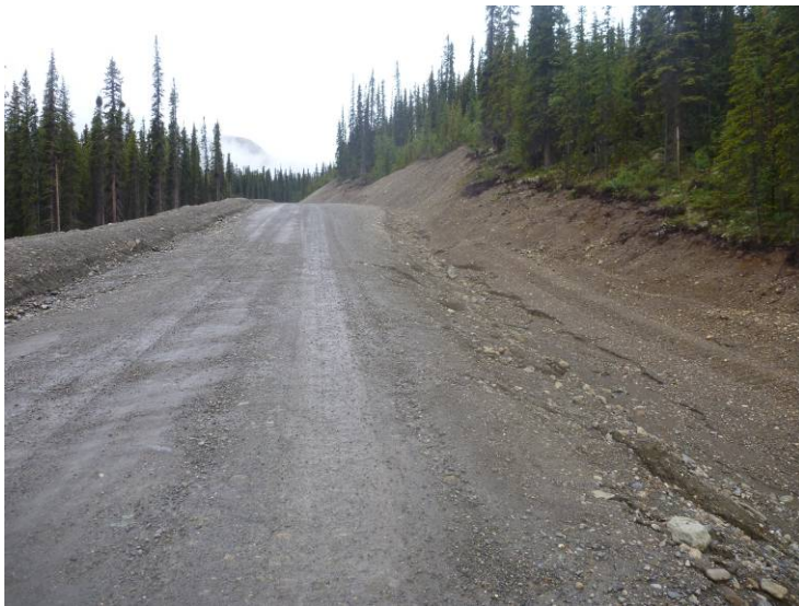
KM11 Water rills throughout the road going into the ditch across road, loose sandy material
