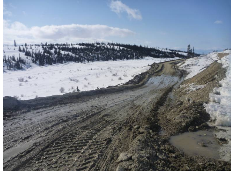
11/04/08 Pooling water and mud at lower bypass Km 27+300
