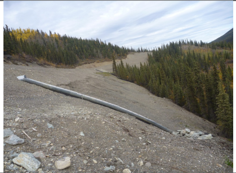
Photo 6 (September 13, 2011): km 9.5 Looking south - tension cracks & erosion channels down slope of the road. Note: No visible water seepage.
