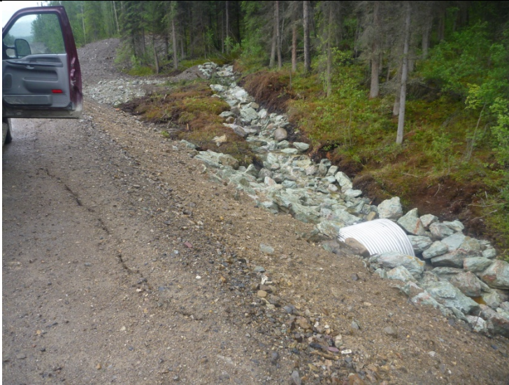
Photo 1 (July 1, 2011): km 4.6 Looking north - tension crack on east side of road.
