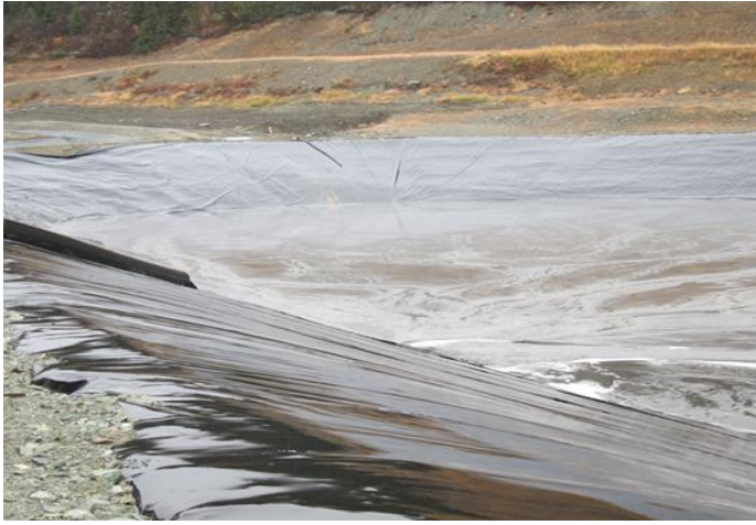
Photo 1: Looking at discharge location at south-west corner side of TFS showing liner movements in the west wall.
