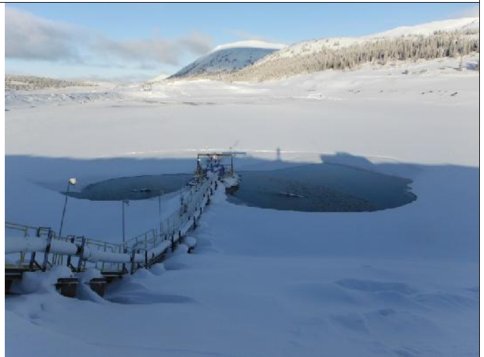
Photo 4: Barge with new de-icing pump effectively opening up the area around barge
