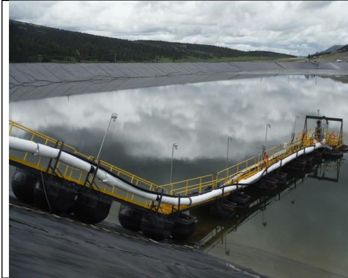
Photo 1: Looking at barge pumping station and discharge line –walk way @East dam & the South wall of TSF
