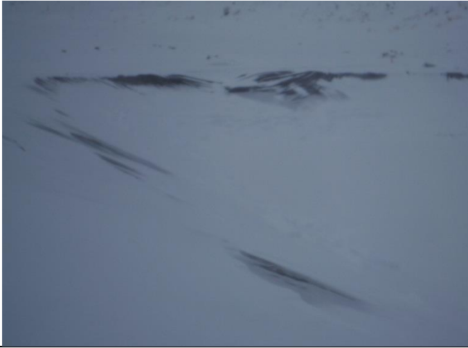
Photo 1: Looking at south-west corner side of TSF showing liner movements in the west wall.
