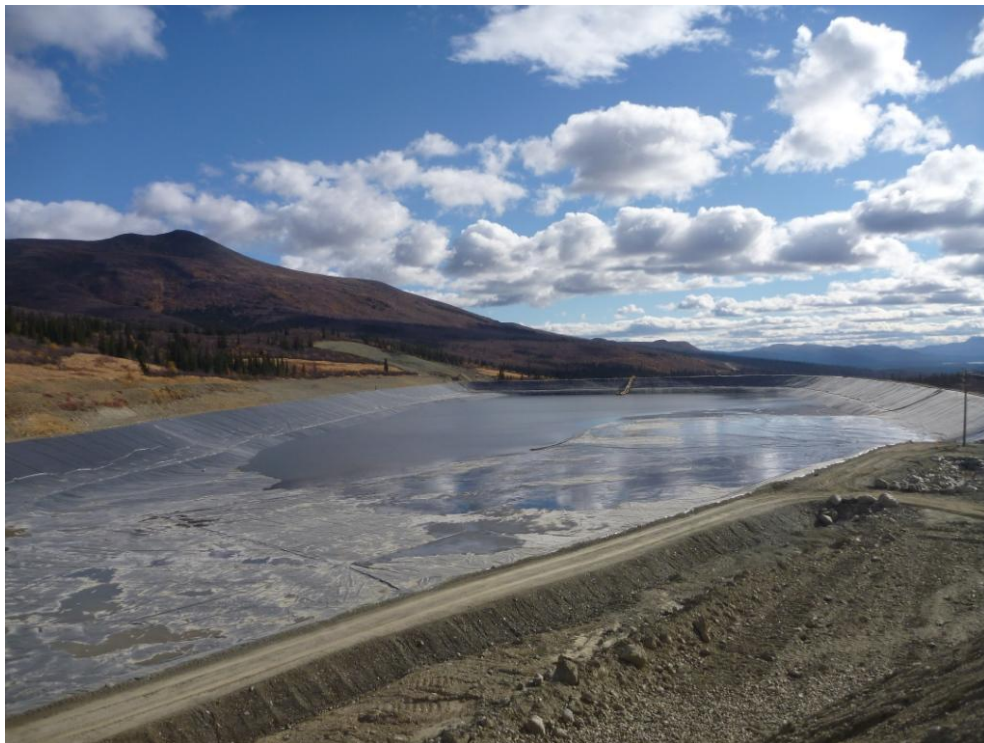
Picture 2-1: Tailings storage facility after dam lift construction project, looking east (top) and west (bottom).
