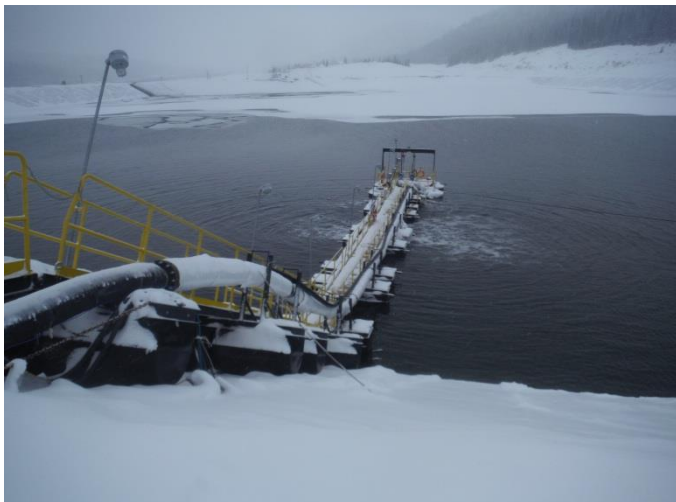
Photo 7: Closer picture of barge pumping station.
