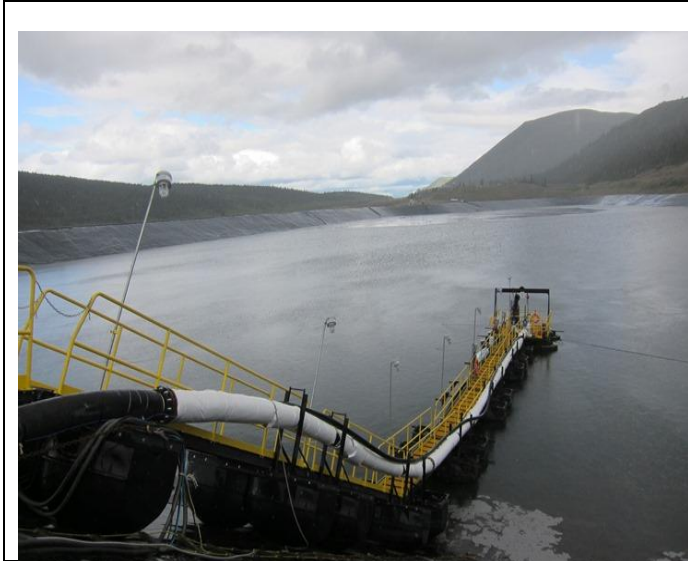
Photo 1: Looking at Barge pump station & its discharge line from East side of TSF
