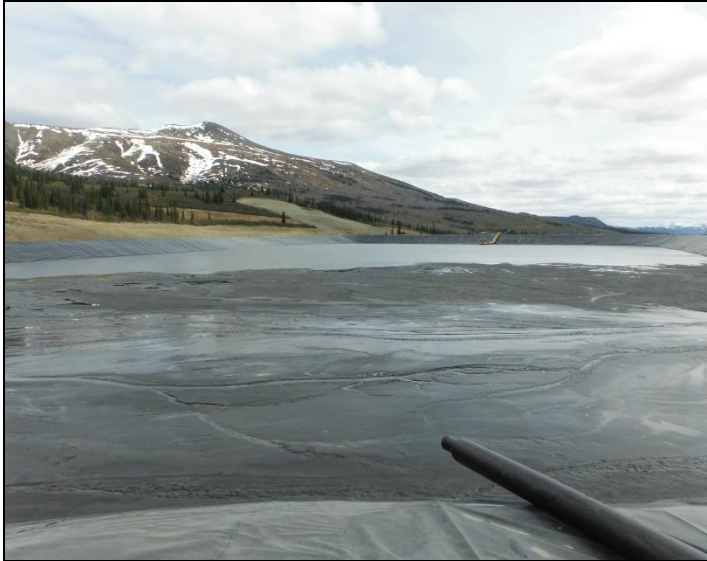
Photo 1: Looking at transfer station over flow line from North West corner of TSF
