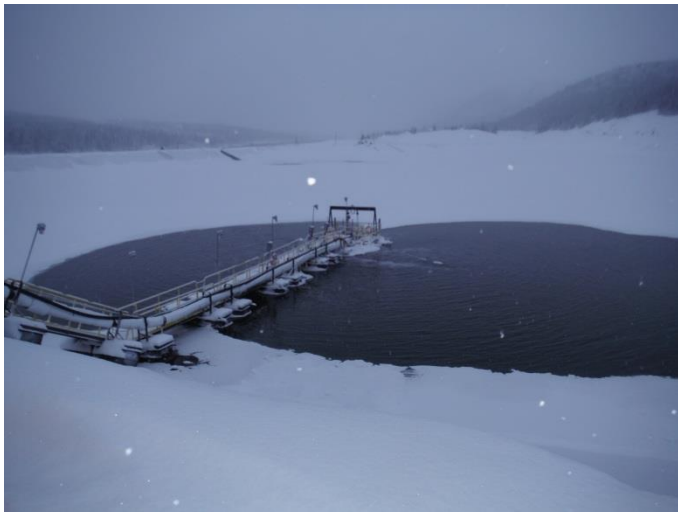
Photo 7: Closer picture of barge pumping station.
