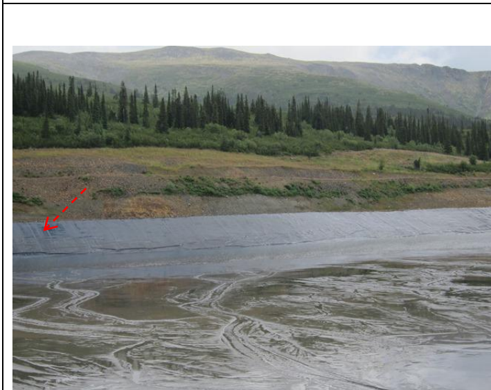
Photo 7: looking at north side of TSF showing ripples on the left corner liner of wall.
