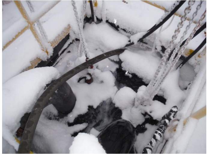
Photo 6: Closer view of barge pumps.
