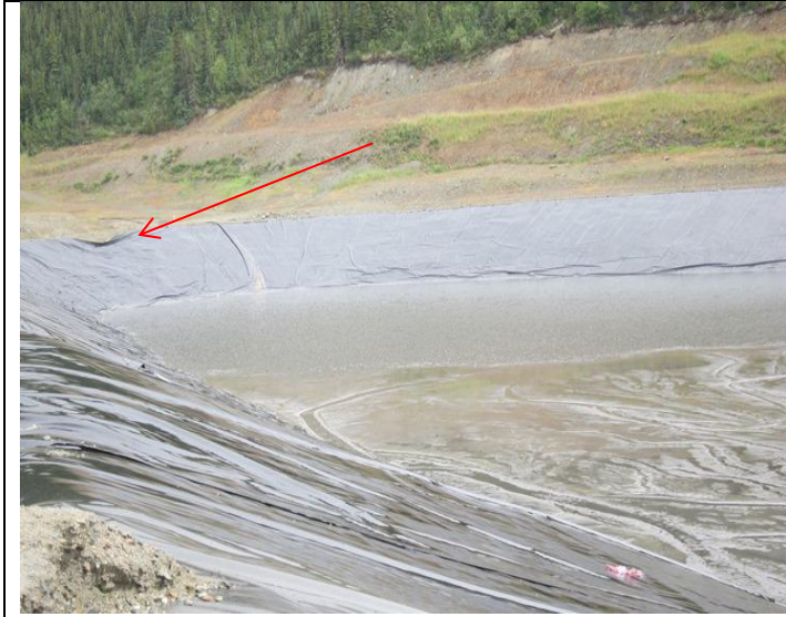
Photo 5: looking at south-west corner bank showing distorted liner at left corner of west wall.
