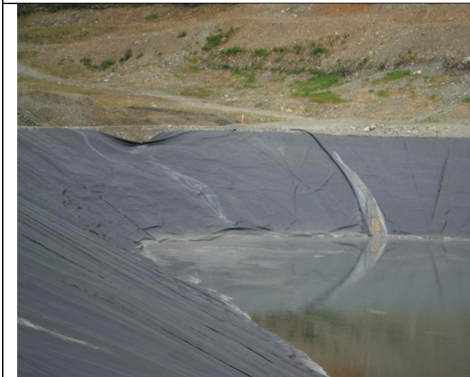
Photo 3: West wall view with slough at upper crest of west wall & disturbance/movements underneath the liners.
