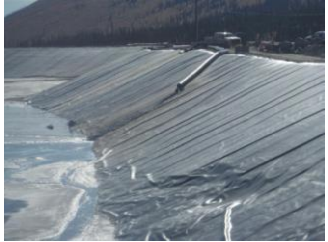
Photo 2: Looking at north-west corner of TSF showing current location of discharge line.
