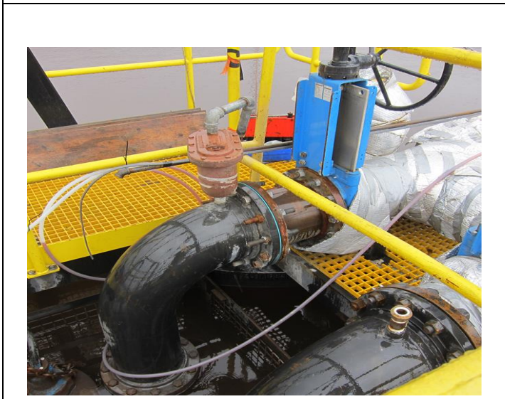
Photo 7: Closer picture of barge pumping station.
