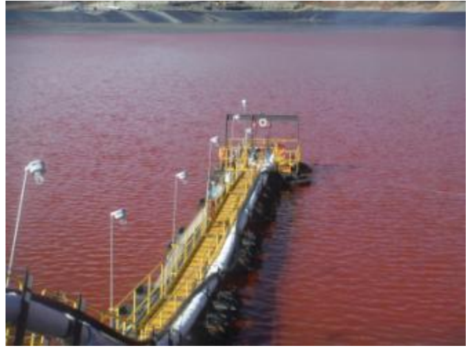
Photo 6: Closer view of barge pump system.
