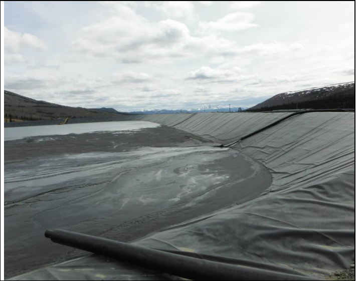
Photo 2: Looking at south wall from North West corner of TSF with Tailing discharge line in foreground.
