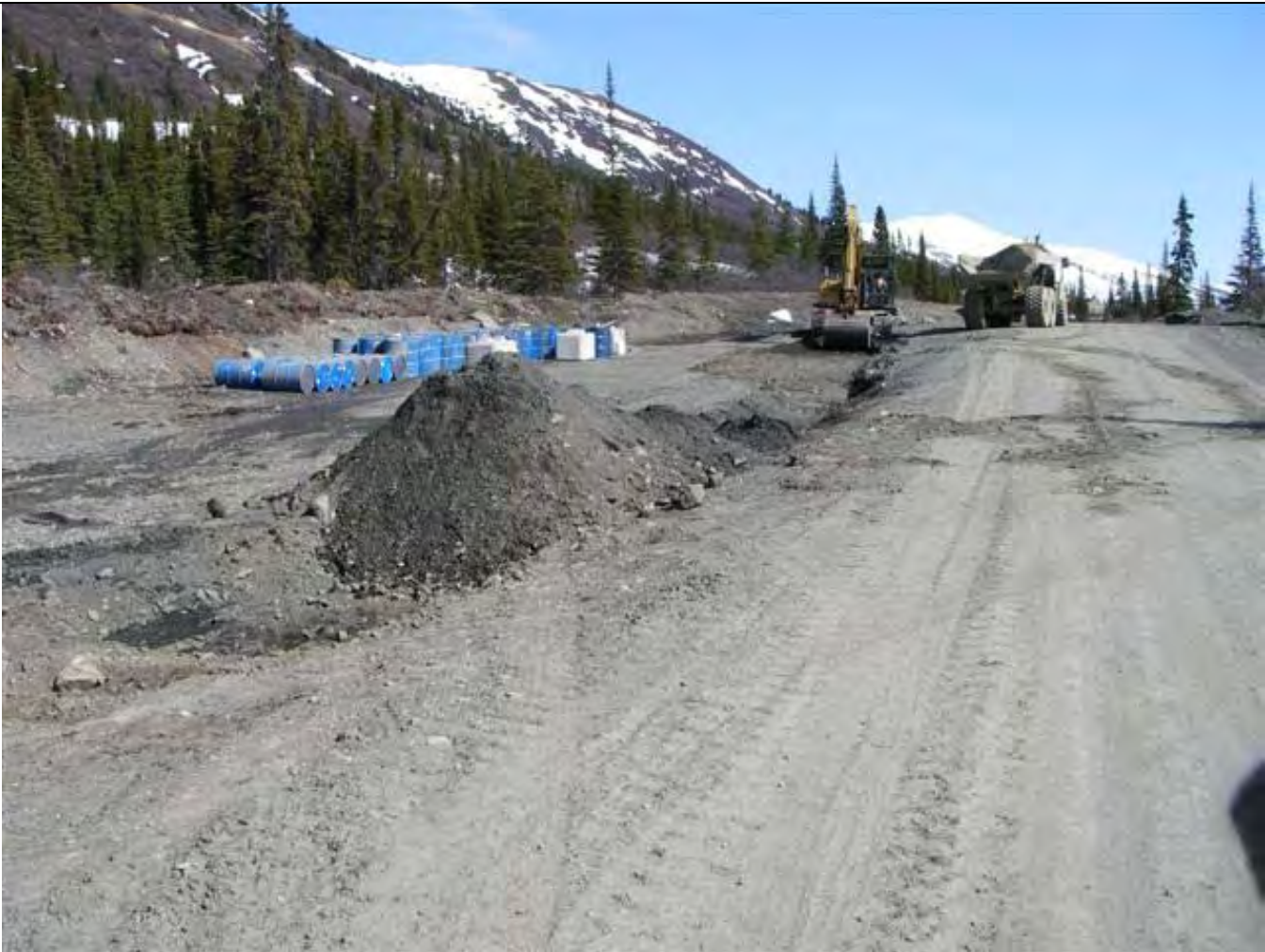
Photo 5. After the drums were moved from Cache A north to Cache B; midway through excavation of the contaminated soil. The red line outlines the contaminated area viewed from the north-west, looking down the site road towards the portal area. Taken May 23, 2007.
