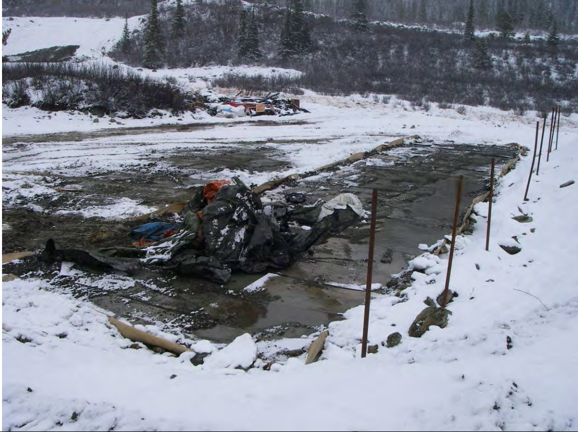
09/27/07 soil storage area, after soil removal – used tarps piled at west end; facing north
