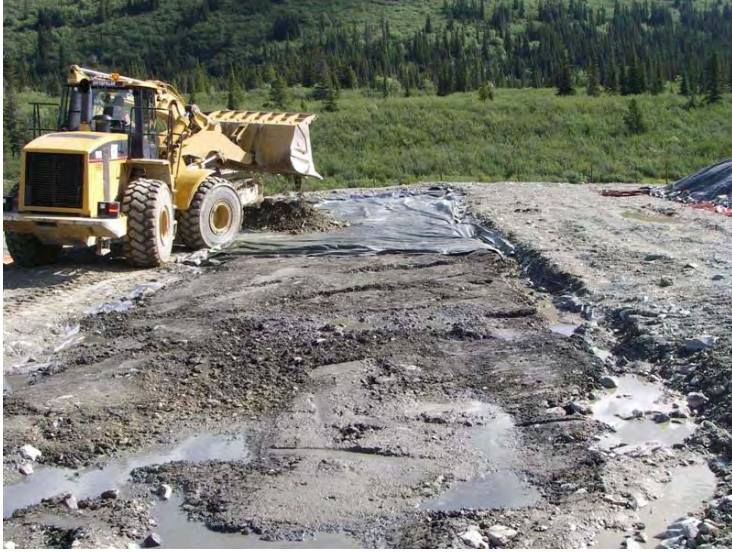
Photo 1 07/26/07 Placing clean soil over the flattened and tarped contaminated material; facing east
