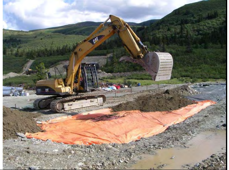
Photo 2 07/26/07 Placing clean soil over the flattened and tarped contaminated material; facing north
