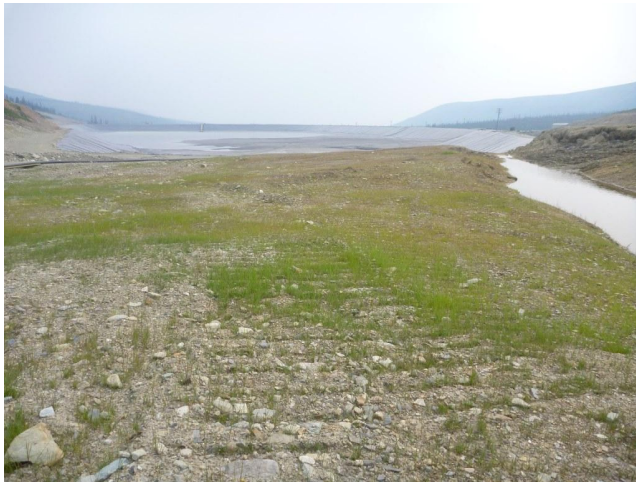
Photo 2-7: Looking South at Established Vegetation on Disturbed Ground Around the TSF Following Fall 2012 Seeding (July 2013)
