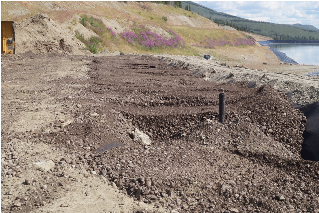
Photo 2-3: Bioreactor Filled with Substrate Material (July 16, 2016)
