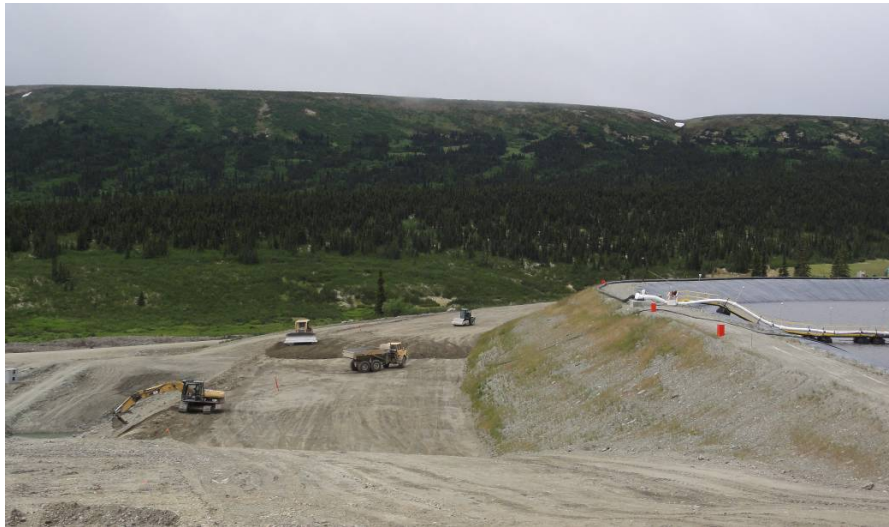
Photo 2-6: Construction of the Ultimate TSF dam; Note Seeding on the Starter Dam Face has Resulted in ~50% Grass Cover Between the Crest and Construction Zone (July 2012)
