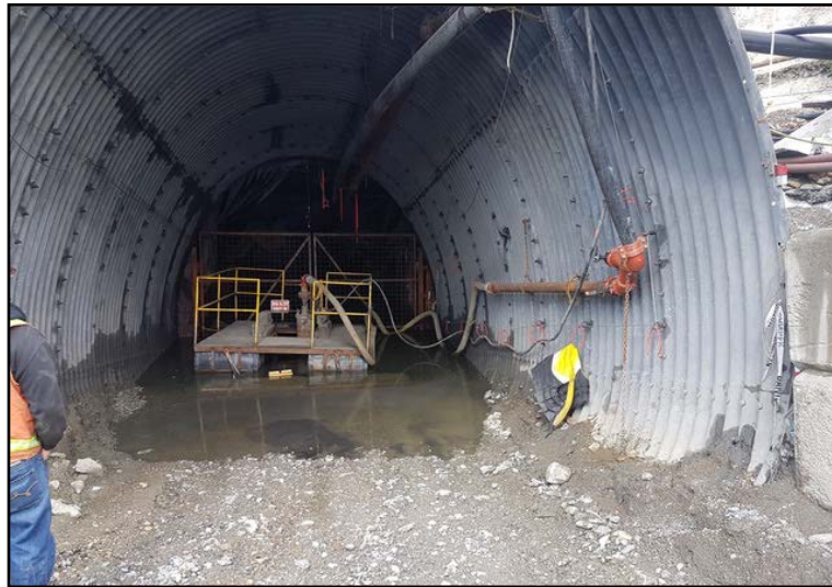
Photo 5-3: Wolverine Mine Adit Groundwater Pump System (July 13, 2017)
