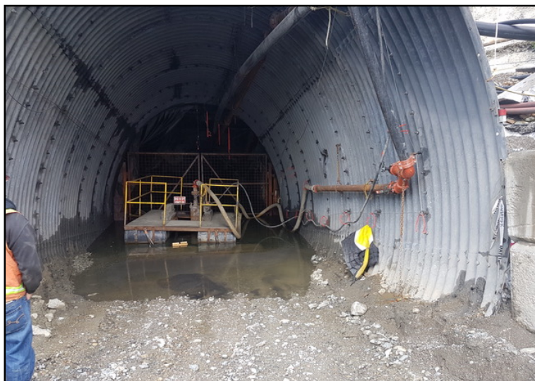
Photo 5-3: Wolverine Mine Adit Groundwater Pump System (July 13, 2017)
