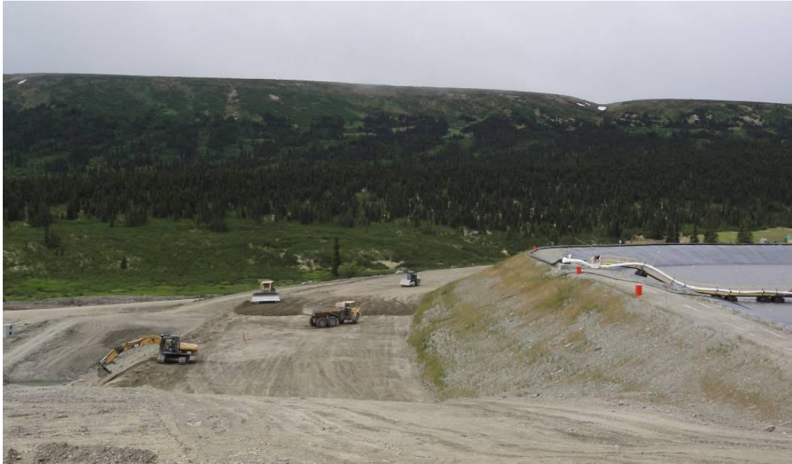
Picture 5-3: Construction of ultimate tailings dam; note seeding on the starter dam face has resulted in ~50% grass cover between the crest and construction zone (July 17, 2012)
