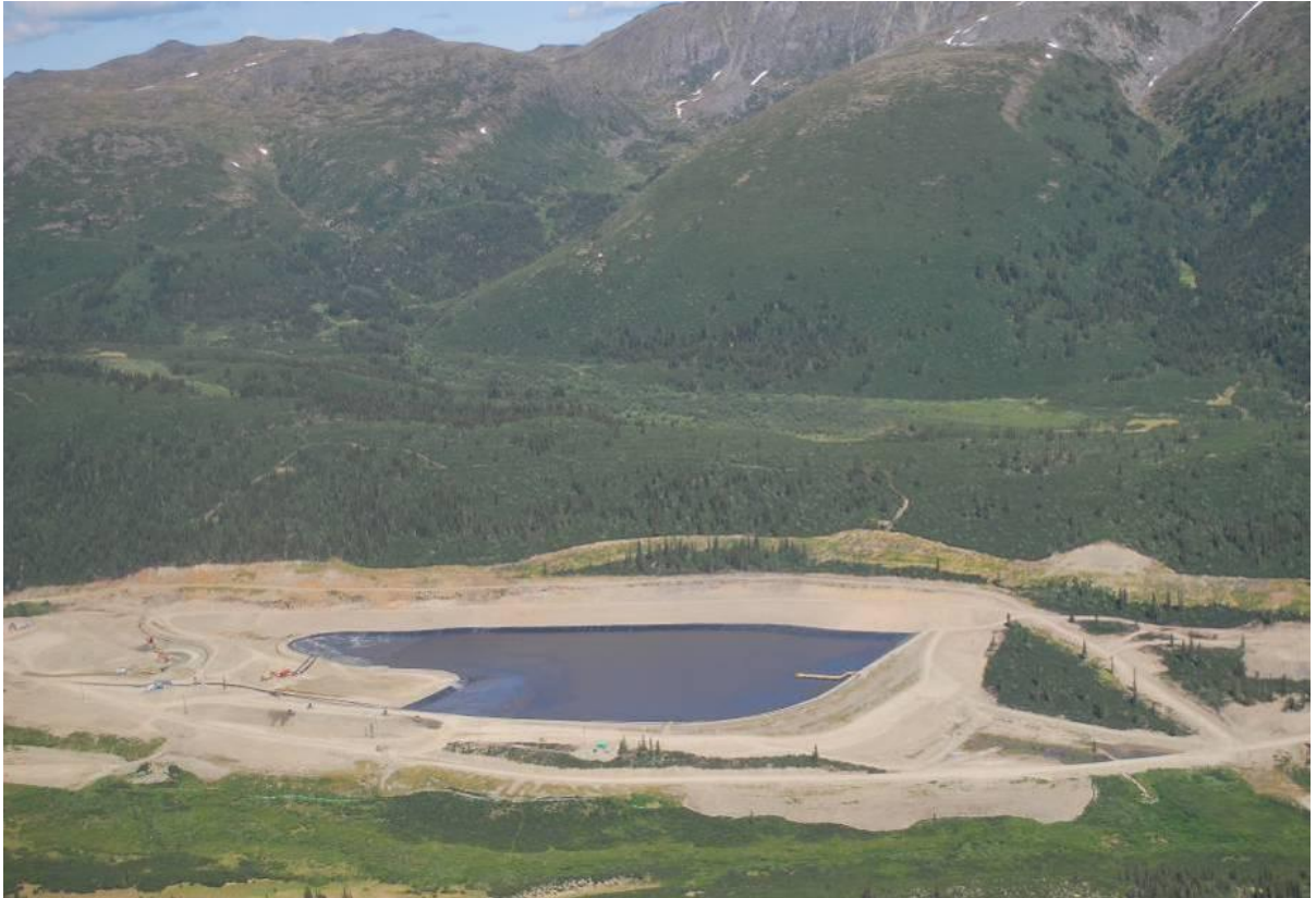
Picture 6-2: Tailings facility area during ultimate dam construction; lined area is starter impoundment (July 6, 2012)
