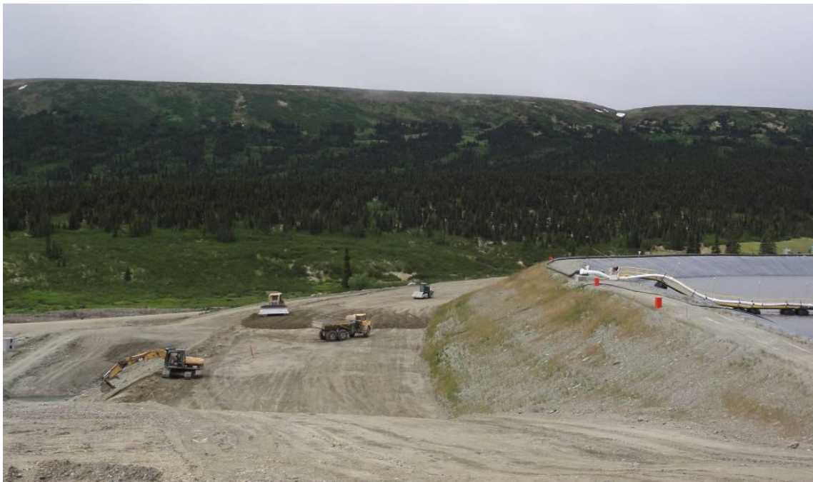
Picture 5-4: Construction of ultimate tailings dam; note seeding on the starter dam face has resulted in ~50% grass cover between the crest and construction zone (July 17, 2012)
