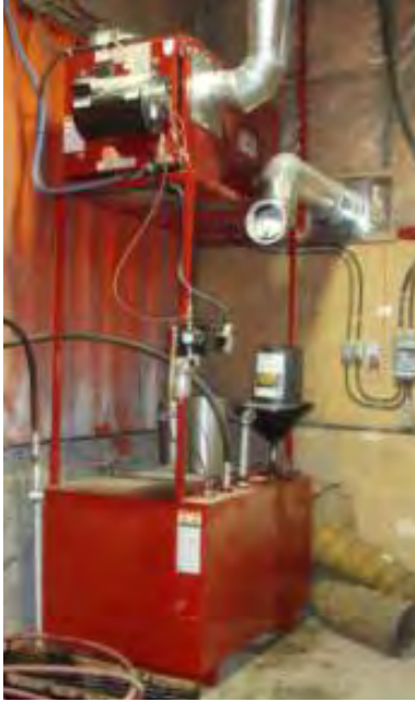
Picture 2-9: Waste Oil Burner in Procon Maintenance Shop
