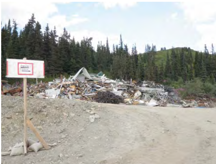
Picture 2-7: Sign showing direction of steel and wood piles with steel pile in background.
