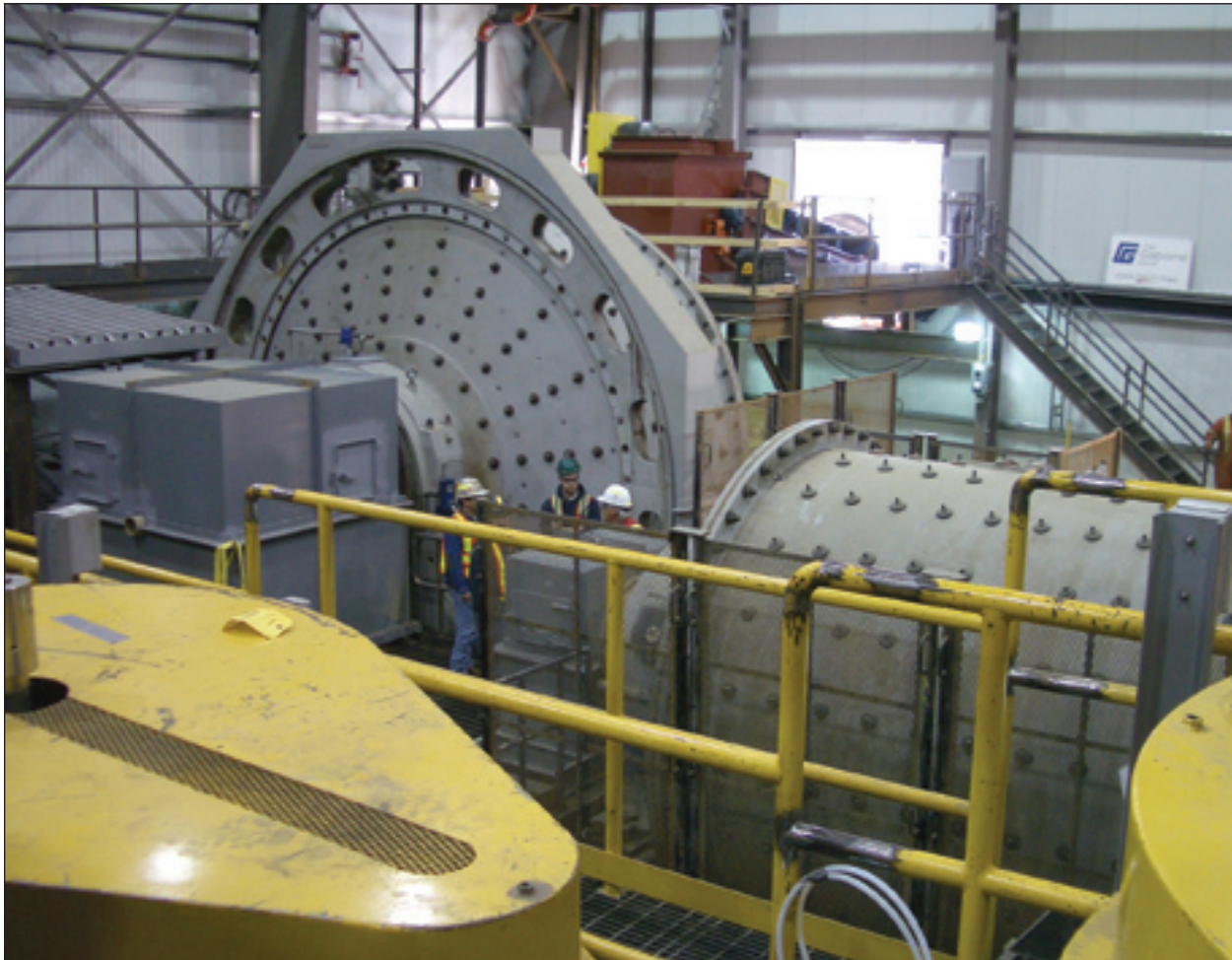
Sherwood Copper's Minto copper-gold mine.
