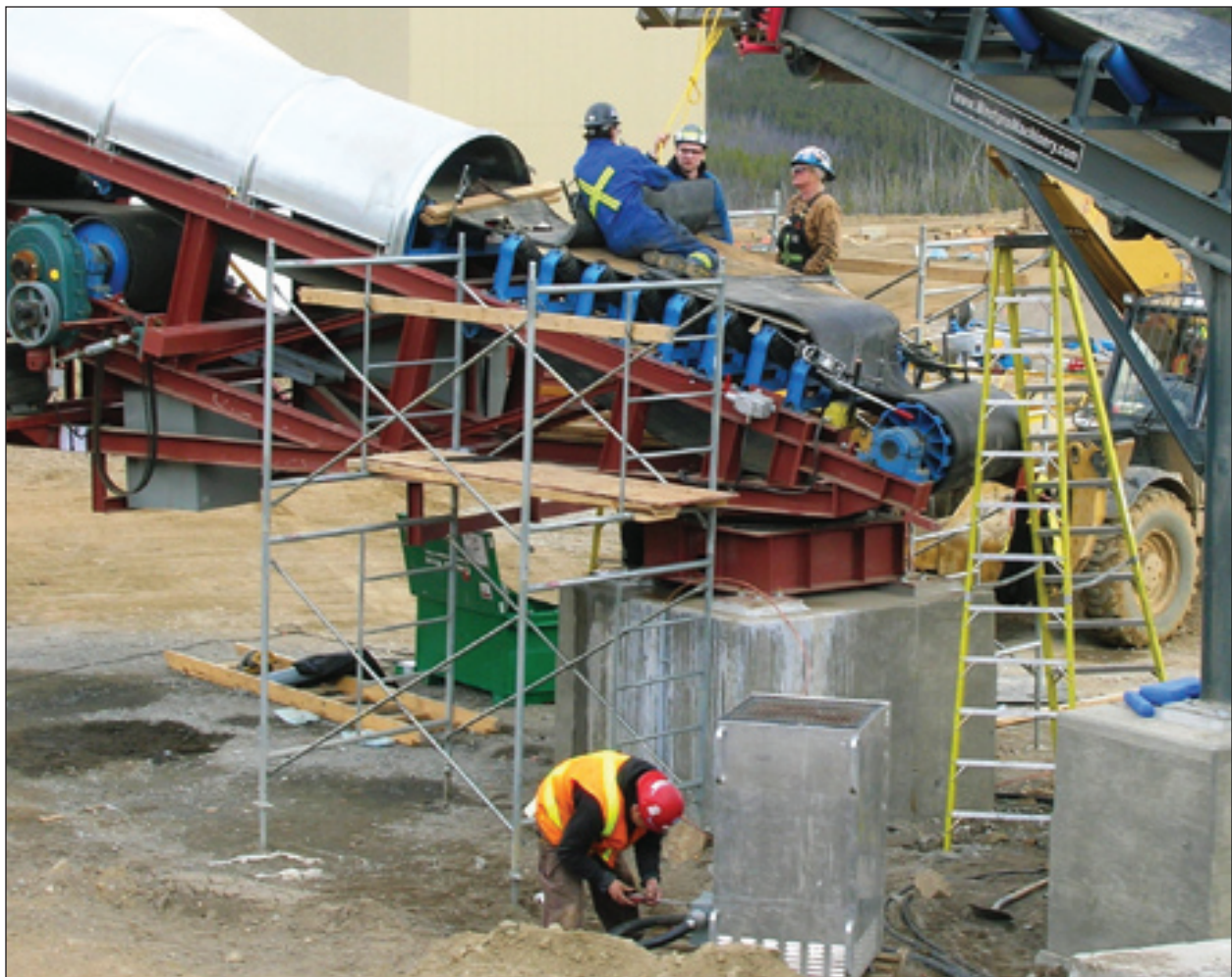
Sherwood Copper’s Minto copper-gold mine.
