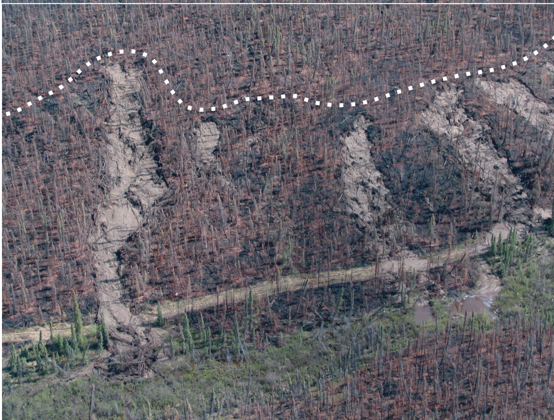
Figure 5.27: Failures SC26A, SC27A, SC28A and SC29A showing break of slope headscarp location (Dashed line indicates break of slope).
