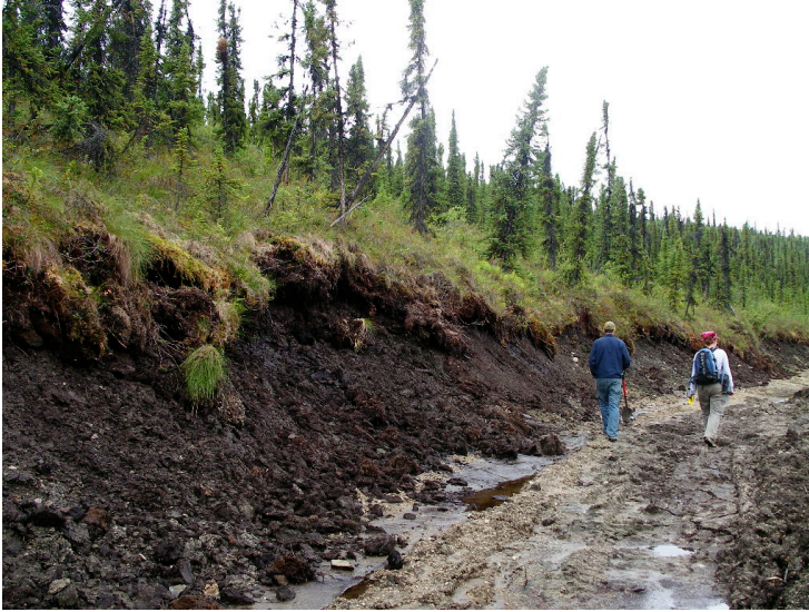
Figure 5.32. Lone Star Road Cut. Excavation approximately 5 m past people.
