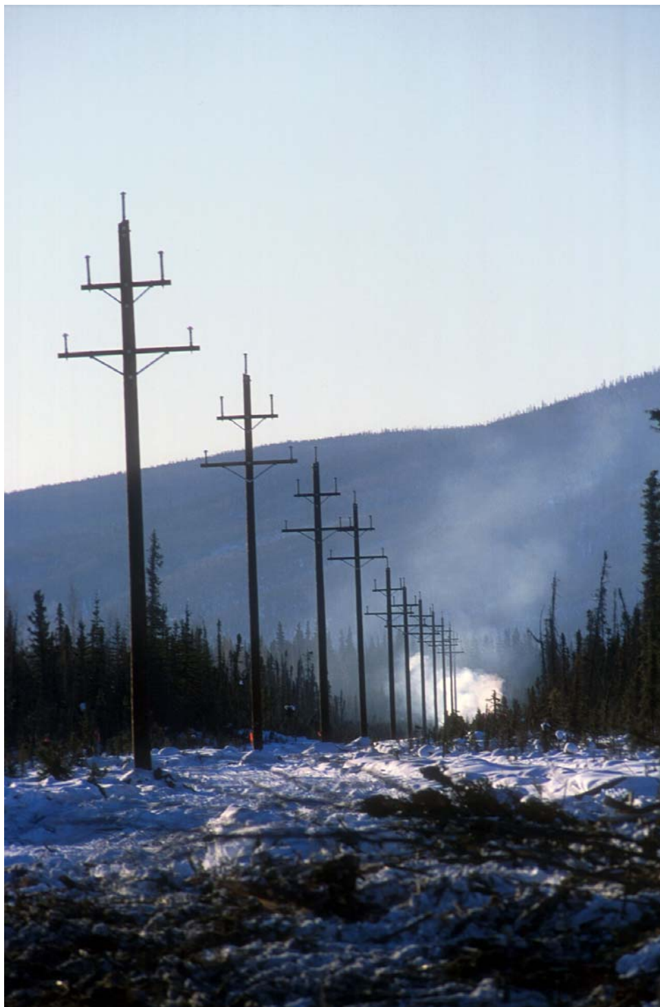
Figure 6-4 Example 69 kV Single Pole Structures
