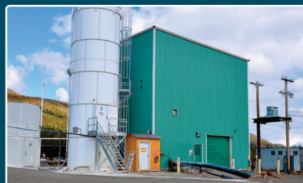
13. Vangorda Water Treatment Plant
