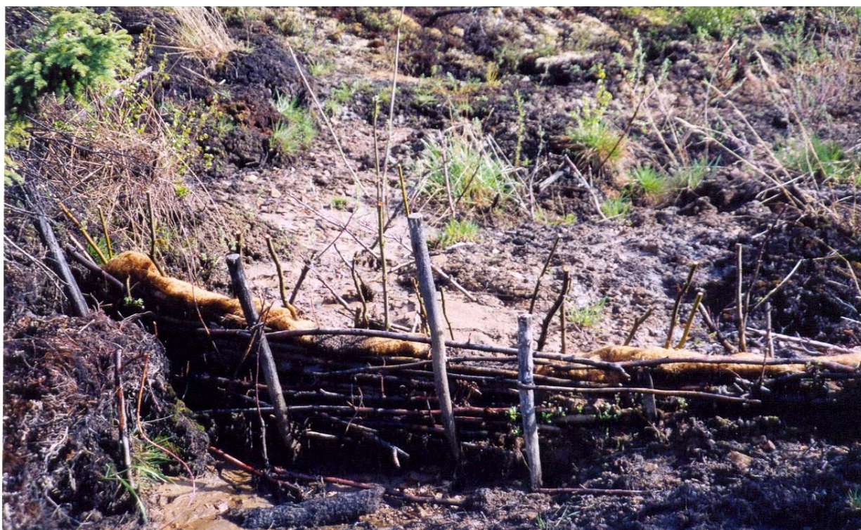
PLATE # 10: Downstream side of gully break #1, May 27, 2004.
