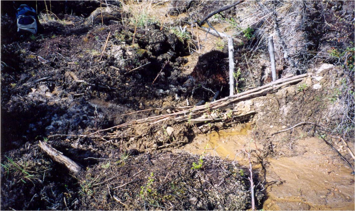
PLATE #11: Gully break #3 prior to repairs, May 27, 2004.
