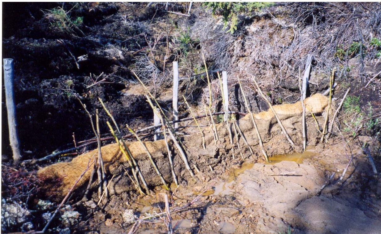
PLATE #9: Gully break #1 repaired in Sept '03 has not breached and has trapped sediment. Note mud layer on geotextile indicating where water level had been earlier in May 2004.
