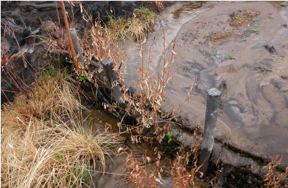
PLATE #20: Close up of gully break showing correct decanting of surface flow. Note new willow shoots on wattle fence.
