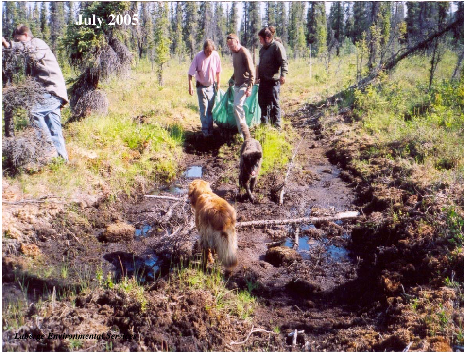
Photo #45: The peat and dead trees were used as fill to remediate the deep ruts, July 2005.
