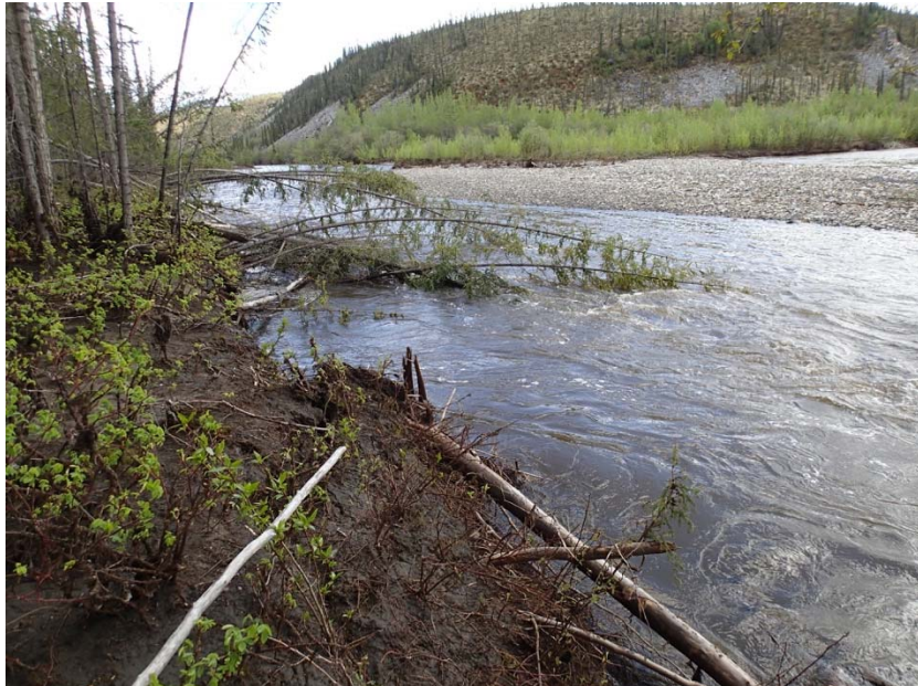
KM 195.1 (Photo 1). Fallen/leaning trees along the outer (northeast) bank of Engineer Creek
