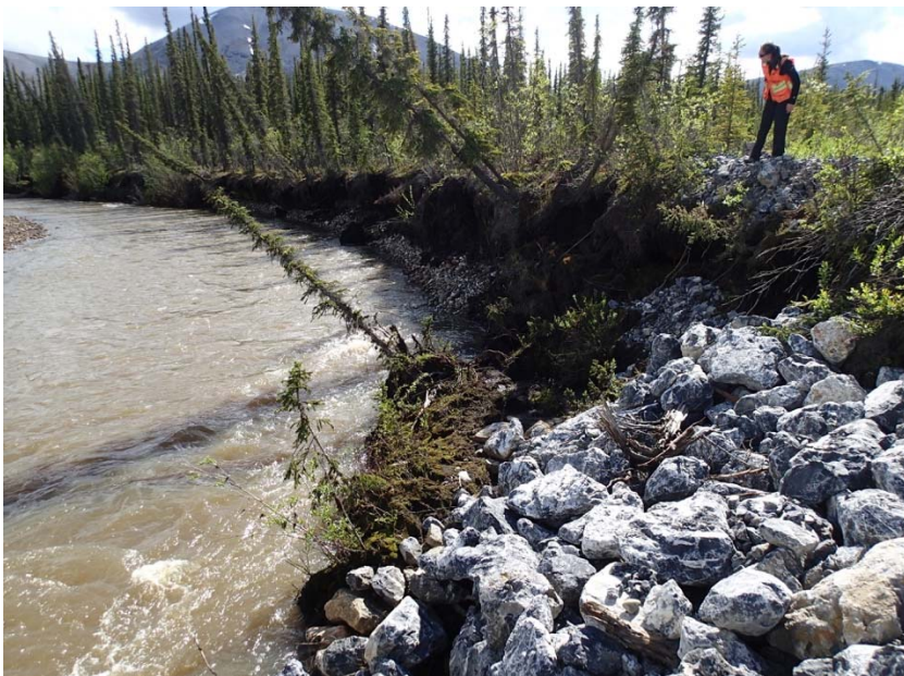
KM 182.1 (Photo 1). Active scour and permafrost degradation beneath previously placed riprap
