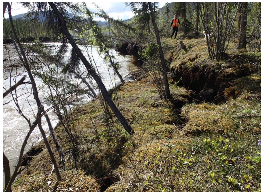
KM 182.1 (Photo 2). Significant bank collapse in permafrost downstream of previously placed riprap
