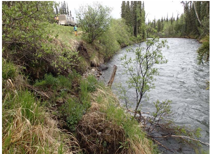
KM 54.9 (Photo 2). Bank slumping at downstream end of encroachment site
