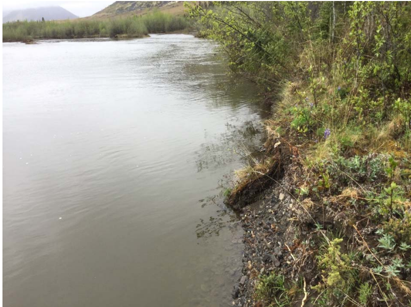
KM 138.5 (Photo 1). Leaning trees and exposed bank at the upstream end of the encroachment site
