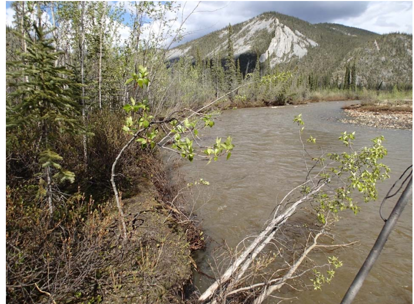
KM 183.3 (Photo 2). Leaning trees and bank scour
