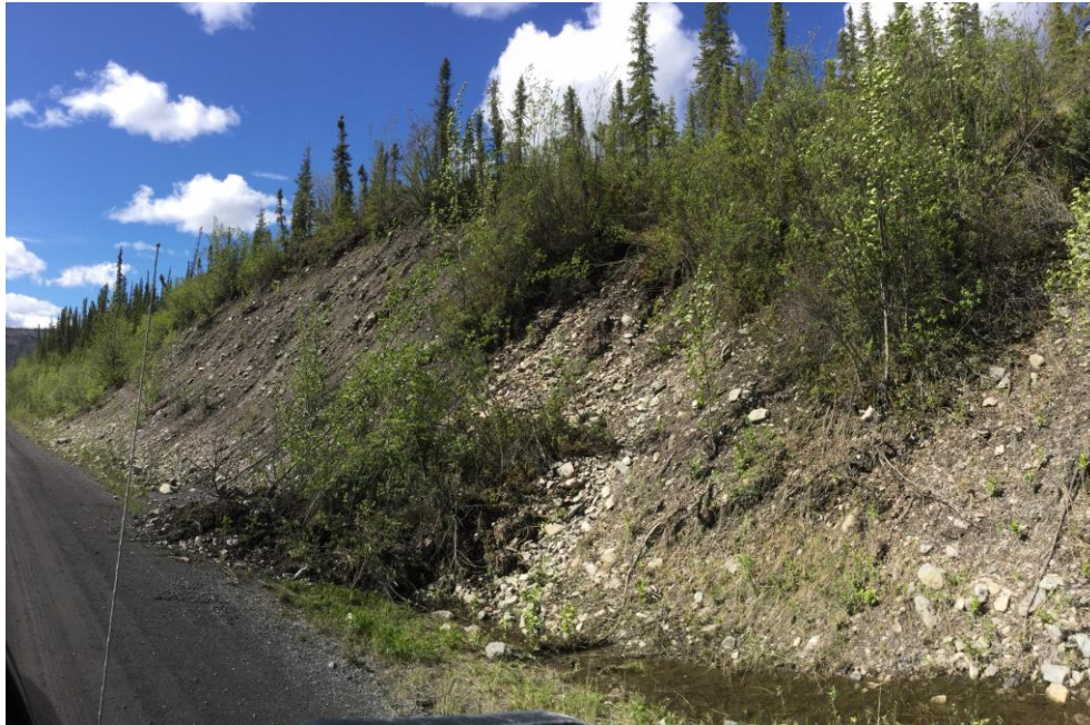
Figure 5-6. Example of a Road-cut Slough Excluded from the Geohazard Inventory
