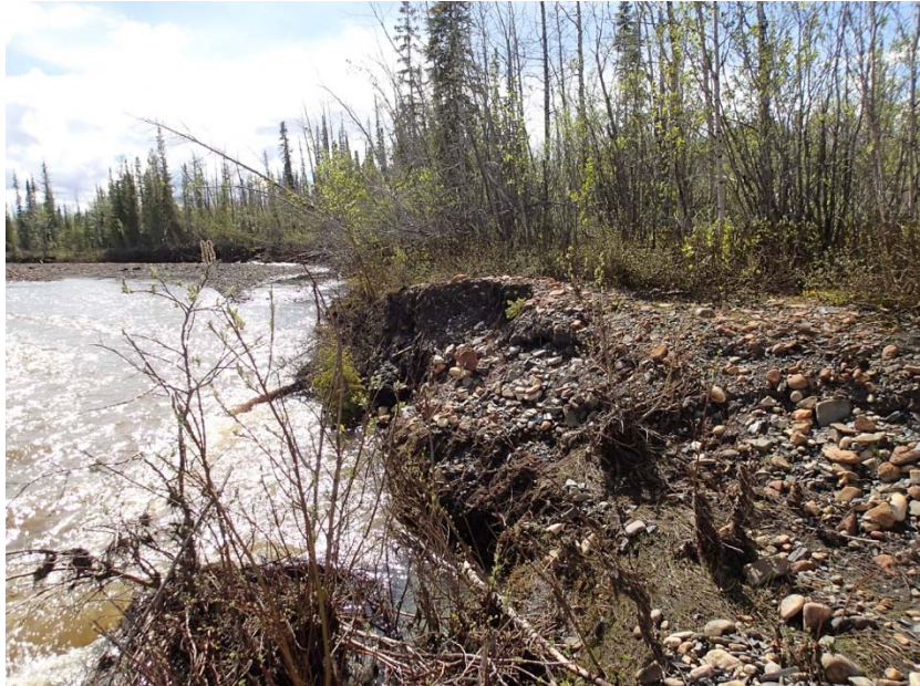
KM 170.9 (Photo 1). Active erosion at upstream end of encroachment site
