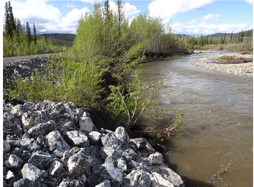
KM 188.6 (Photo 2). Leaning trees and bank scour downstream of recently placed riprap
