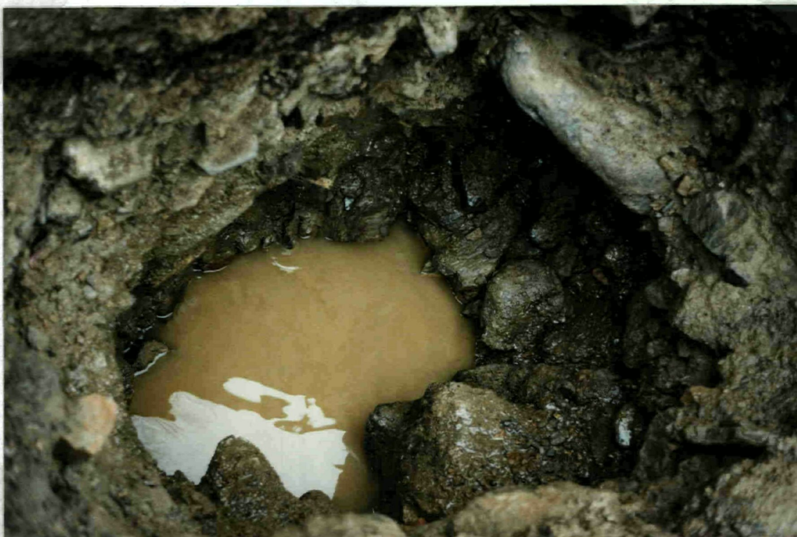
SITE WITH WATER POURING IN
