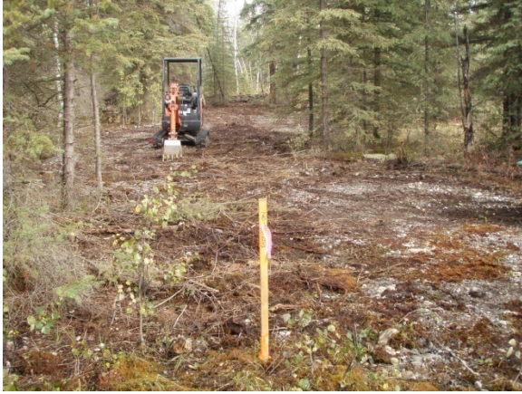
NC-TR-15-01, reclaimed, a small amount of vegetative mat was present due to the proximity of gravel in a well drained area, looking north
