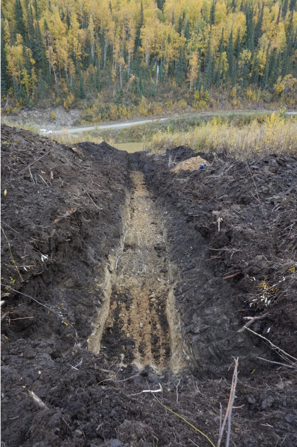
Figure 7. Completed trench looking downslope toward Canyon Creek. The far end of the trench bottoms on muck due to a drop in the bedrock surface.
