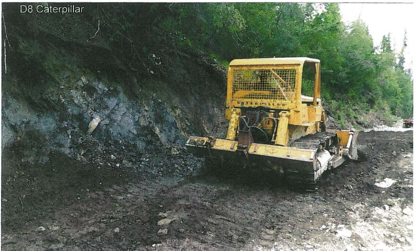
Photo 11: Left Limit Trench where bulldozer has exposed the bedrock- gravel contact. Note how high the bedrock is as it rises rapidly to the west marking the edge of any placer gold reserves
