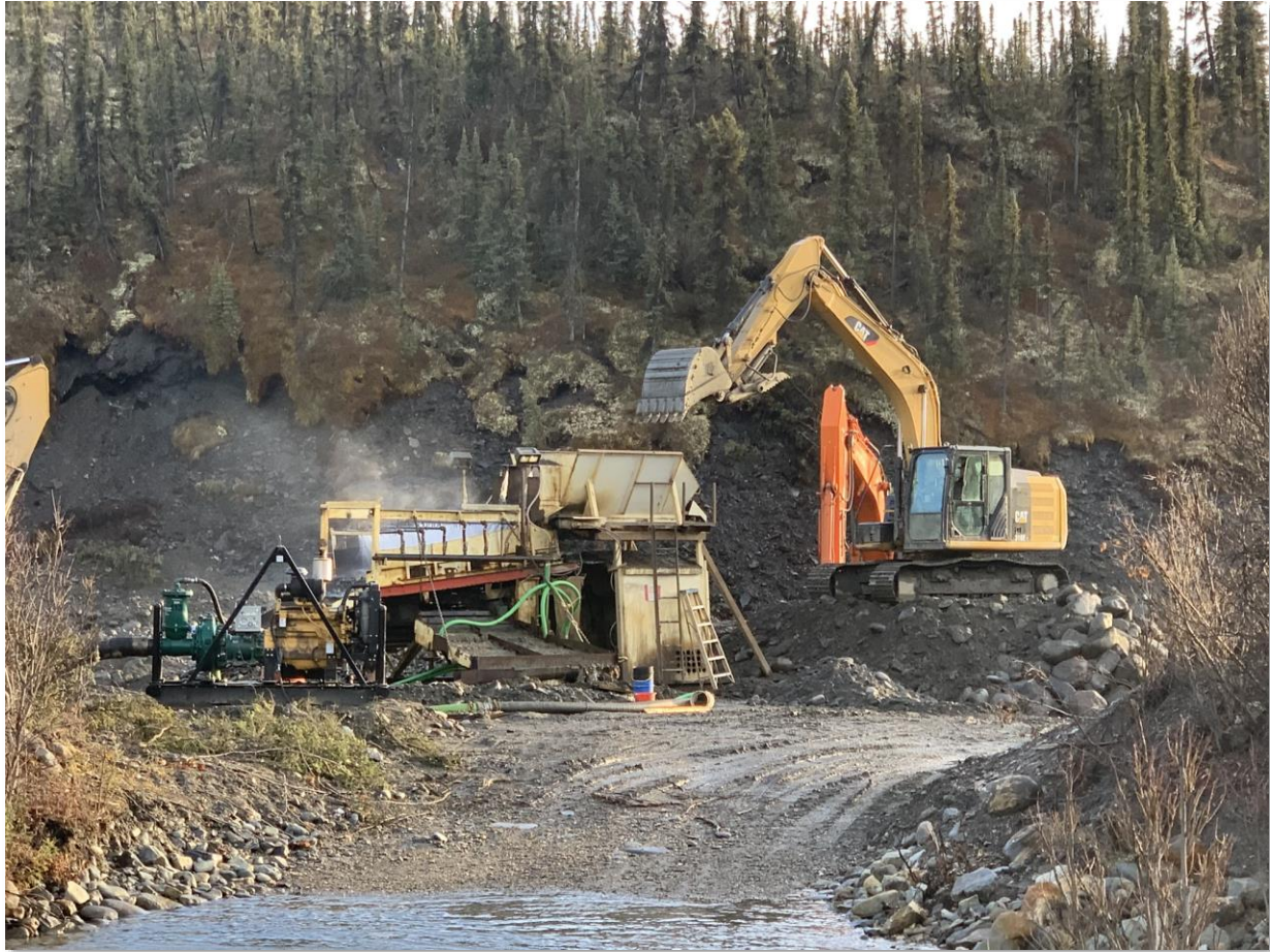
Figure 11 – Bulk sample 22-6 (1791 cubic yards) was processed from near-surface gravels near the confluence of Lightning and Upper Duncan Creeks, using an oscillating screen deck and sluice runs. The gravels were stockpiled near the sluice plant and fed with a CAT 316 excavator.
