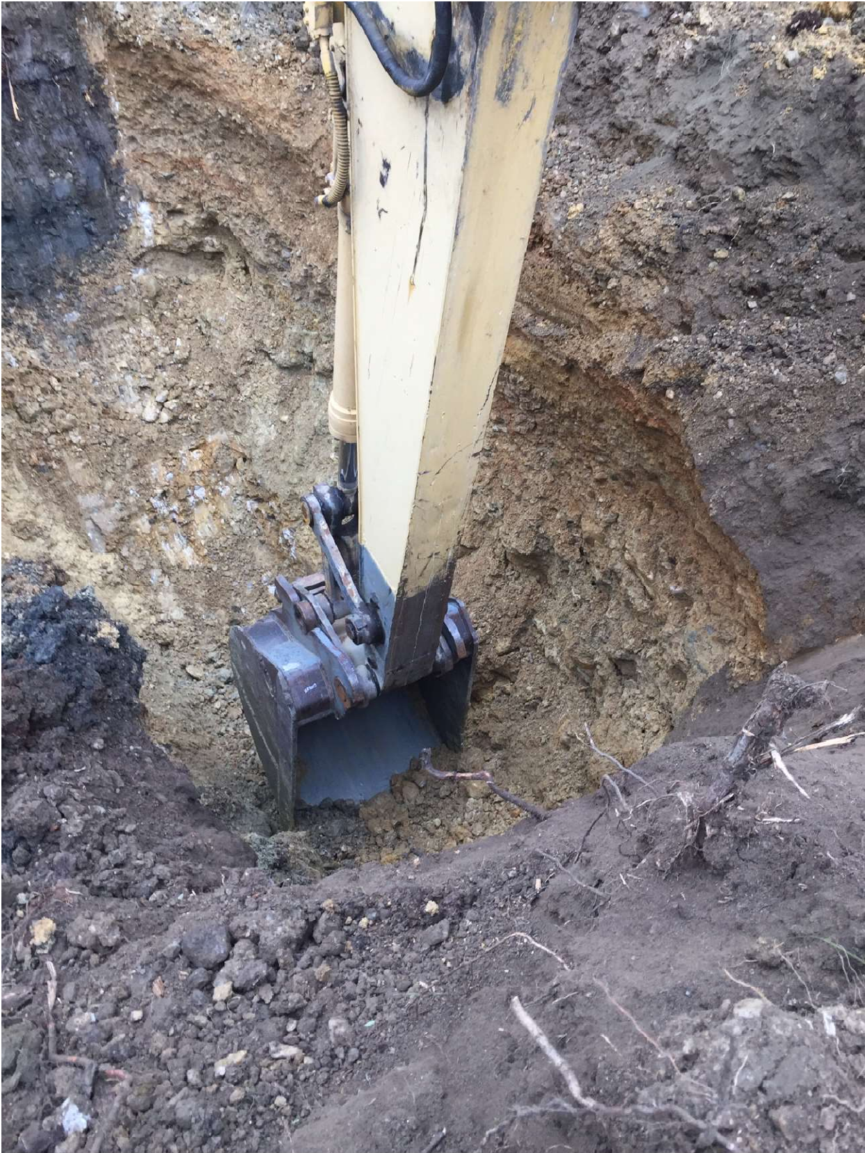
PHOTO #8 Excavating Deep pit upper unit (Colluvium?) Backfilled old 1992 trench top left
