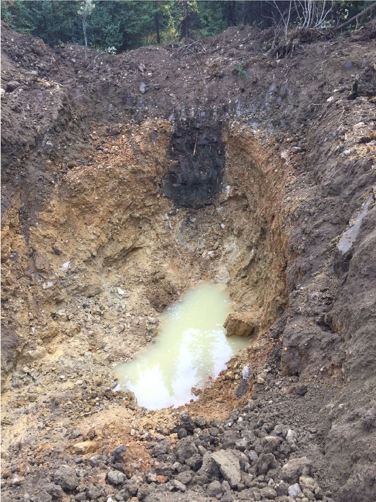
PHOTO #10 Completed Deep pit with groundwater ponding and slump from walls
