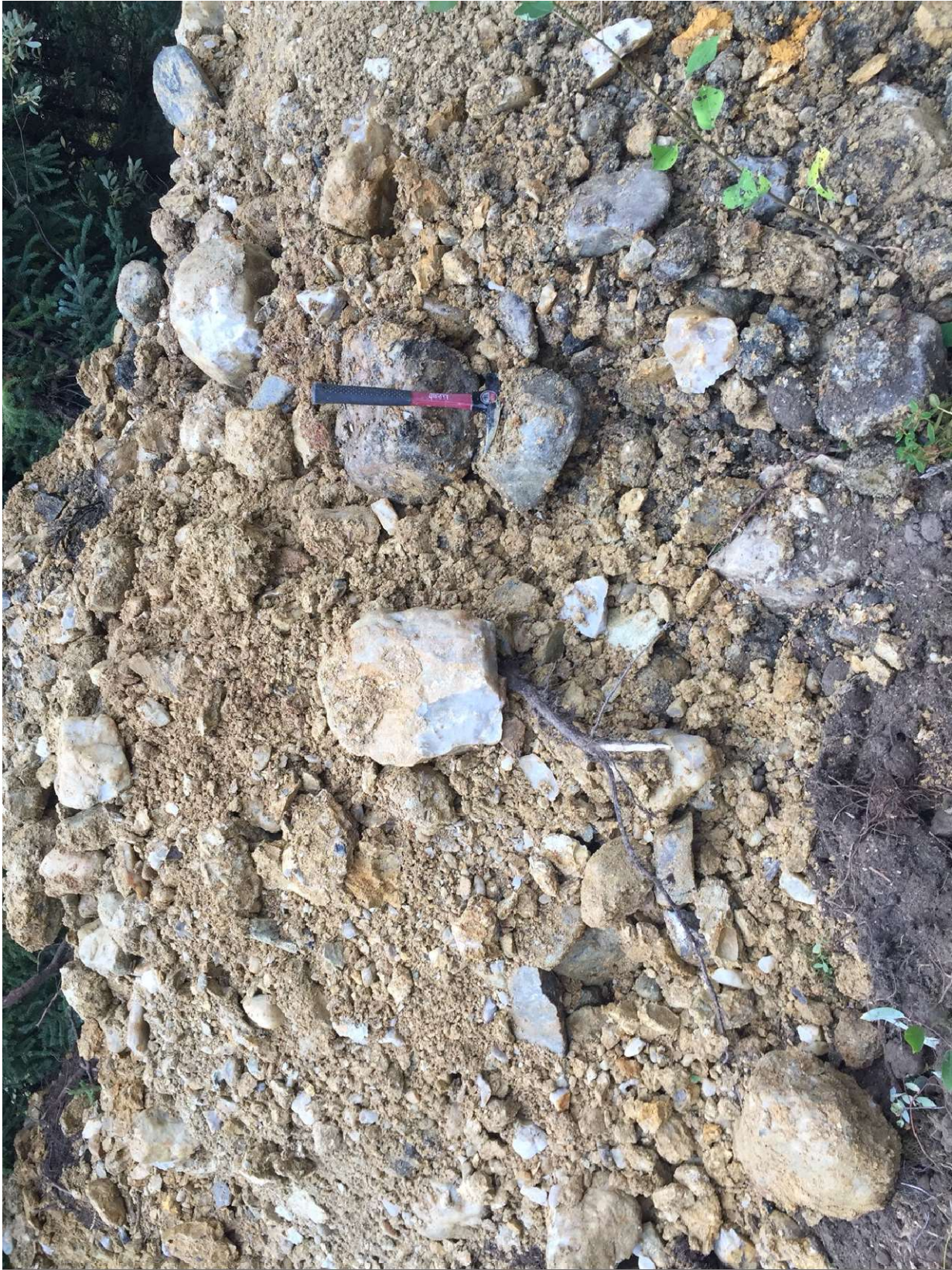
PHOTO #14 Deep pit excavated pile with boulders and cobbles from basal unit
