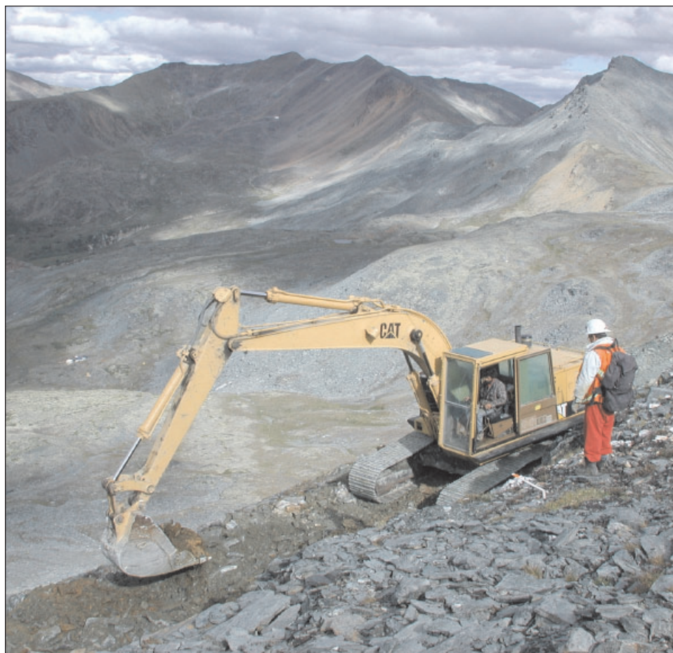
Figure 24. Bernie Gaboury of True North Gems directs excavator trenching on the Regal Ridge emerald property. Photo by Brad Wilson, True North Gems.
