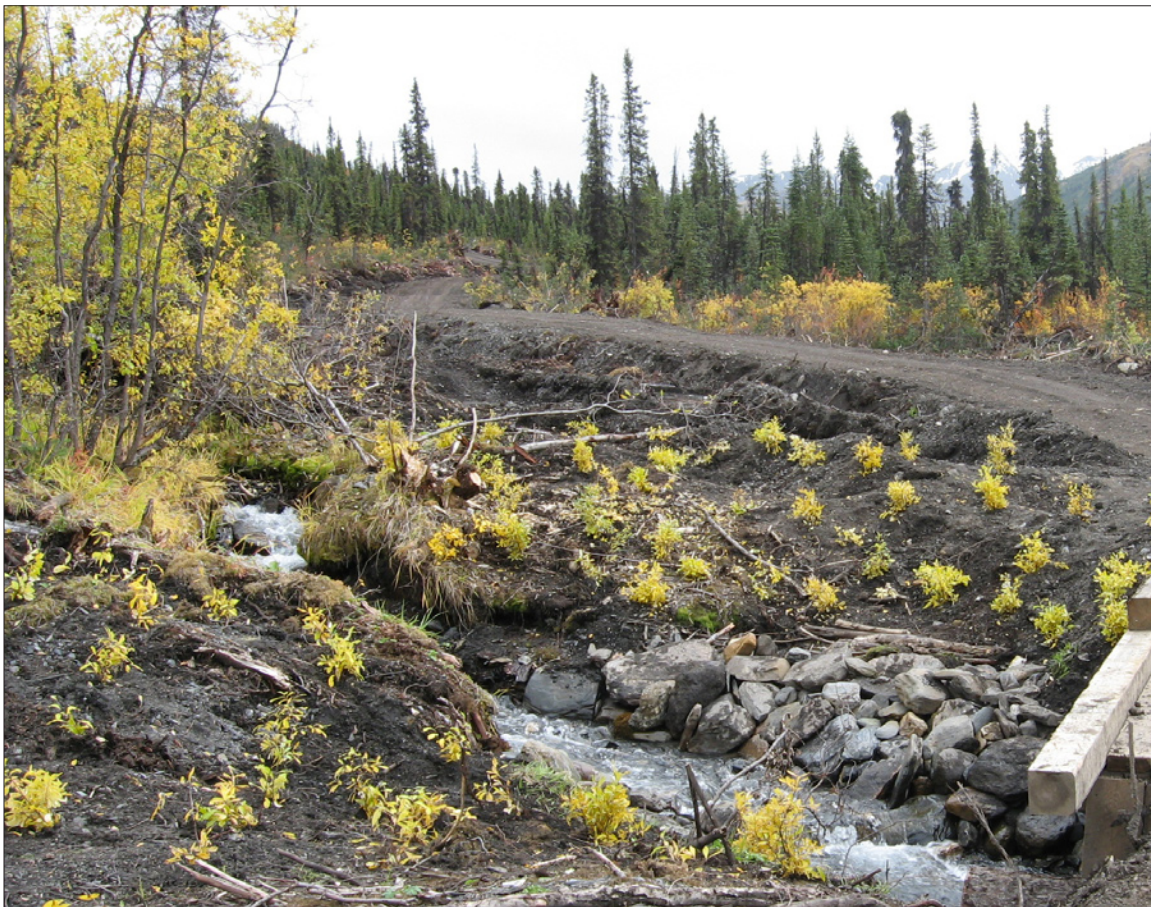
Figure 1. Bio-engineering in the Don Valley: live willows are being planted to stabilize the banks of the road.
