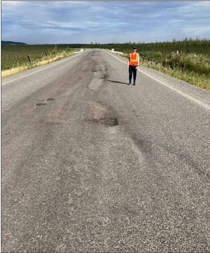
Figure 4. Site survey of Study Area B indicating a longitudinal depression in the central part of the highway (brown area), as well as potholes and other local depressions.
