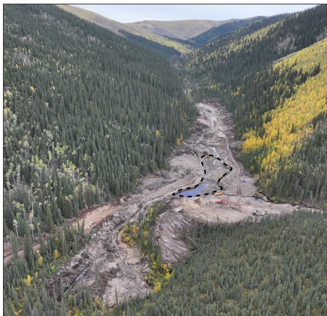
Figure 13. Aerial view of Waddington Charter and Contracting Ltd.'s active cut on Donahue Creek. The cut is outlined with a black dashed line. The view is looking upstream and to the east.
