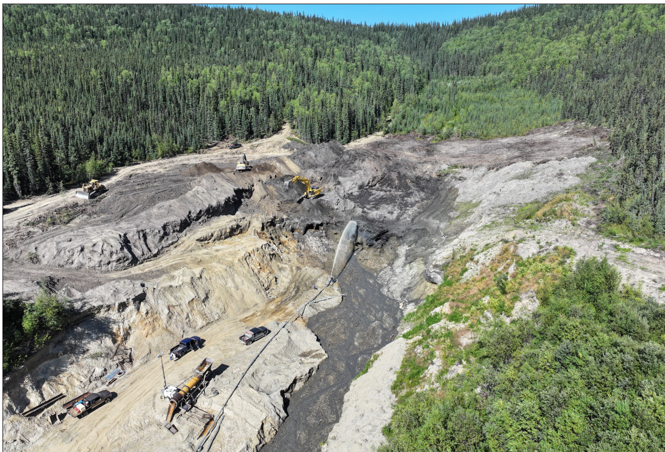
Figure 8. Monitoring at DK Gold Inc. and Lucky Dog Mining's joint operation on the left fork of Green Gulch.
