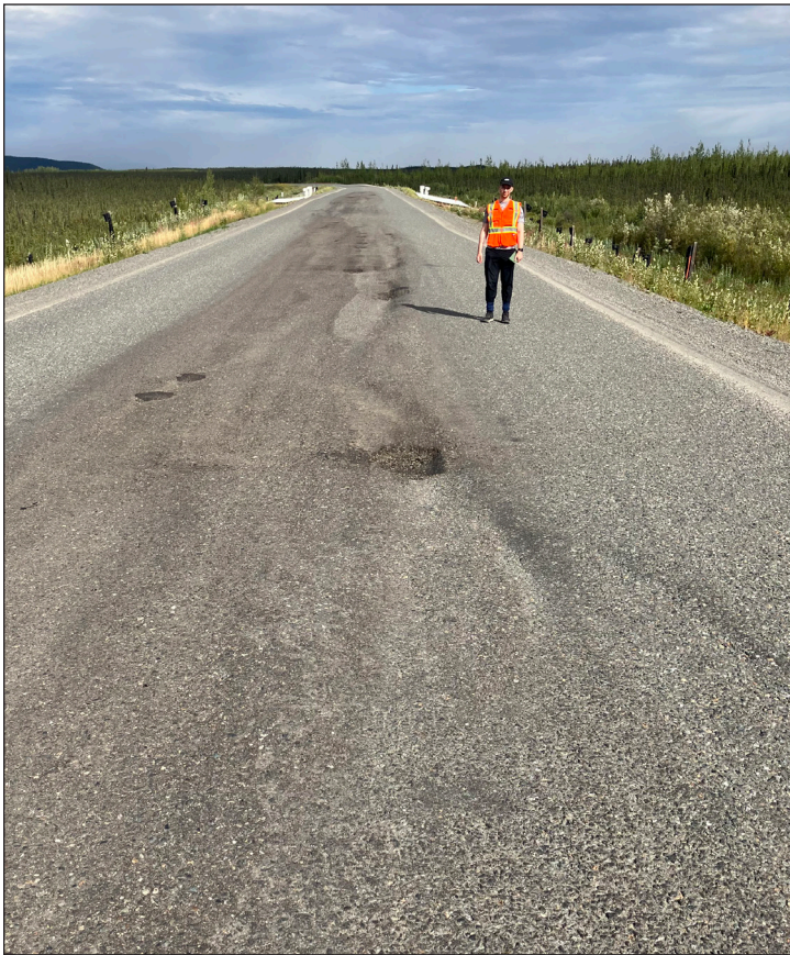
Figure 4. Site survey of Study Area B indicating a longitudinal depression in the central part of the highway (brown area), as well as potholes and other local depressions.
