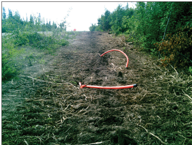
Figure 11. An example of the installed fibre optic line in 2022 at KM 311.6 of the Dempster Highway. The photo was taken 100 m from the embankment failure, and the removal of vegetation is evident.
