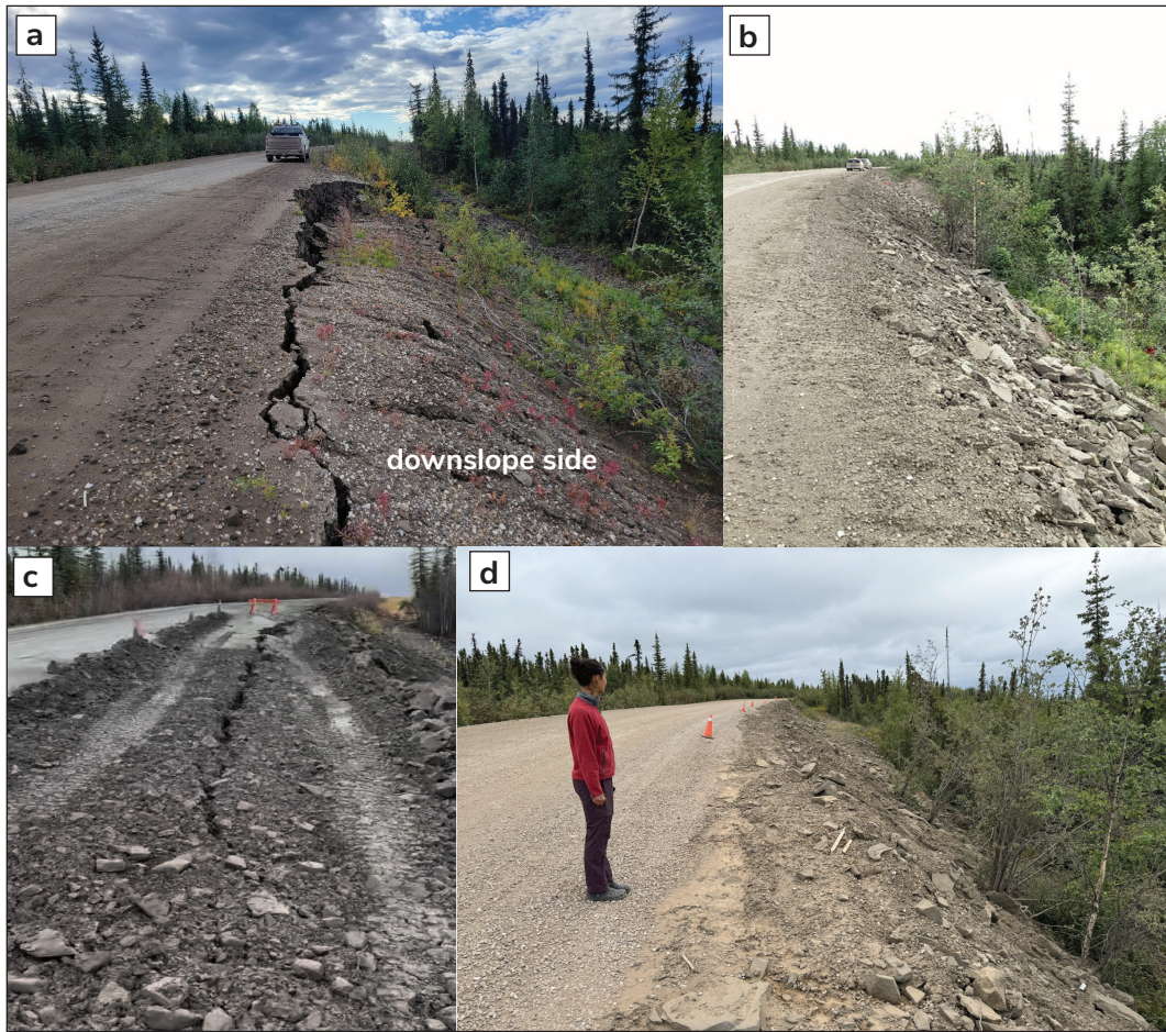
Figure 10. The evolution of the embankment failure at KM 312 of the Dempster Highway: (a) the initial failure in August 22, 2023; (b) the repaired embankment in July 22, 2024 and minimal cracking; (c) the failed embankment in October 2024; and (d) the stabilized embankment in July 2025. Photo by Stephan Gruber.
