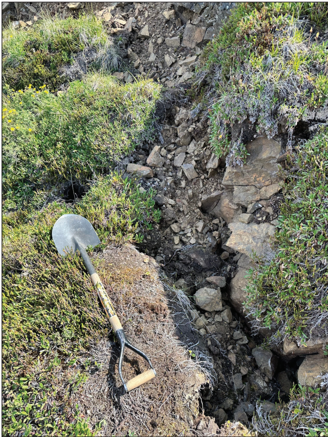
Figure 4. Large tension crack observed just below Miles Ridge. Note the fresh-appearing nature of the debris and the angular rock fragments. Shovel for scale is 100 cm long x 20 cm wide (blade).
