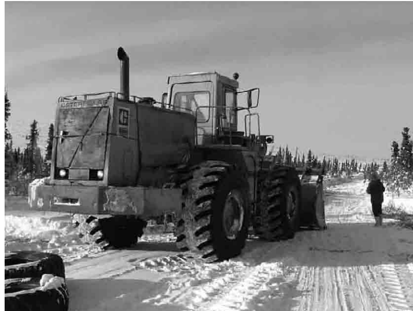
▲ Winter access road construction. Construction of new access roads is an important regional issue (photo: S. Francis)
