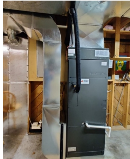
Figure 1: Mitsubishi Zuba (42,000 BTU/hr) indoor unit with single side return installed
