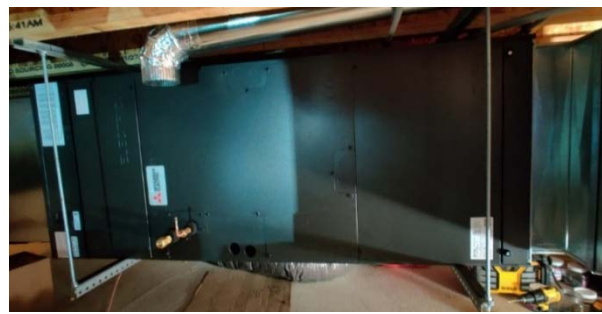
Figure 2: Mitsubishi Zuba (36,000 BTU/hr) indoor unit installed horizontally in a crawlspace.
