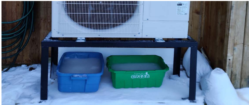
Figure 3: Mitigation measures taken to manage the defrost water coming off the Mitsubishi Zuba (42,000 BTU/hr) outdoor unit included putting bins and sandbags under and around the unit.
