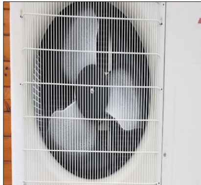
Figure 4: Accumulated frost on blades of Mitsubishi outdoor unit (42,000 BTU/hr).
