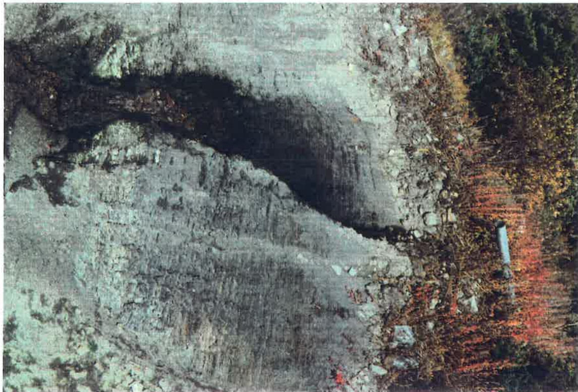
Photo B: Discharge pipe to pit - showing bank erosion
