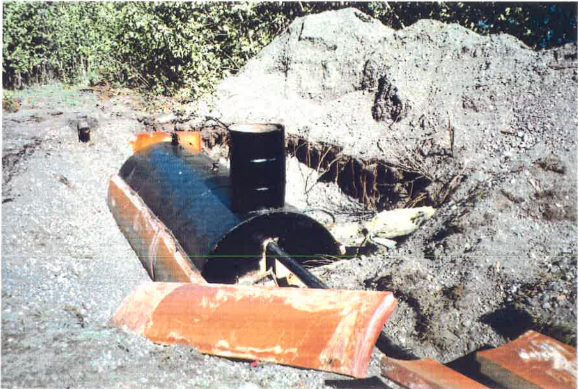
Photo A: Burwash Resort Holding Tank
