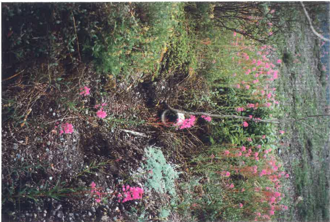
Photo B: Destruction Bay Sewage Lagoon - Old Discharge
