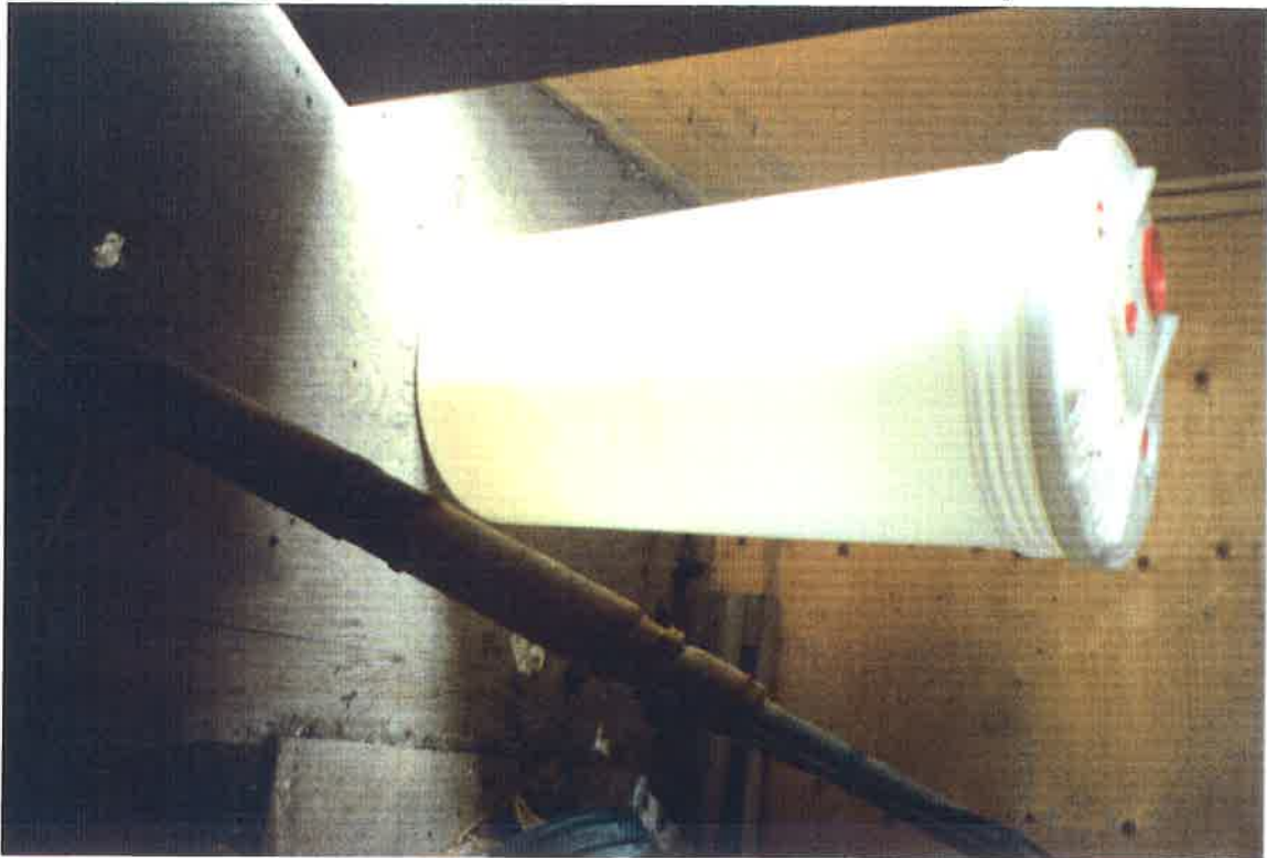
Photo L: Burwash Landing - Tank from Chlorination System
