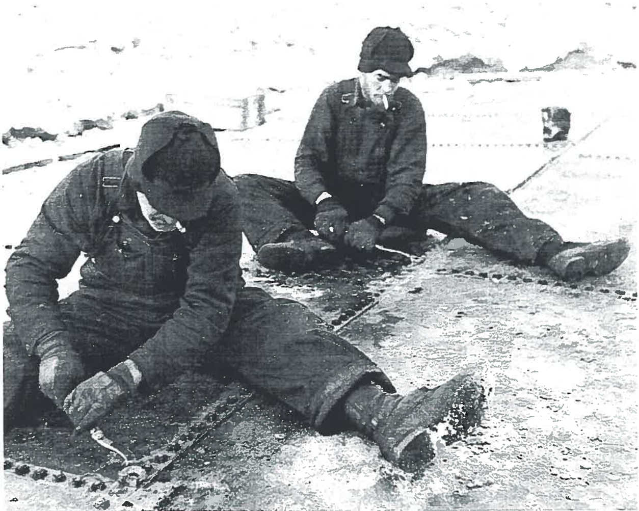
Figure 1. "J. P. Lanius and B. S. Field tightening bolts on the floor of tank #10." YA. Finnie Coll.. PHO 142. 675.
