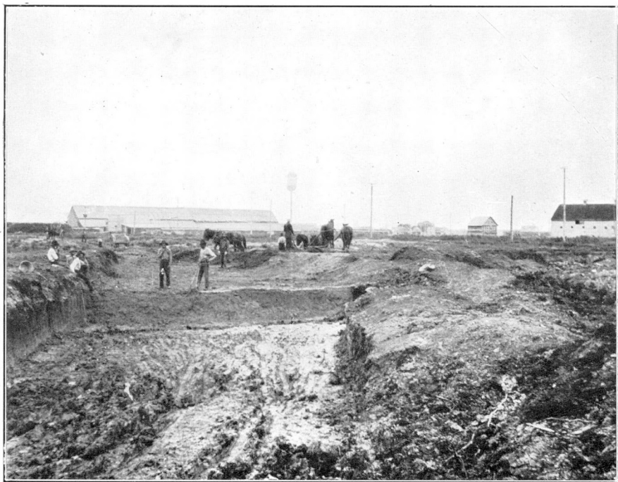
Pit in surface clay at Alsip's brick plant, Winnipeg, Man. The pit has been excavated in the calcareous surface clay and the bottom of the excavation represents the top of the underlay.
