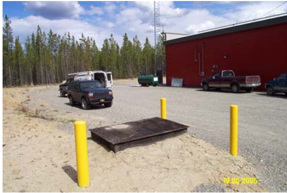
Photo 0188: 1391 Well Head Enclosure (front), Hootalinqua Firehall and Above Ground Fuel Storage Tank (back)
