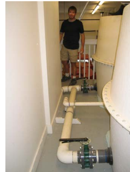
Photo 0013: 1391 Water Storage Tanks
