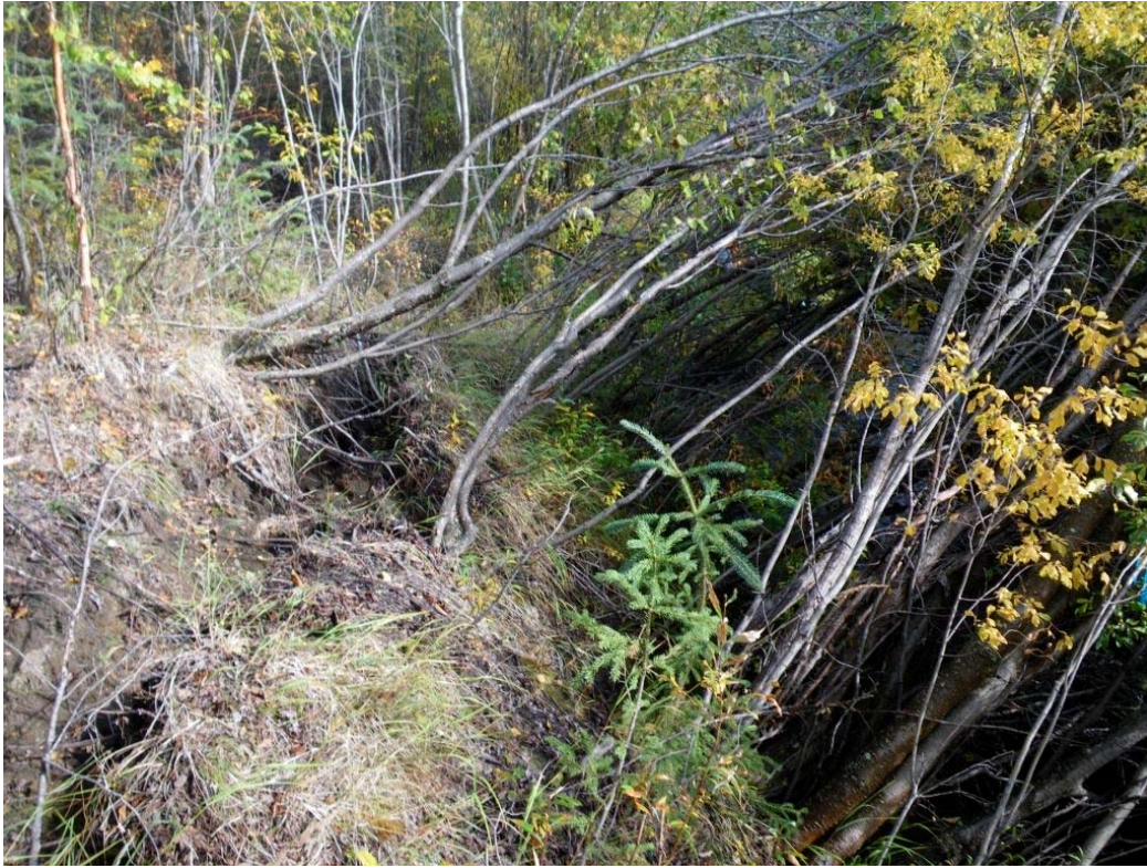
Photo #5: Slumping bank at B-8, looking upstream, September 1, 2009.
