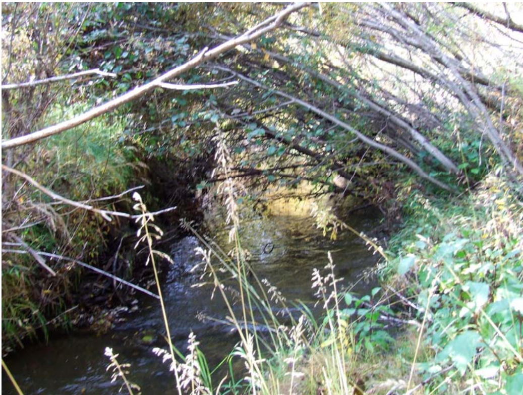
Photo #6: Slumping bank at B-8, looking downstream, September 1, 2009.
